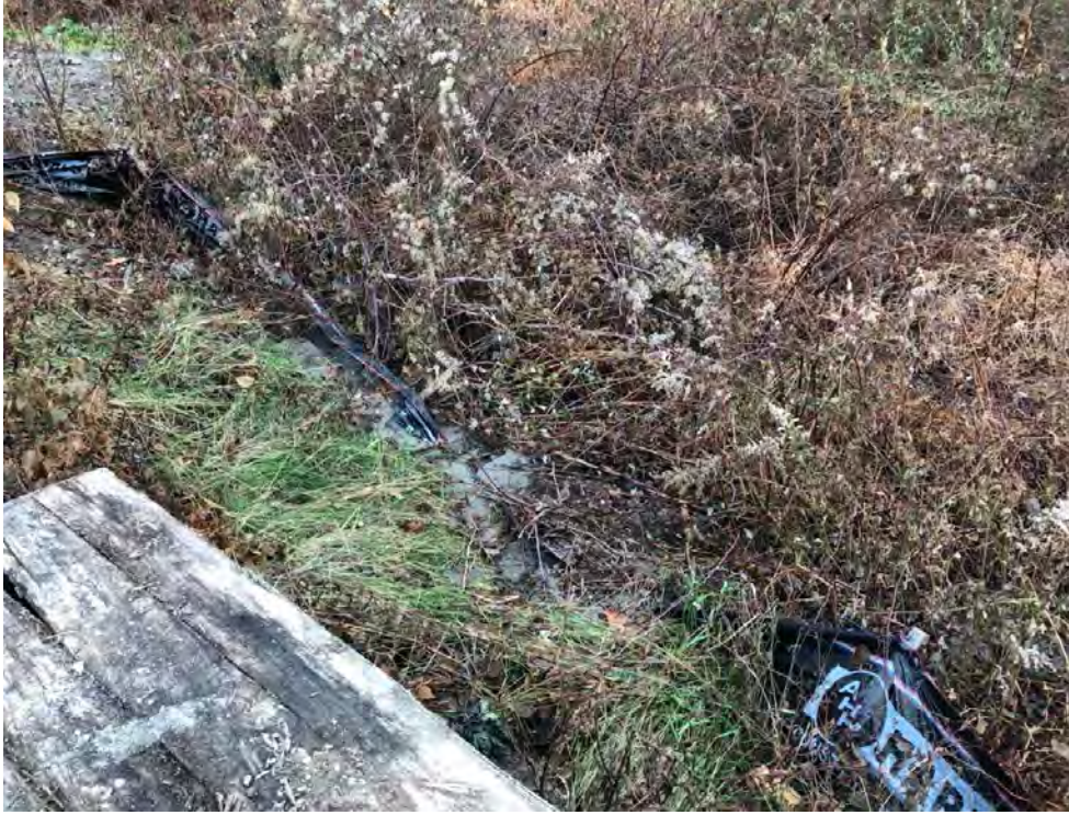
Photo 8: 11/17/2017, Watertown: Map 09, Str23, damaged silt fence.
