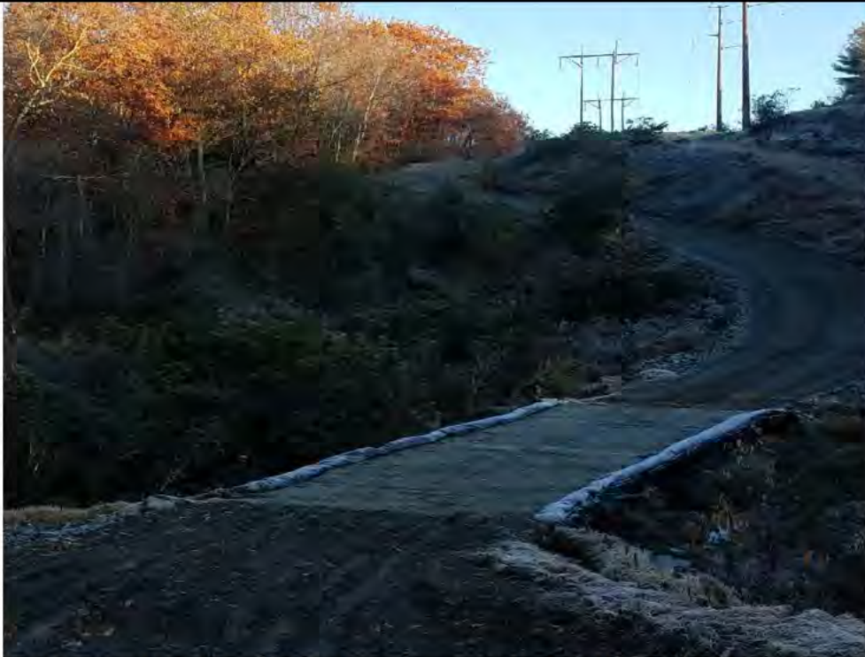
Photo 3:11/09/17, Watertown: Map 14, timber mat crossing conditions at W-C20, buildup of sediments on timber mats due to upland access road area conditions.
