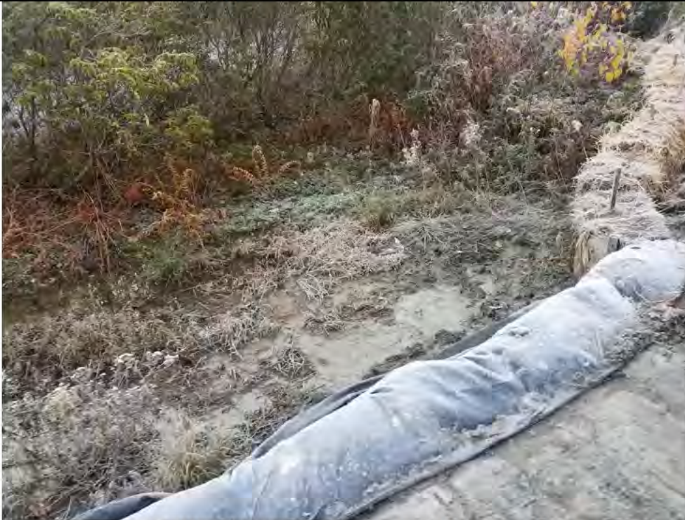
Photo 6: 11/09/17, Watertown: Map 14, W-C20 sedimentation through E&S controls and excess sediment buildup on timber mat crossing due to poor upland access road conditions.
