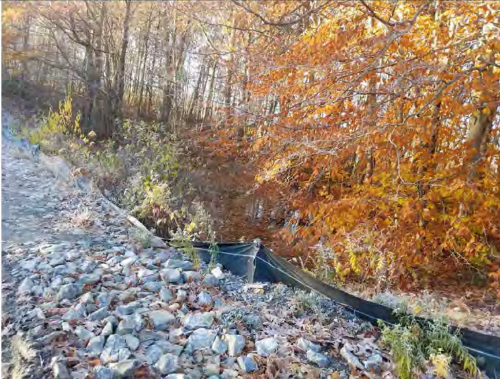
Photo 5: 11/09/17, Watertown: Map 11, west of Str31, non-compliant silt fence conditions, road base material height and pressing against silt fence, broken stakes, pictures through silt fence material due to road base gravel.
