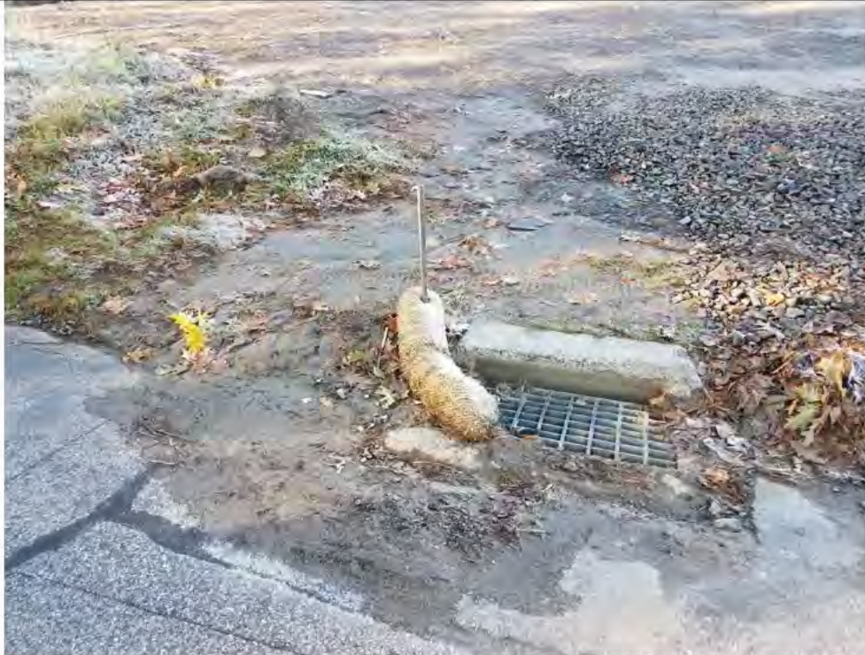
Photo 7: 11/09/17, Litchfield: Map 29, catch basin at Str81 west side of Campville Road, sediment movement from surface water runoff impacting catch basin and public access roadway.
