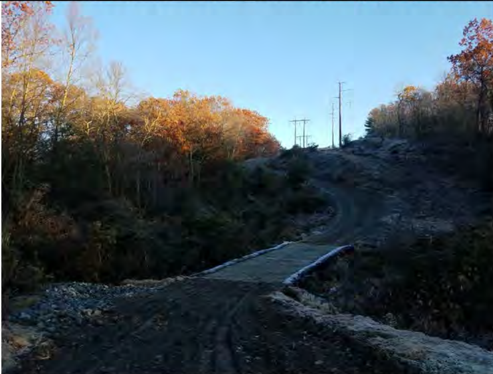
Photo 2: 11/09/17, Watertown: Map 14, access road conditions at W-C20, flattened water bar, visible tire rutting, poor access road grading at the sediment trap.
