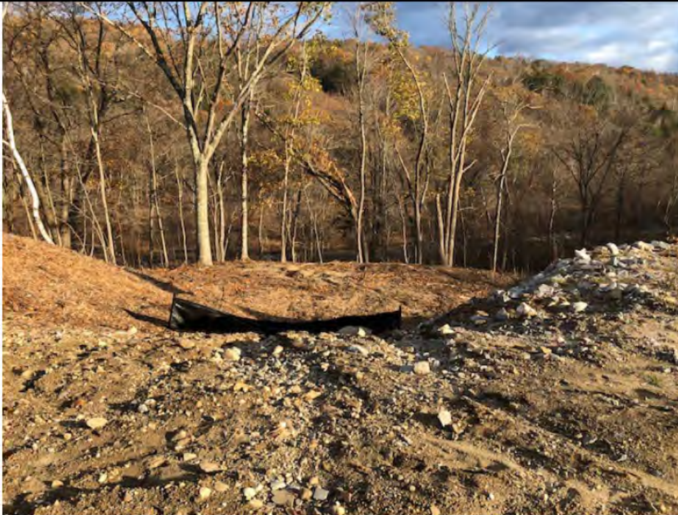
Photo 12: 11/17/2017, Watertown: Map 01, down gradient of Str1A, rill erosion and sedimentation down gradient to the east toward the Connecticut Wetland Only designated area, CORRECTIVE ACTION -E&S (silt fence) installed.
