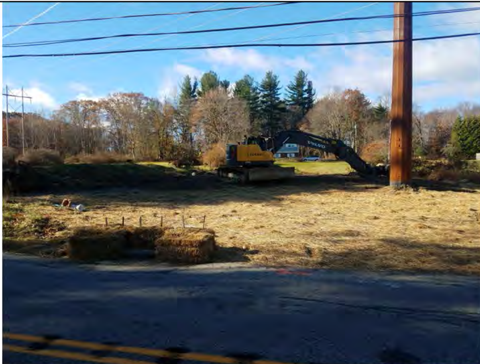
Photo 13: 11/17/2017, Litchfield: Map 29, Str81 and catch basin on Campville Road, CORRECTIVE ACTION - Installed E&S controls to protect catch basin, sediments were removed from the catch basin, straw placed over work pad to aid in controlling surface water runoff, restoration of the work pad has begun.
