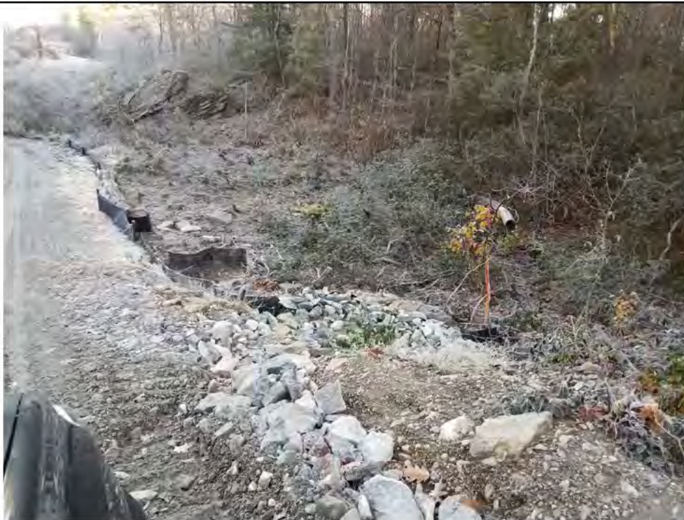
Photo 4:11/09/17, Watertown: Map 12, south of Str34, non-compliant silt fence conditions, sedimentation through E&S controls, road base materials exceeding height limits (structural) of silt fence, punctures through silt fence material due to road base gravel.
