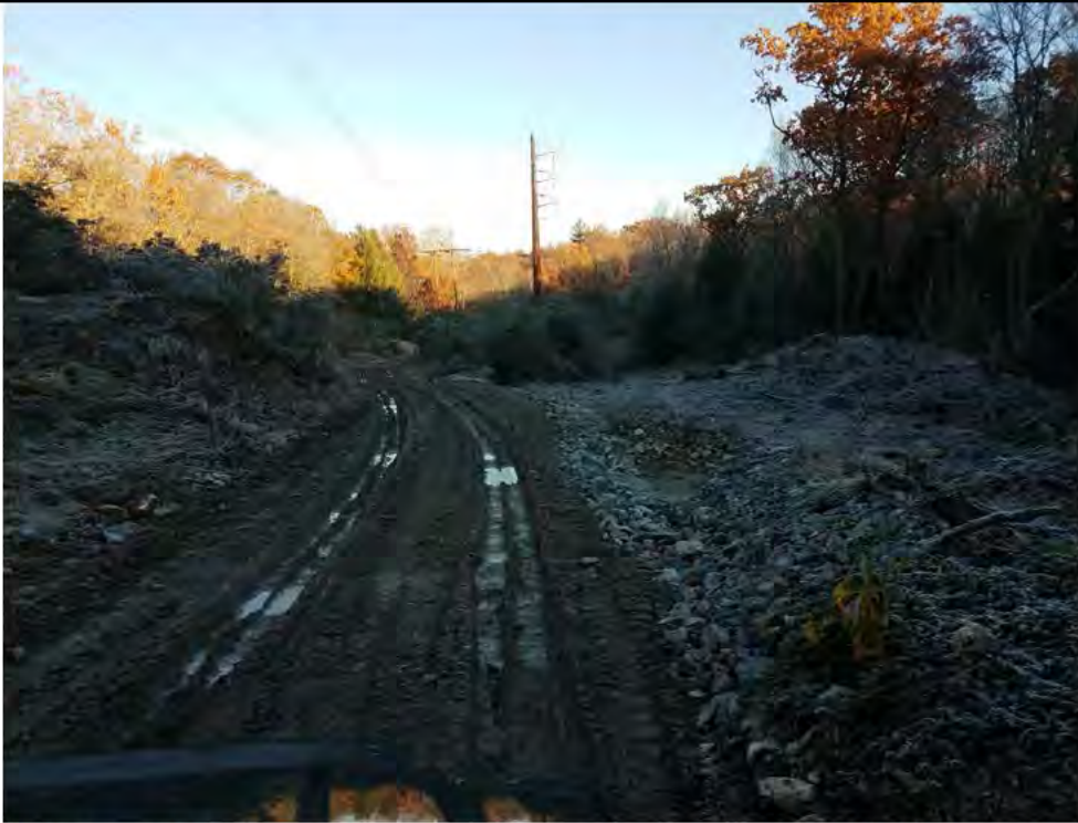
Photo 1: 11/09/17, Watertown: Map 14, access road conditions between Str38 and Str39, tire rutting, poor drainage and ponding visible, flattened water bar and poor access road grading at the sediment trap.
