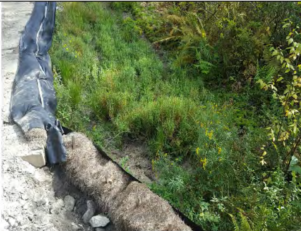
Photo 4: 09/15/17, Watertown: Map 14, at southeast corner of timber mat crossing over wetland W-C20. CORRECTIVE ACTIONS- Accumulation of sediments into wetlands cleared by hand. Photo provided by Northern of the corrective action taken, after initial inspection on 09/15/17.
