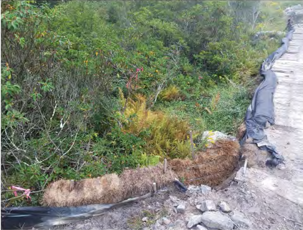
Photo 5: 09/15/2017, Watertown: Map 14, at southwest corner of timber mat crossing over wetland W-C20, excess buildup of sediments and sedimentation into W-C20, silt fence repair required. CORRECTIVE ACTION- Cleared excess sediments by hand, silt fence repair still required.
