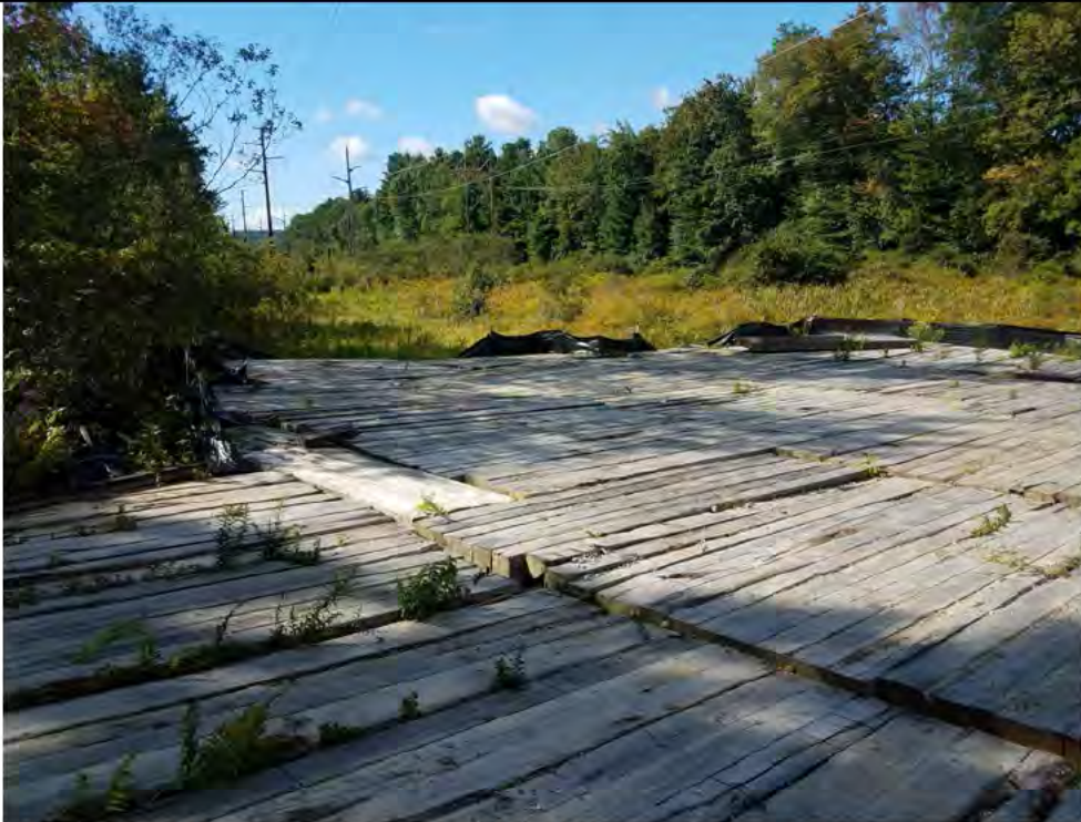
Photo 10: 09/22/17, Harwinton: Map 35, timber mat pad at Str95, perimeter silt fencing utilized to prohibit turtle access is in need of repair or removal.
