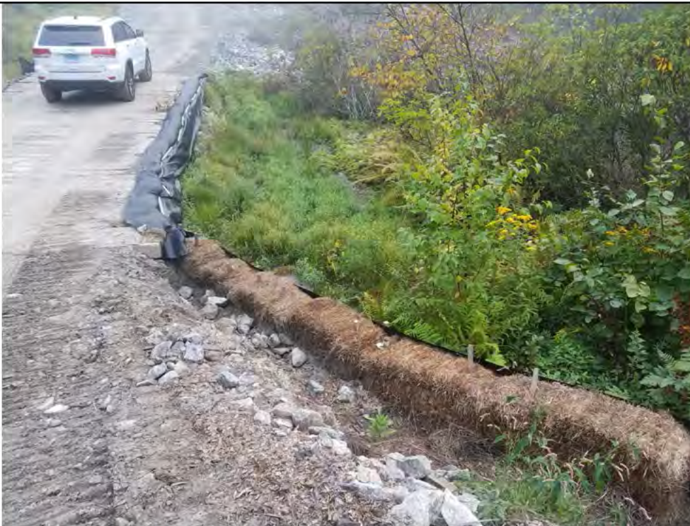
Photo 2: 09/15/17, Watertown: Map 14, at southeast corner of timber mat crossing over wetland W-C20. Corrective actions- CLEARED excess accumulation of sediments.
