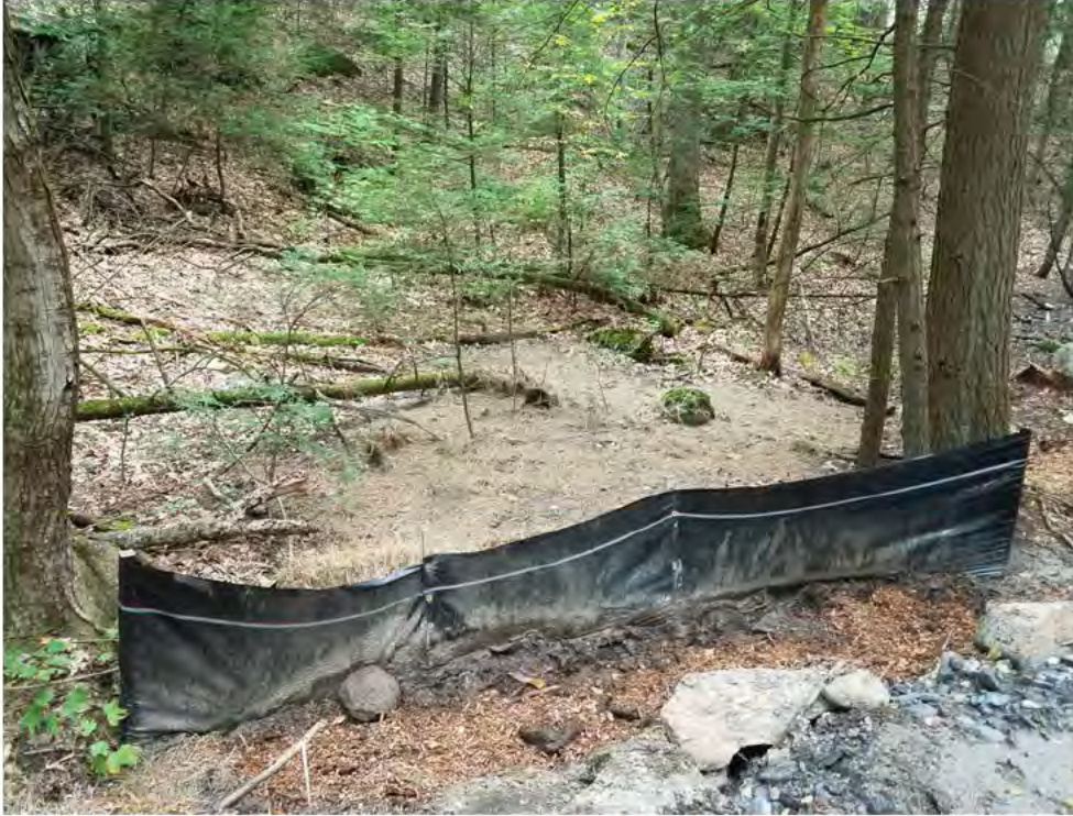
Photo 7: 09/15/17, Watertown: Map 15, access road between Str44 and Str45 approximately 100 feet north of the CT State marked Hiking trail, rills and sediment flow off access road. CORRECTIVE ACTIONS- Cleared sediments by hand and stabilized with wood chips.
