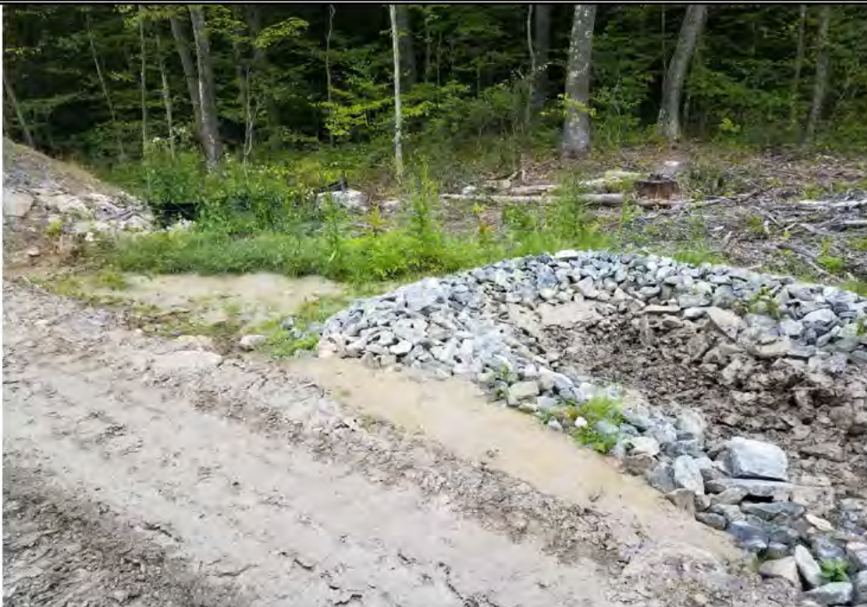
Photo 8: 09/15/17, Watertown: Map 13, south of Str36, excess sediments in temporary basin. CORRECTIVE ACTIONS- Cleared excess sediments from basin. Sediment runoff from uncontrolled storm water flow off the access road still in place.
