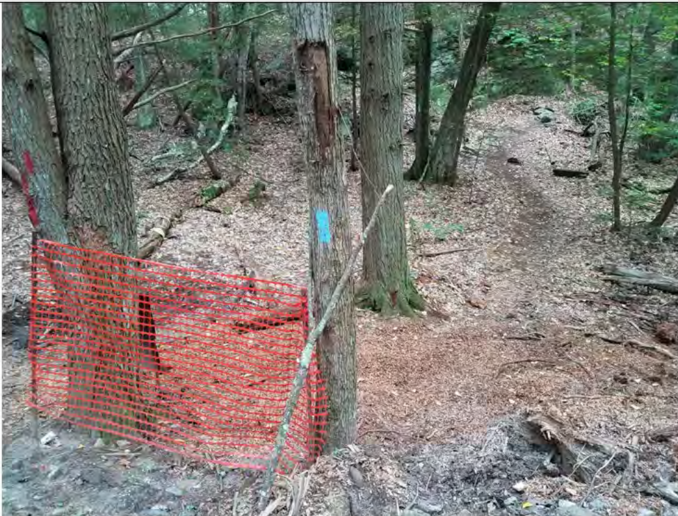
Photo 6: 09/15/17, Watertown: Map 15, access road between Str44 and Str45 at the CT State marked Hiking trail, rills and sediment flow off access road into the access point of hiking trail. CORRECTIVE ACTIONS- Cleared sediments by hand and stabilized with wood chips.
