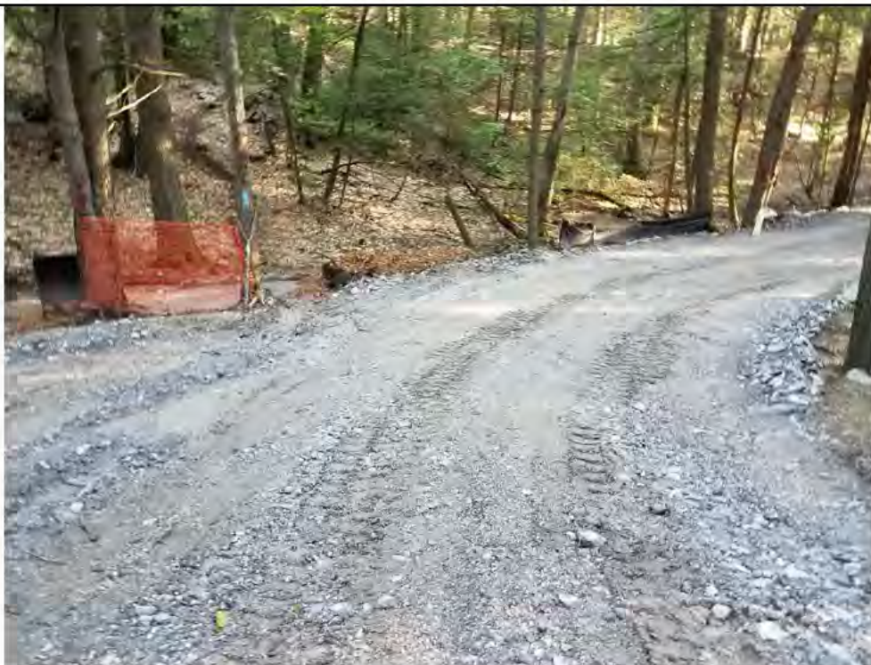
Photo 18: 09/08/2017, Watertown: Map 15, access road between Str44 and Str45 at the CT State marked Hiking trail, rills and sediment flow off access road into the access point of hiking trail.
