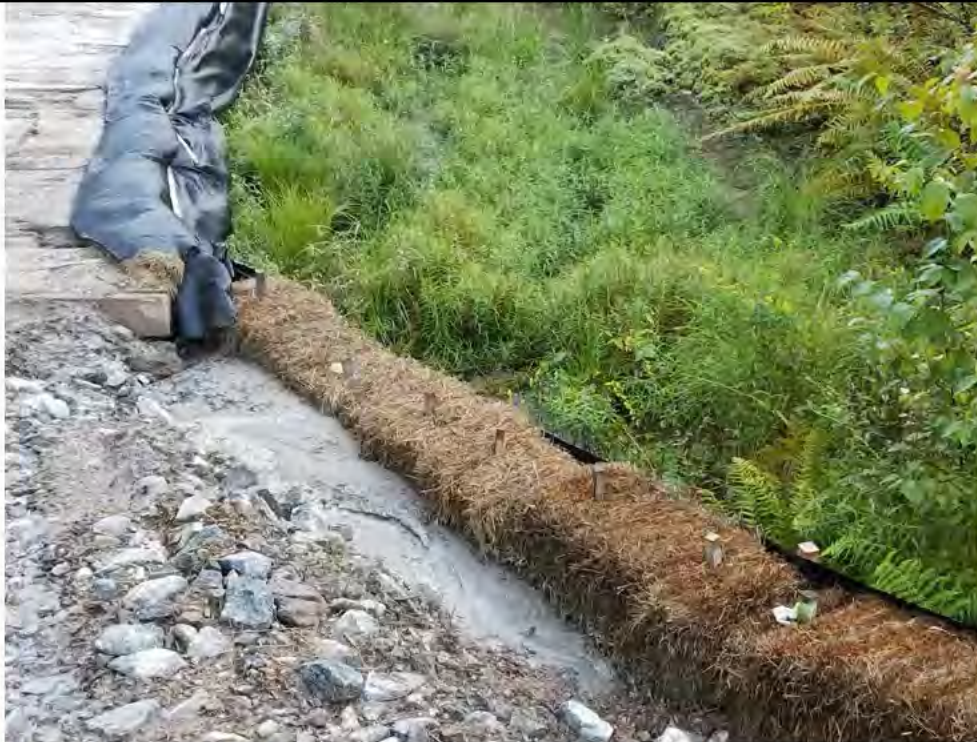
Photo 11: 09/08/2017, Watertown: Map 14, at southeast corner of timber mat crossing over wetland W-C20, excess buildup of sediments.
