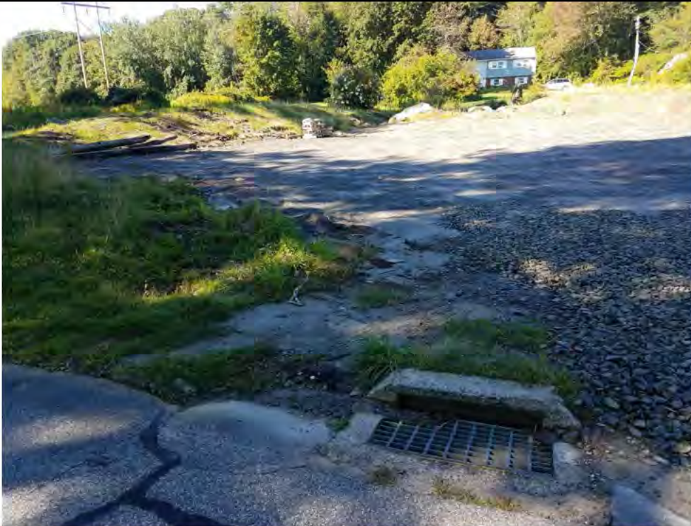
Photo 21: 09/08/2017, Litchfield, Map 29: At Str81, sediment flow into the catch basin located on Campville Road, no silt sack or catch basin protection
