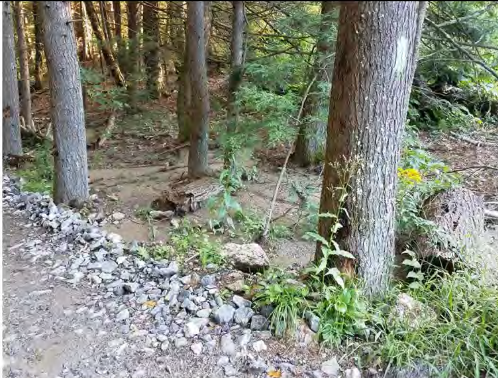
Photo 17: 09/08/2017, Watertown: Map 15, access road at Str44, rills and sediment flow off access road into wooded area.
