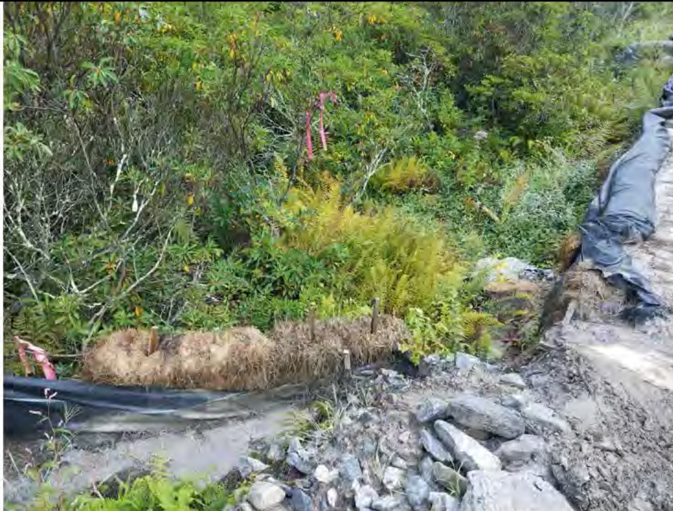
Photo 13: 09/08/2017, Watertown: Map 14, at southwest corner of timber mat crossing over wetland W-C20, excess buildup of sediments and sedimentation into W-C20.
