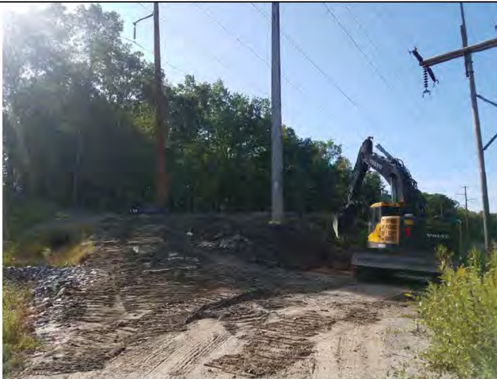
Photo 2: 09/01/2017, Thomaston/Litchfield: Maps 25-26, Eversource Maintenance crew at Str73 grading pad with excavator bucket.
