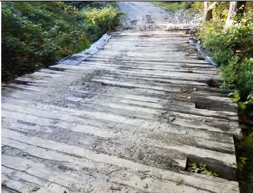
Photo 4: 09/08/2017, Watertown: Map 12, timber mat crossing at W-C15/S-C5, timbers pushed to the outside of the bend in the access road.
