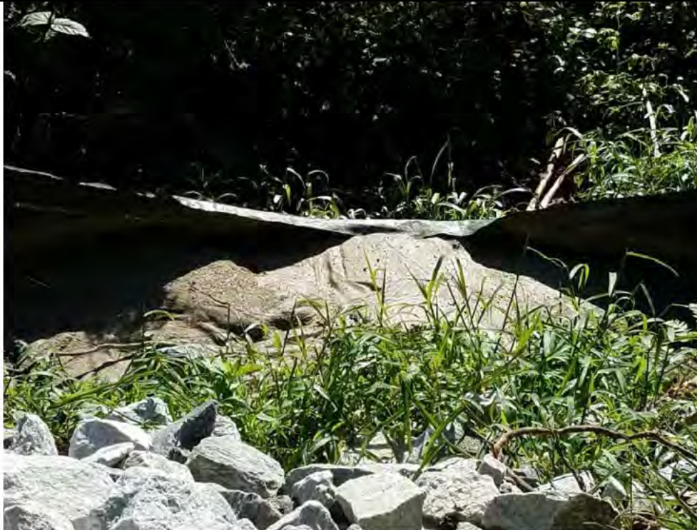
Photo 9: 09/08/2017, Watertown: Map 10, between Str26 and Str27, excess buildup of sediment in temporary sediment pond, excess buildup on silt fence.
