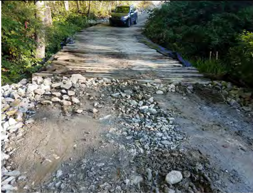
Photo 3: 09/08/2017, Watertown: Map 12, timber mat crossing at W-C15/S-C5, timbers pushed to the outside of the bend in the access road.
