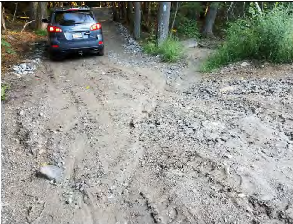
Photo 16: 09/08/2017, Watertown: Map 15, access road at Str44, rills and sediment flow off access road into wooded area.
