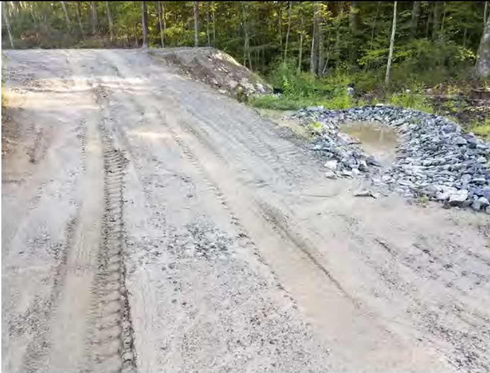
Photo 5: 09/08/2017, Watertown: Map 13, South of Str36, temporary sediment basin, movement of sediments along access road caused by storm water flow.
