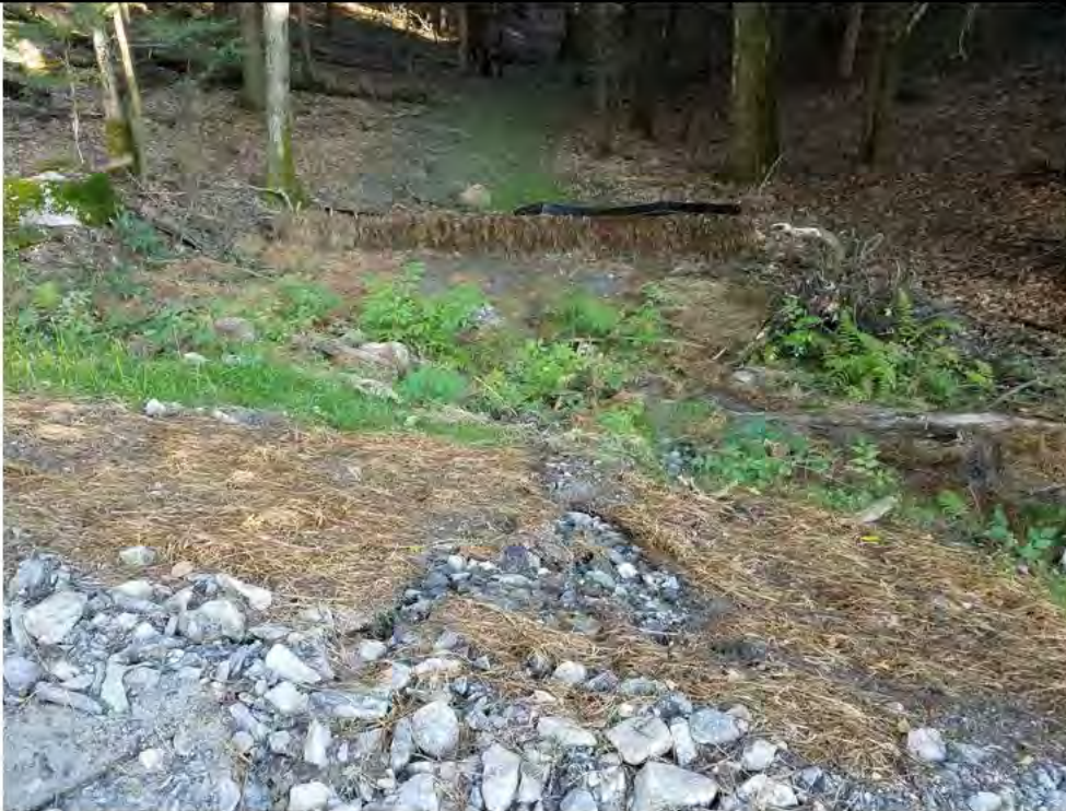
Photo 15: 09/08/2017, Watertown: Map 15, access road between Str42 and Str43, rills and sediment flow off access road, sedimentation visible down to hay bales (previously restored area).
