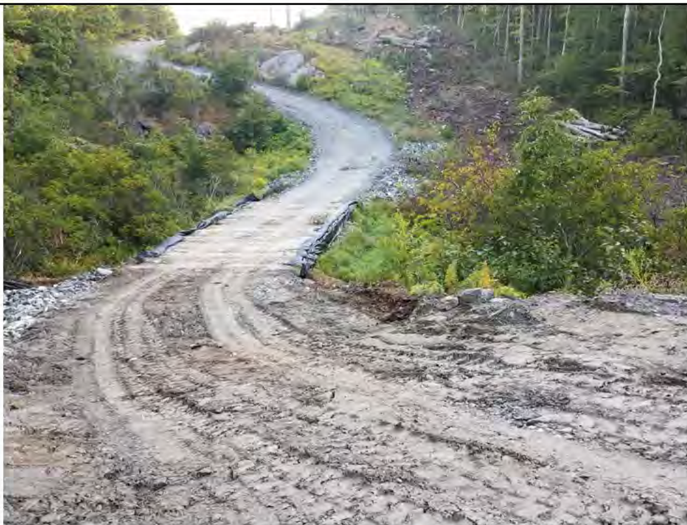
Photo 10: 09/08/2017, Watertown: Map 14, access road north of Str39 to wetland W-C20, water bar flattened out.
