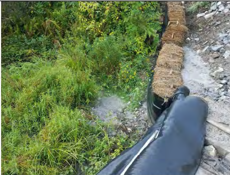
Photo 12: 09/08/2017, Watertown: Map 14, at southeast corner of timber mat crossing over wetland W-C20, excess buildup of sediments and breakthrough into W-C20.
