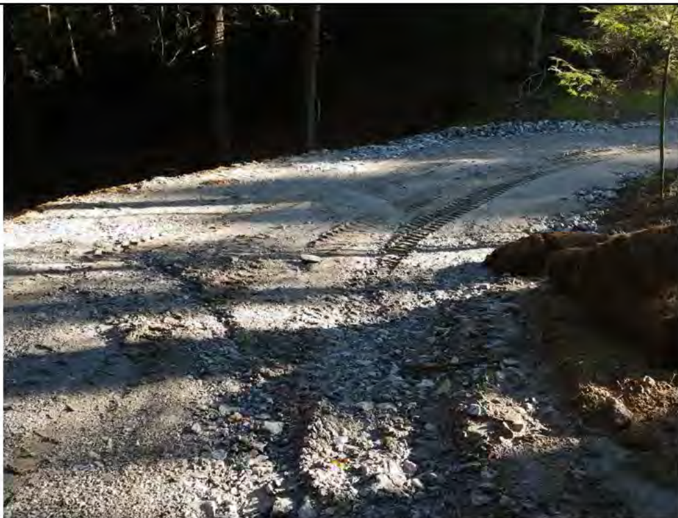
Photo 14: 09/08/2017, Watertown: Map 15, access road between Str42 and Str43, rills and visible sediment flow off outer edge of road from uncontrolled surface water flow.
