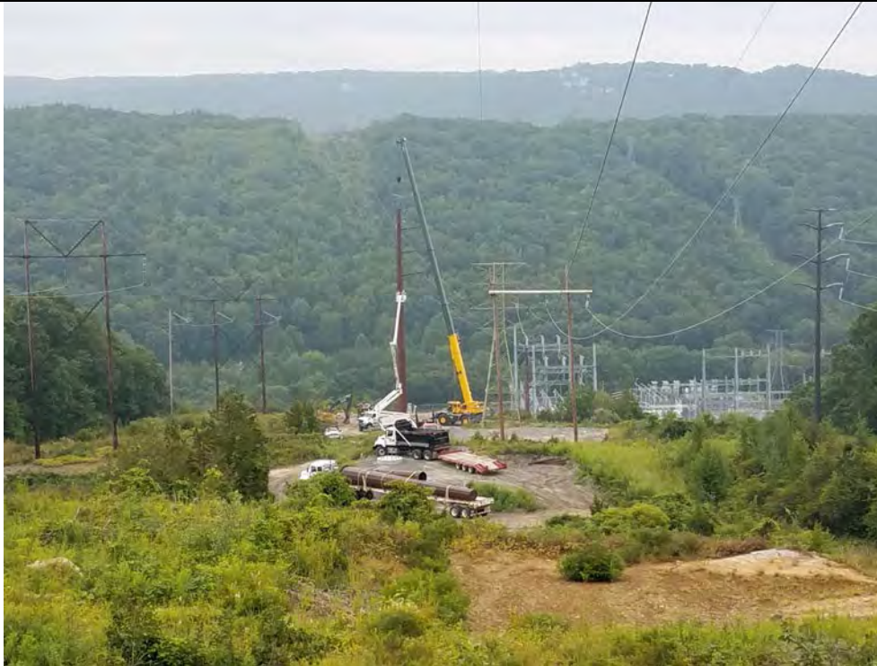
Photo 2: 08/18/17: Watertown, Map 2, Str3 and Str4, construction of a steel structure at Str3 and a trailer loaded with sections of a steel structure staged at Str4 waiting to be off loaded.
