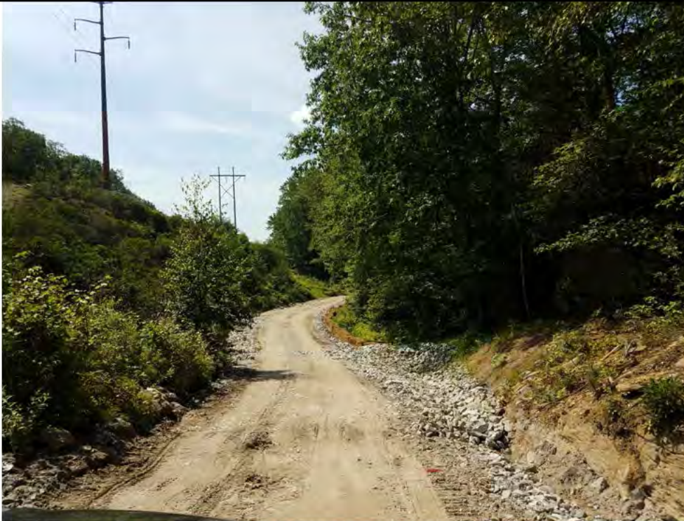
Photo 9: 08/11/17: Watertown, Map 13, access road repair by W-C18 at access road to Str37.
