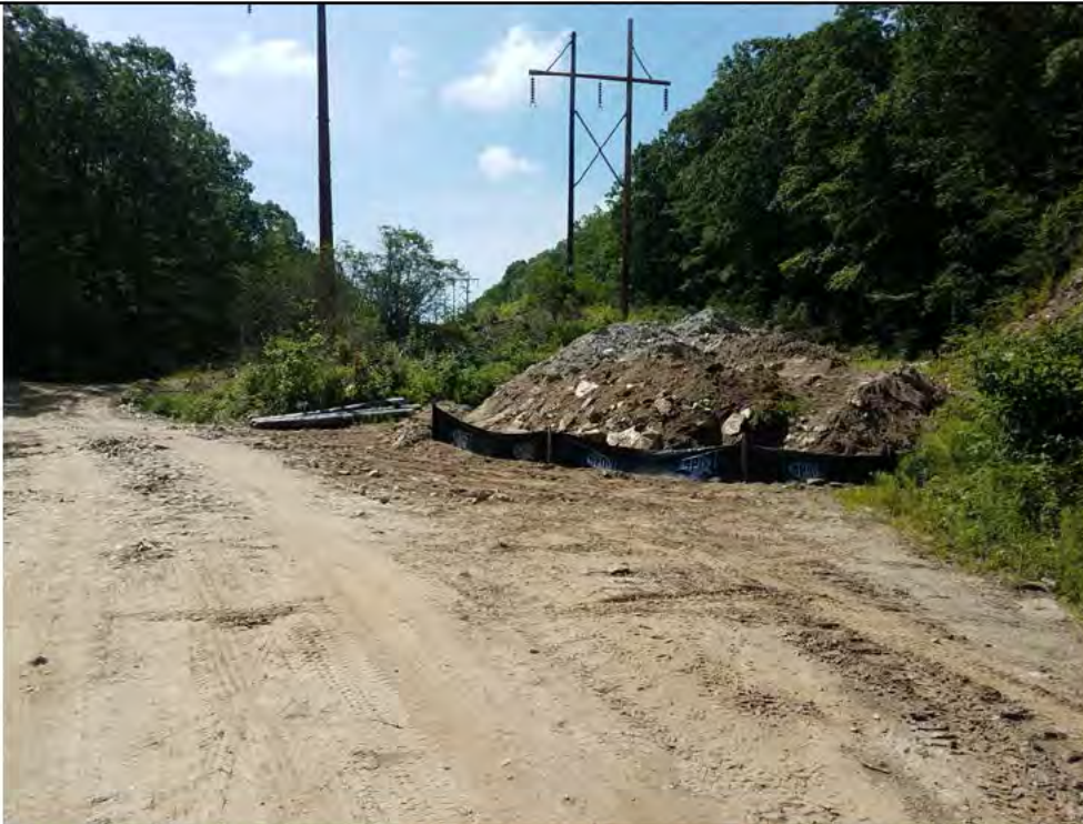
Photo 10: 08/11/17: Watertown, road base material spoils pile from new ROW access road improvements & new construction in areas between Str34 and Str43.
