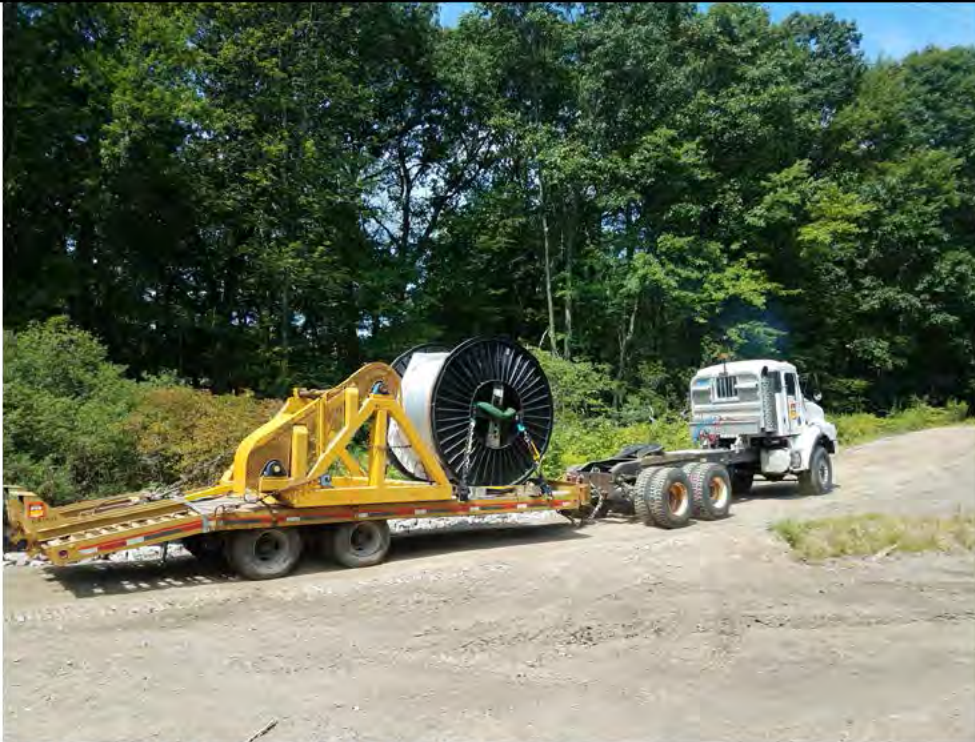
Photo 7: 08/11/17: Watertown, PAR equipment, cable feed system.
