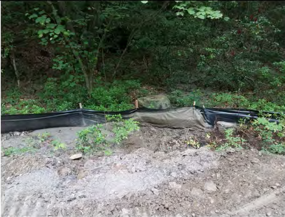
Photo 5: 06/30/2017, Watertown: Map 15, access road between Str41 and Str42, Silt fence maintenance performed.
