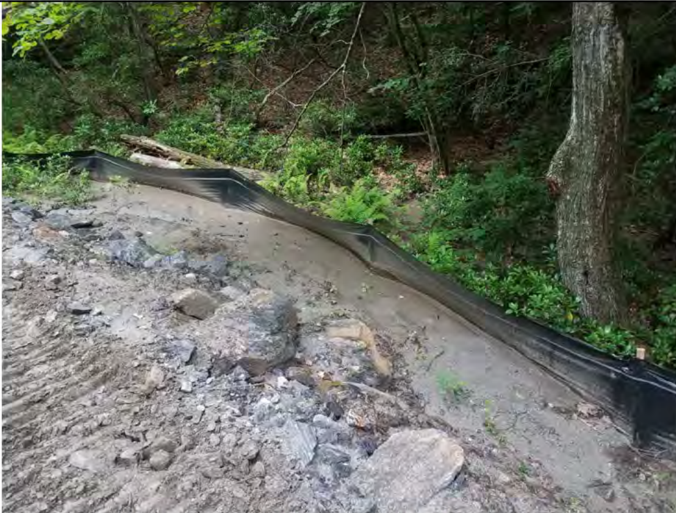
Photo 6: 6/30/2017, Watertown: Map 15, access road between Str41 and Str42, Silt fence maintenance was reportedly performed and since then a rainfall event caused more sediment buildup and the area needs to be cleared again. No noticeable change between this event and the previous Interim event Photo #2. Note the leaf by the 3rd stake in from the left on both photos, Photo #2 taken on the 6/23 and Photo #6 taken on 6/30.
