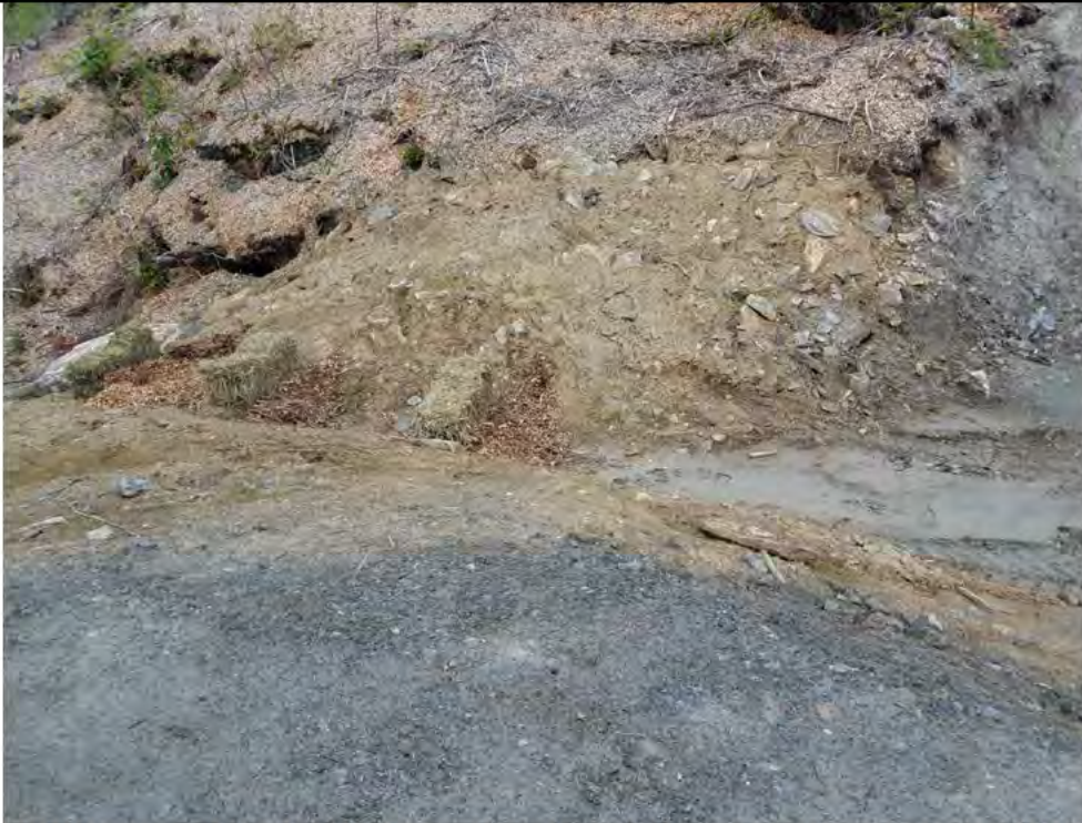
Photo 7: 06/30/2017, Watertown: Map 15, Str42 pad, at south end of the pad, storm water runoff is channeled to the slope via cut swale. Northern placed hay bales and wood chips (check dams) to capture sediments prior to slope.
