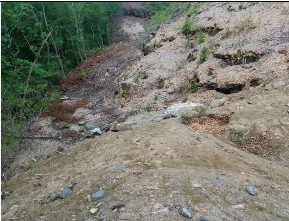
Photo 8: 06/30/2017, Watertown: Map 15, Str42 pad, at south end of the pad, Sedimentation on slope will reportedly be addressed as part of the project restoration phase.
