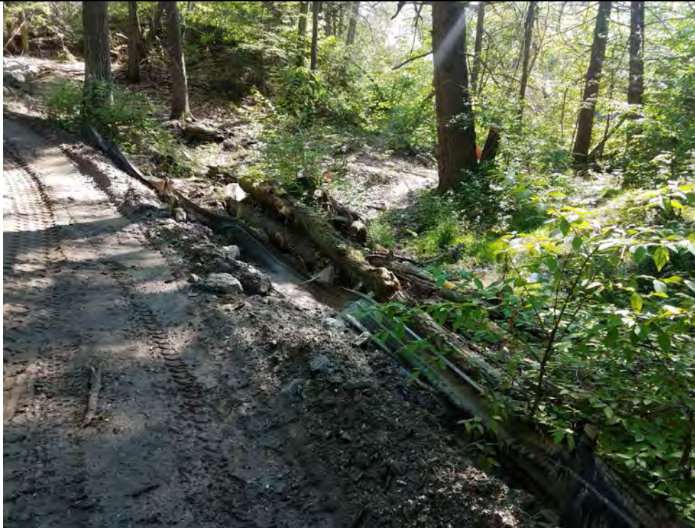
Photo 2: 06/02/2017, Watertown: Map 16, E&S control maintenance and access road improvements required at wetland W-C22.
