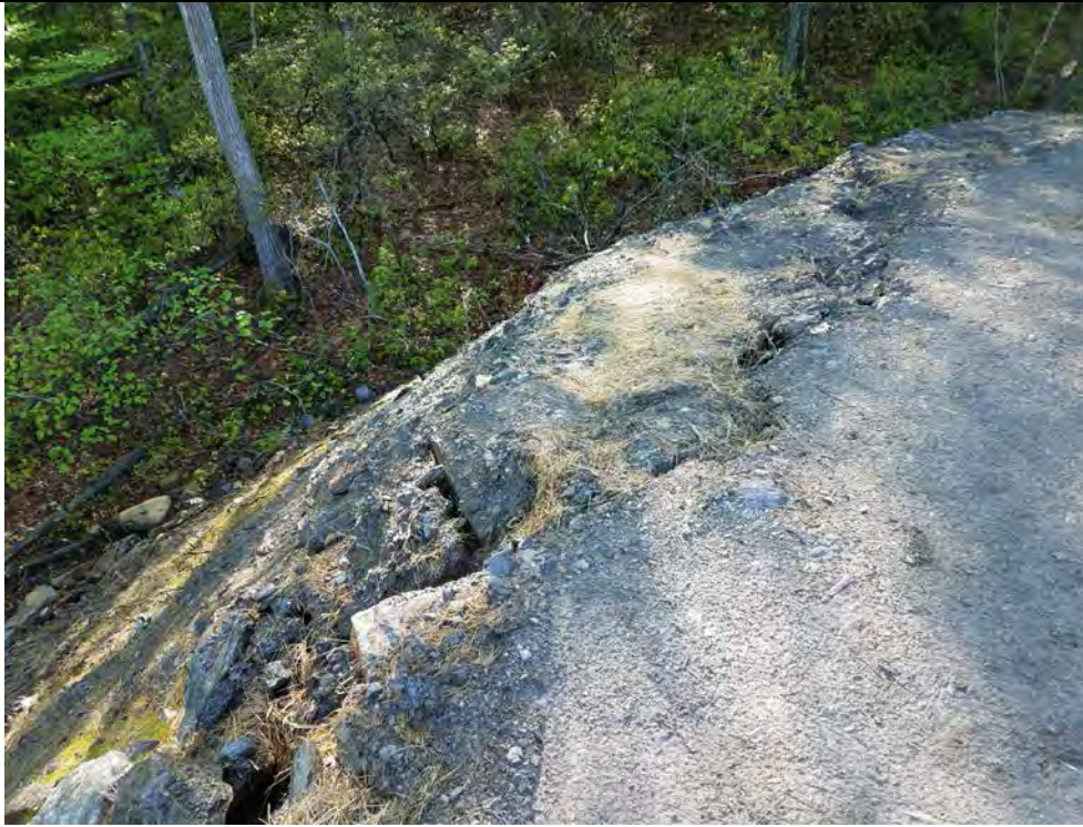
Photo 5: 05/19/2017, Watertown: Map 13, Structural failure-slope failure occurring at pad Str38.
