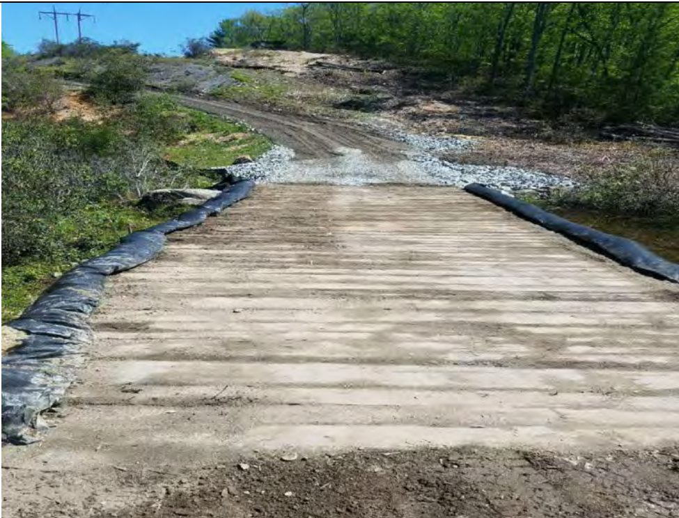
Photo 8: 05/19/2017, Watertown: Map 14, at VP-C20-1 crossing, timber mats and silt fence cleared of excess sediments, completed on 05/19/2017 by Northern.
