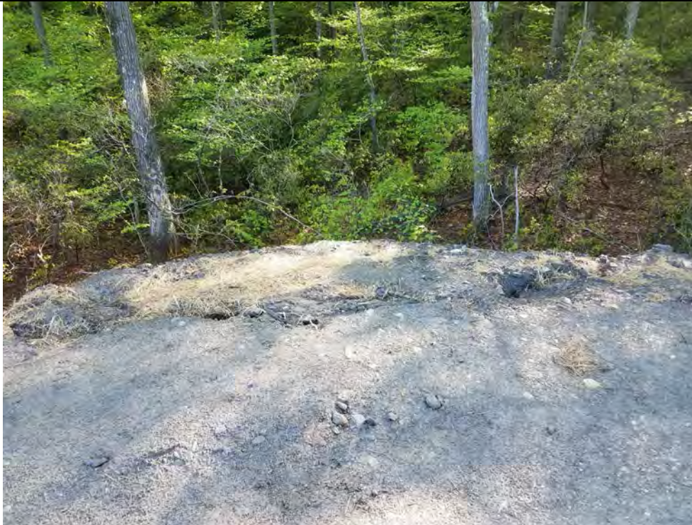
Photo 6: 05/19/2017, Watertown: Map 13, Structural failure-slope failure occurring at pad Str38.
