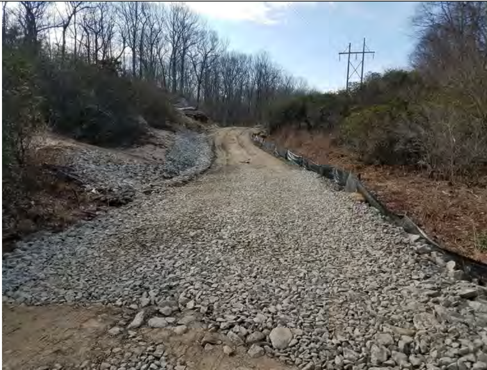
Photo 4: 4/14/2017, Watertown: Map 12, access road improvements, stone swale, and addition of perimeter silt fence.
