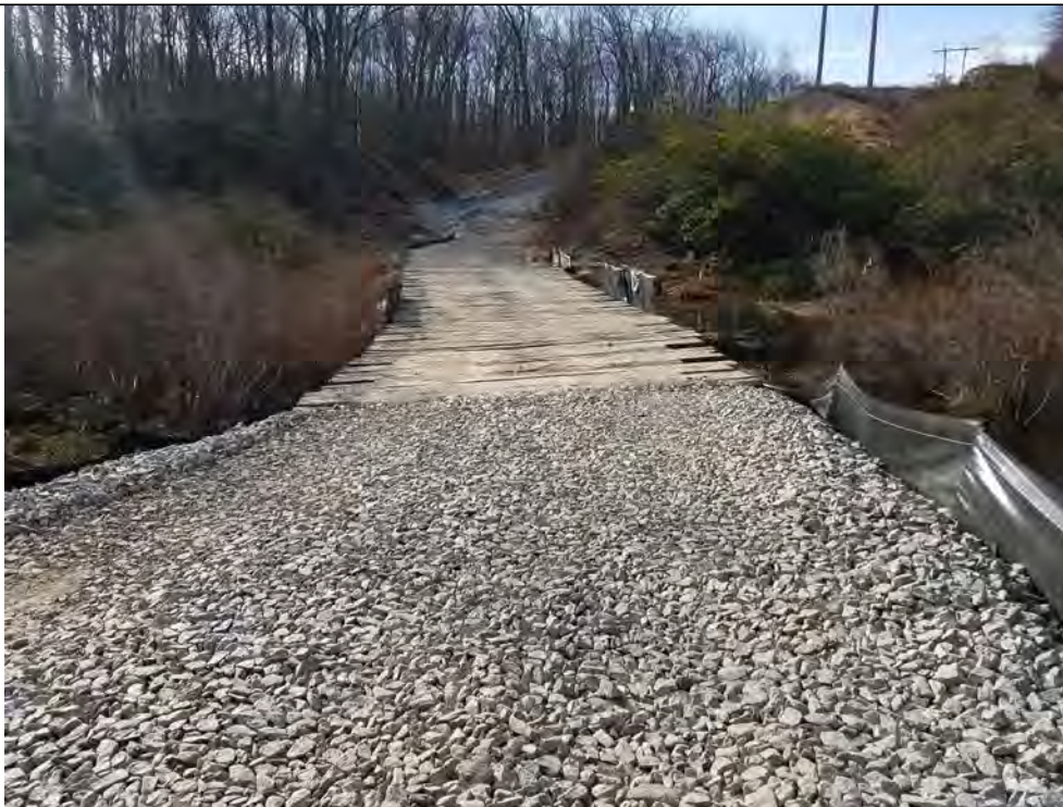
Photo 6: 4/14/2017, Watertown: Map 11, timber mat water crossing at W-C12 & VP-C12-1, access road E&S control improvements.
