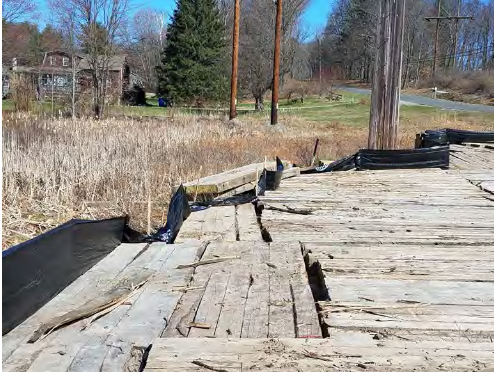
Photo 9: 4/14/2017, Harwinton: Map 35, Str95, Rare Species Avoidance and Minimization Measures, perimeter silt fence needs repair/replacement.
