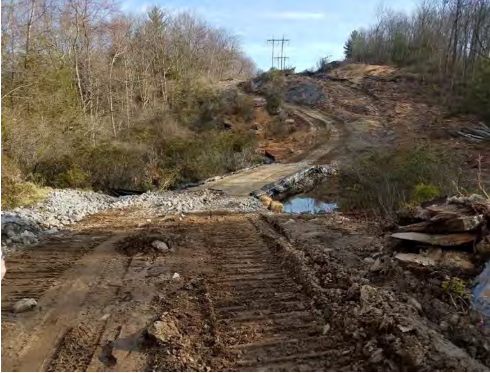
Photo 1: 4/14/2017, Watertown: Map 14, water crossing at W-C20 & VP-C20-1, Stone access tracking pads and E&S Improvements.
