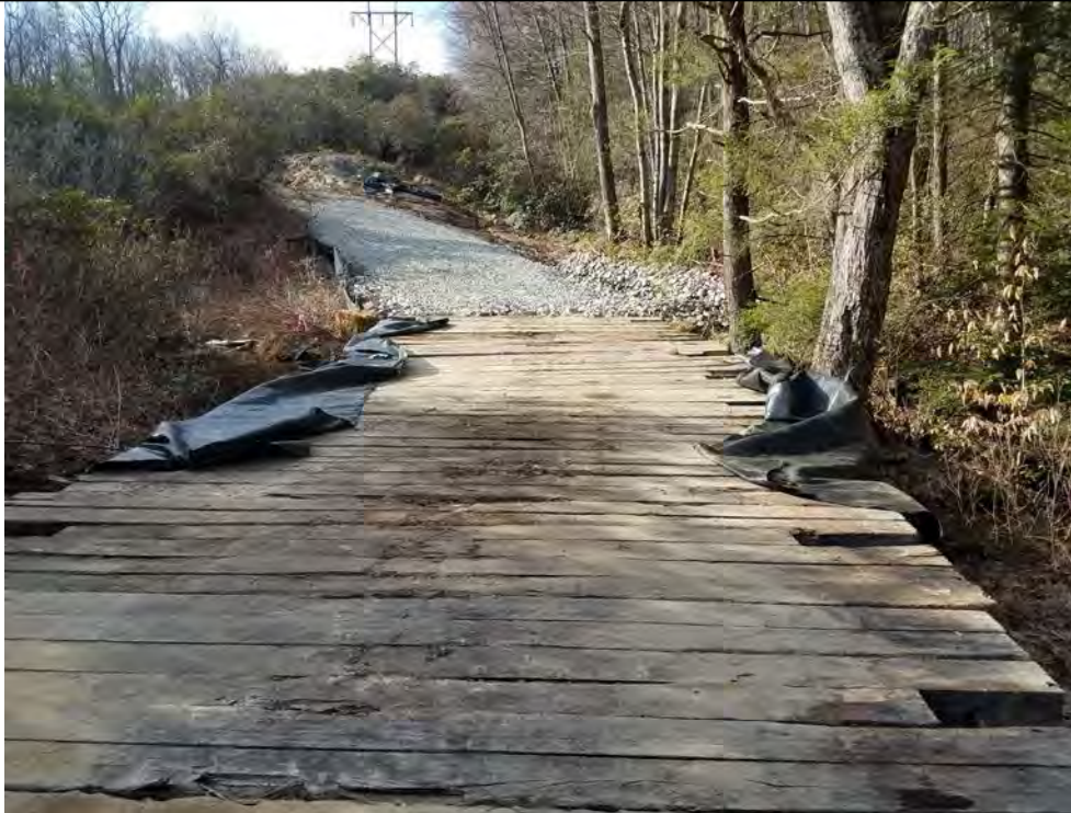
Photo 3: 4/14/2017, Watertown: Map 12, water crossing at W-C14, stone access tracking pads and E&S Improvements.
