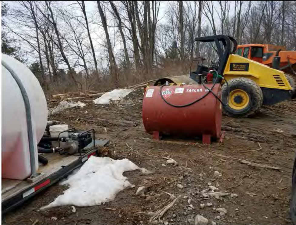
Photo 13: 3/24/2017, Litchfield: Maps 31 & 32, PAR Electric's diesel fuel storage tank (no secondary containment).
