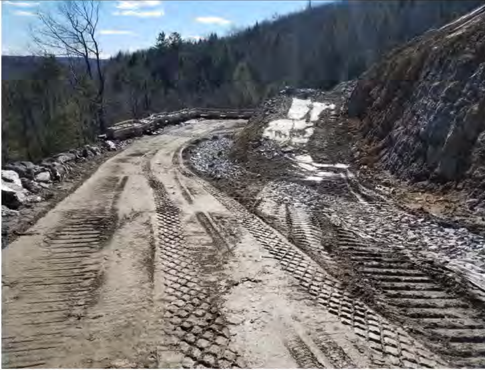
Photo 3: 3/3/2017, Litchfield: Map 31, Pad and access road construction at Str86, Str3171, and Str3231.
