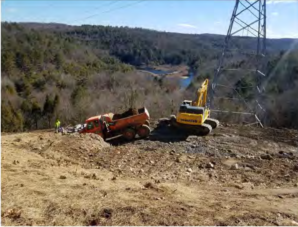
Photo 1: 3/3/2017, Litchfield: Map 31, Pad and access road construction at Str86, Str3171, and Str3231.
