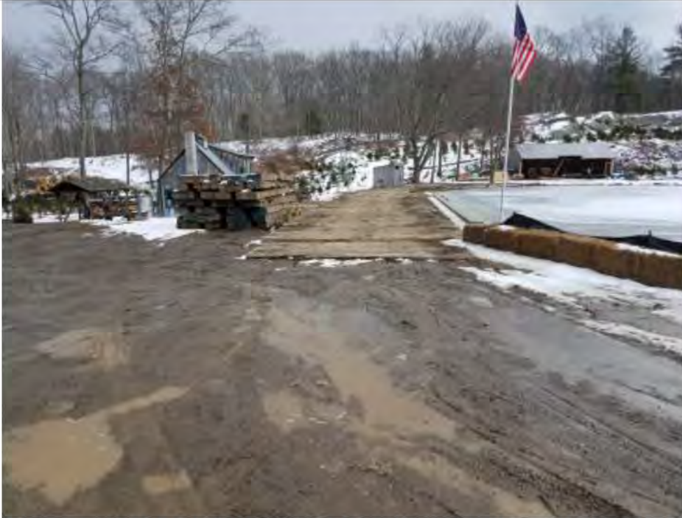
Photo 11: 2/2/2017, Thomaston: Str58 and Str59 access road maintenance, timber mats cleaned of tracked sediments.
