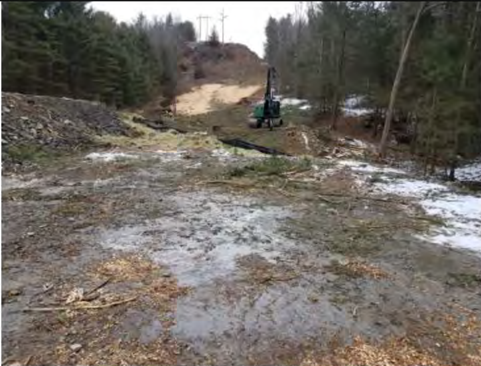
Photo 10: 2/2/2017, Harwinton: Clearing around and through W-F12 completed, equipment staged on timber mats.
