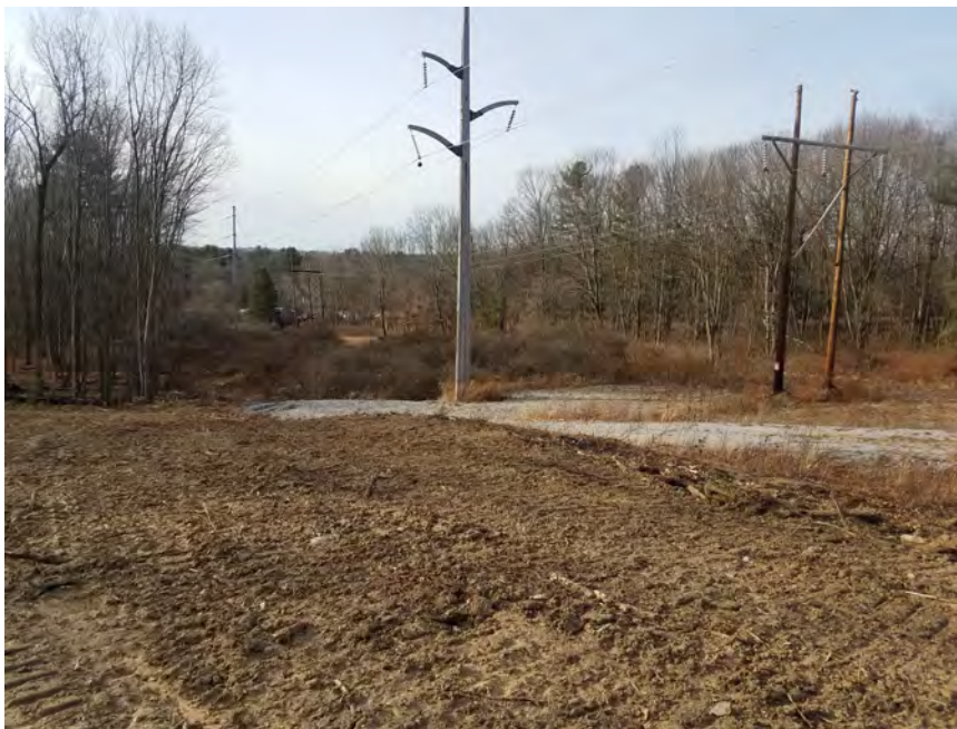
Photo #4: 1/5/2017: Harwinton, Map 35, Str97, partial access road, 25-foot buffer from wetlands W-G1
