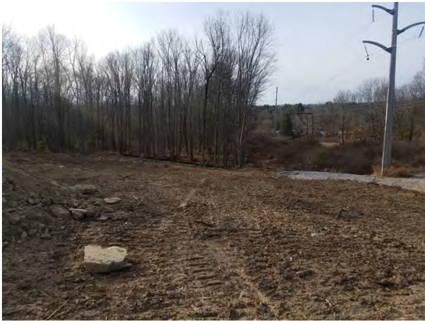
Photo #3: 1/5/2017: Harwinton, Map 35, Str97, E&S controls (Silt Fence) installed at tree line
