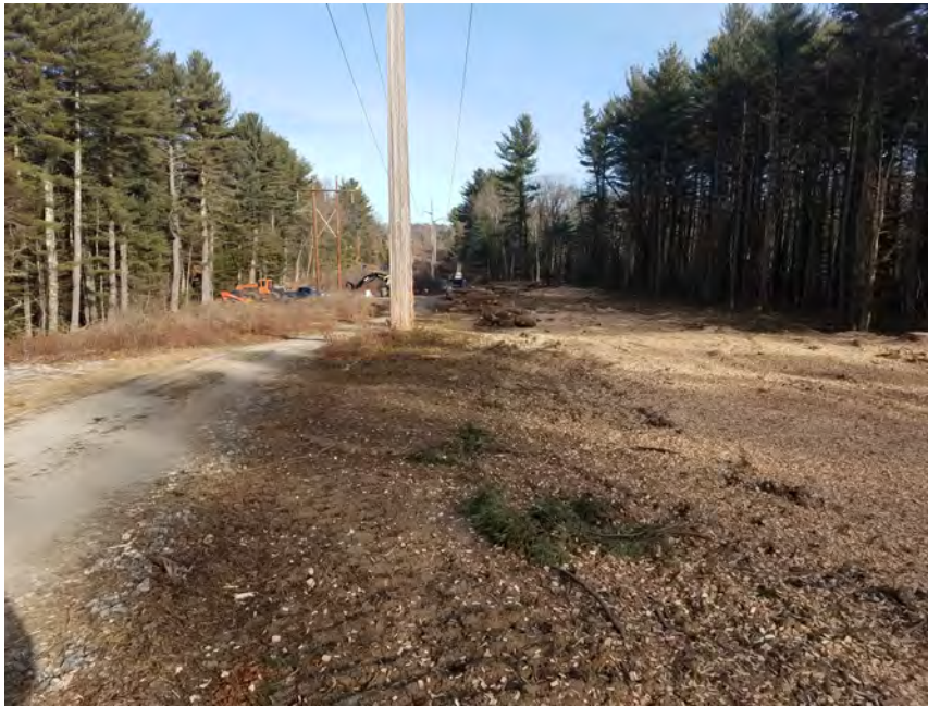
Photo #5: 1/5/2017: Harwinton, Map 33, photo taken facing north from pull pad area toward Str92, Str93 and Str94, clearing and tree removal completed, tree stumps removed, wood chips to stabilize area
