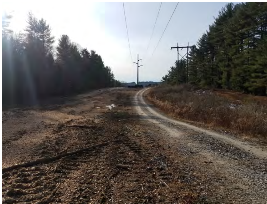
Photo #6: 1/5/2017: Harwinton, Map 33, Photo facing south from pull pad area toward Str91 and Str90, clearing and tree removal completed, wood chips to stabilize area
