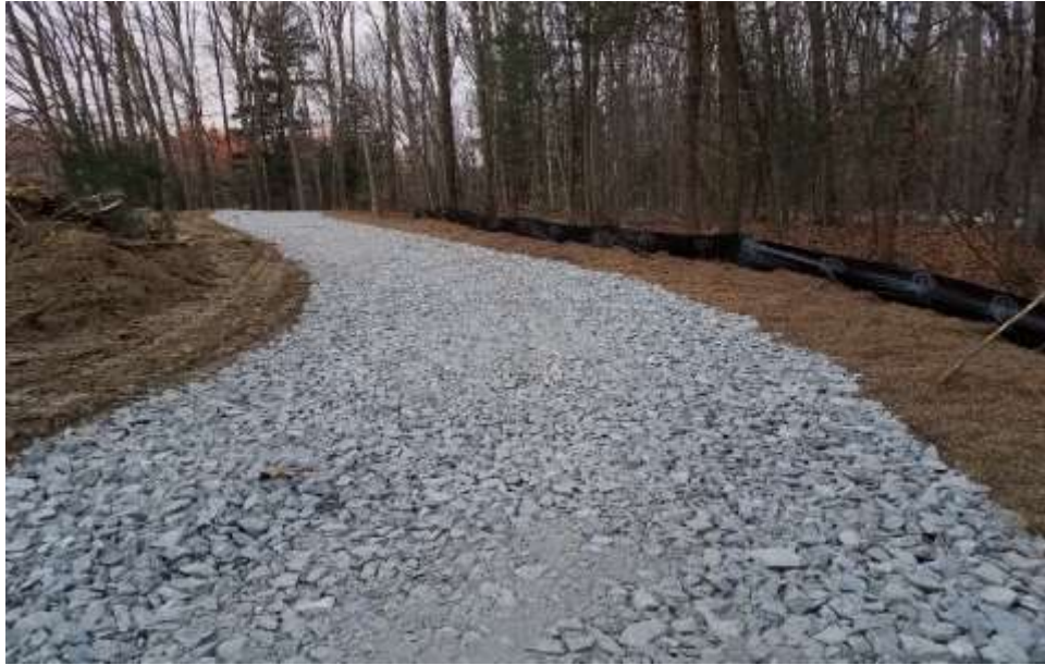
Photo #1: 12/15/16-Temporary Access Road construction and installed silt fence east of the Campville Substation Expansion Area, Town of Harwinton.
