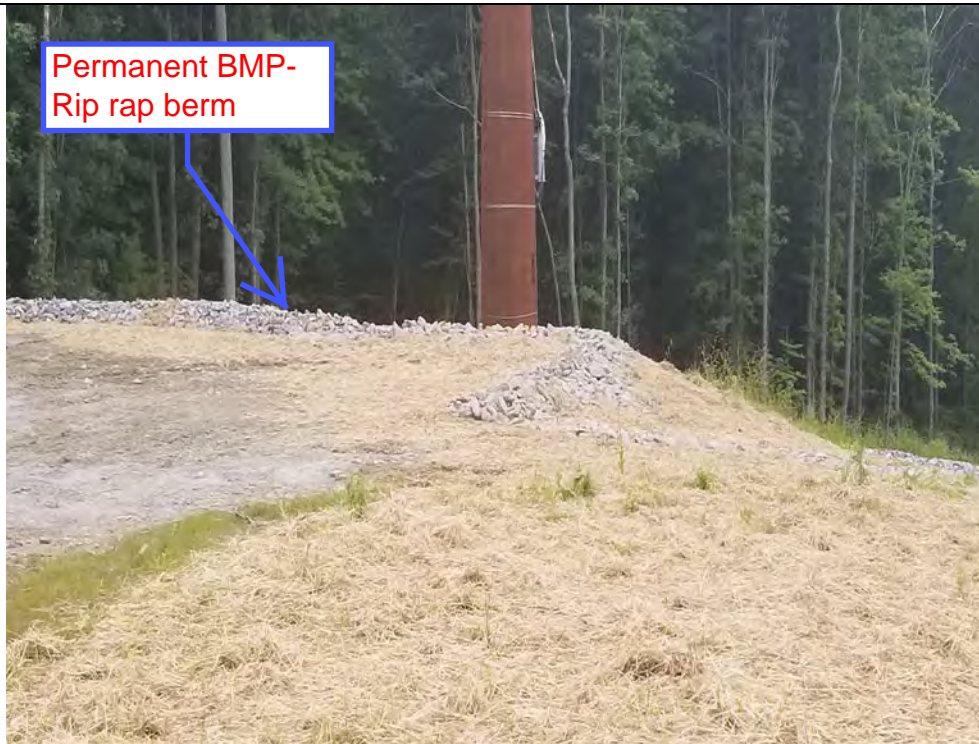
Photo 45: 08/17/2018: Harwinton, Map 35, Structure Str 97, Permanent BMPs- rip rap berm and rip rap armored slopes, drainage swale at points of stormwater runoff, seed and mulch.
