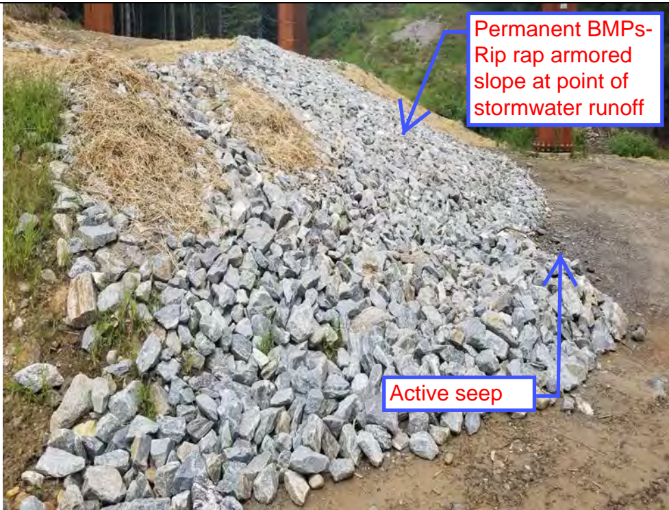
Photo 42: 08/17/2018: Harwinton, Map 32, Structure Str 87, Permanent BMPs- rip rap berm and rip rap armored slopes at points of stormwater runoff, active seep at toe of slope.
