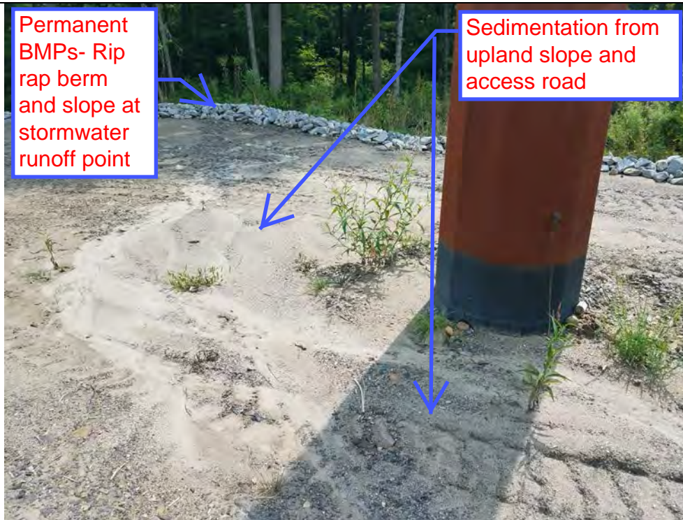
Photo 35: 08/17/2018: Litchfield, Map 29, Structure Str 83, sediment buildup from erosion off of upland slope and sediments moving over pad area during rainfall events, Permanent BMPs- rip rap berm at points of stormwater runoff.
