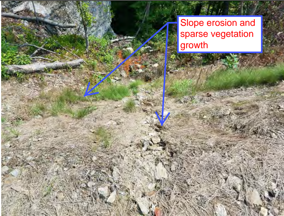
Photo 7: 08/16/2018: Watertown, Map 10, Structure Str 27, slope erosion and sparse vegetation growth.
