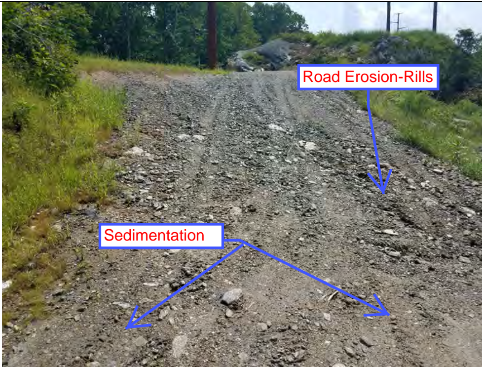
Photo 8: 08/16/2018: Watertown, Map 11, Structure Str 31, access road erosion.
