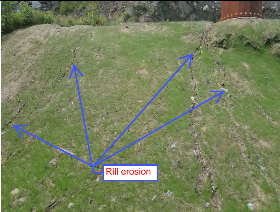
Photo 41: 08/17/2018: Litchfield, Map 31, Structure Str 3236, down gradient slope, work pad, erosion and bare soils areas, vegetation growth.
