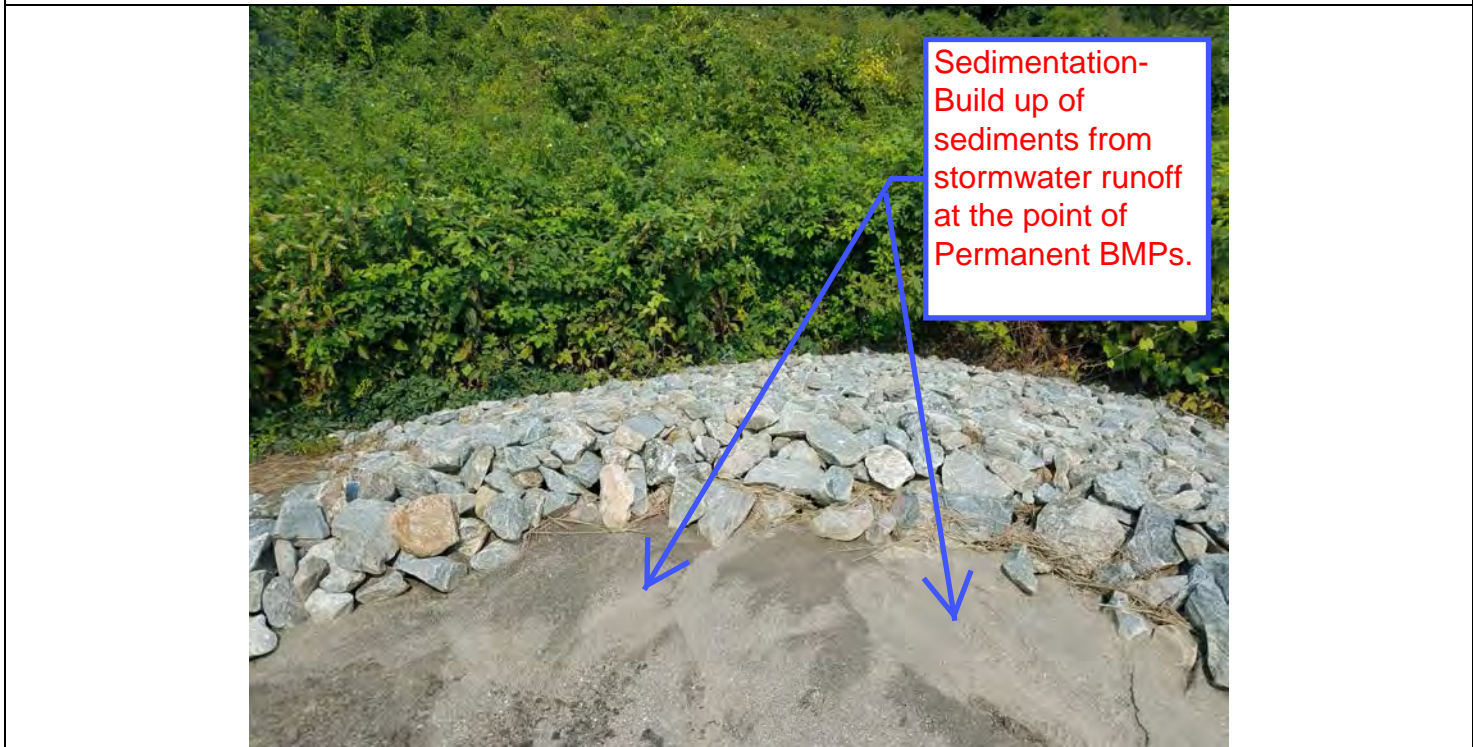
Photo 4: 08/16/2018: Watertown, Map 08, Structure Str 20, sediment build up at corner of pad, Permanent BMPs-rip rap berm and rip rap armored slope at point of stormwater runoff.
