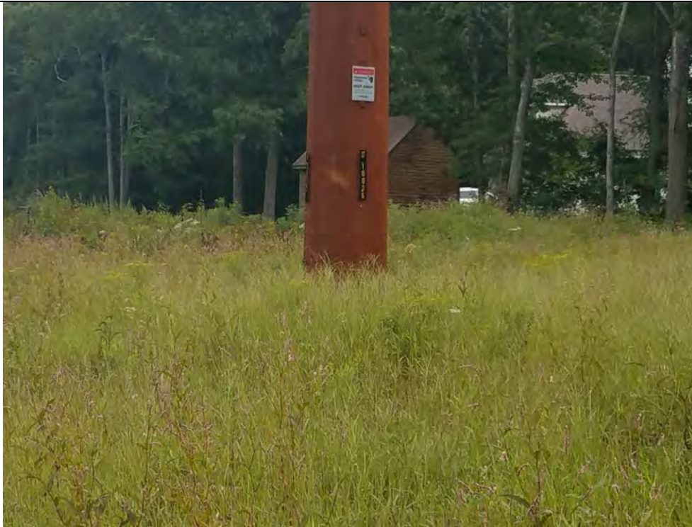
Photo 33: 08/17/2018: Litchfield, Map 27, Structure Str 77, vegetation growth.
