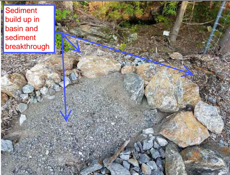
Photo 16: 08/17/2018: Thomaston, Map 17, Structure Str 47, full sediment basin, sediment passing through improperly constructed sediment basin and traveling down gradient.
