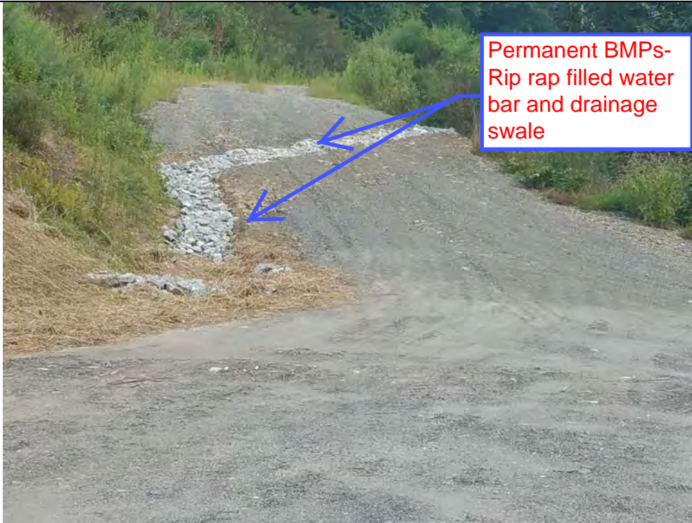
Photo 31: 08/17/2018: Thomaston, Map 25, Structure Str 70, Permanant BMPs- rip rap filled water bar and swale.
