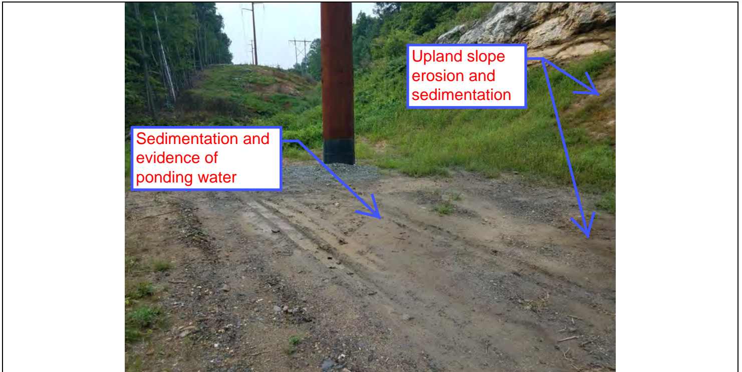
Photo 25: 08/17/2018: Thomaston, Map 20A, Structure Str 60, upland slope erosion and sedimentation and ponding conditions on access road.
