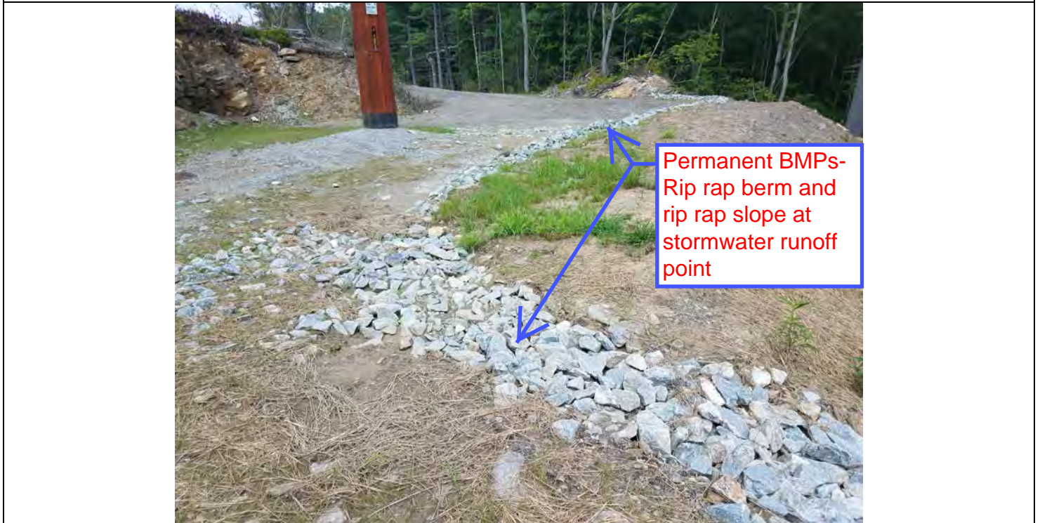
Photo 12: 08/16/2018: Watertown, Map 12, Structure Str 35, implemented Permanent BMPs- rip rap berm and rip rap slope at point of stormwater runoff.
