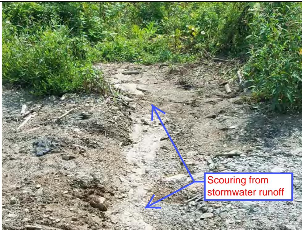
Photo 36: 08/17/2018: Litchfield, Map 29, Structure Str 83, erosion off of pad and access road from non-armored/rip rap lined water bar.
