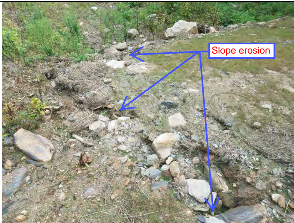
Photo 30: 08/17/2018: Thomaston, Map 24, Structure Str 69, soil berm constructed along top edge of slope, erosion off and down slope.
