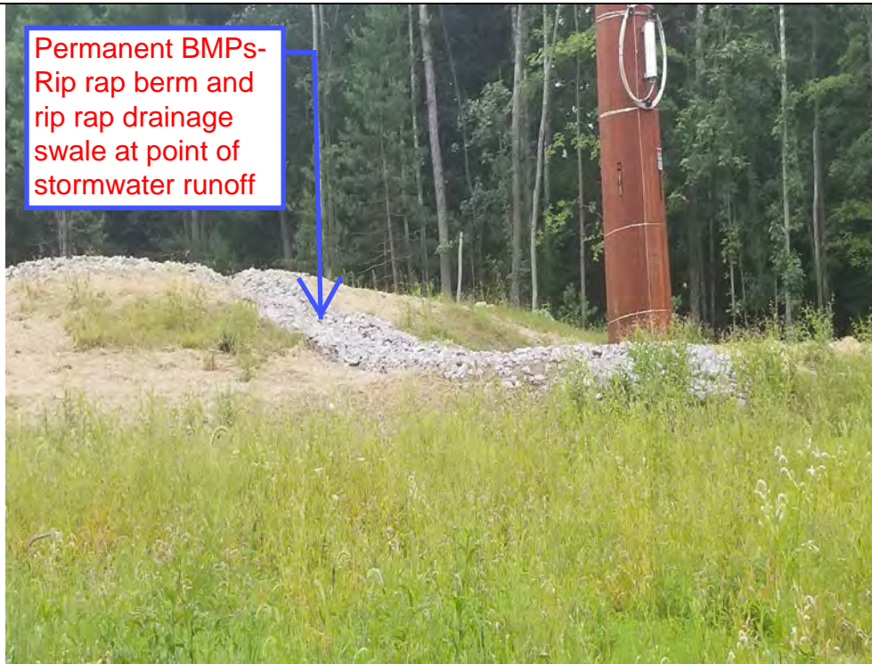
Photo 46: 08/17/2018: Harwinton, Map 35, Structure Str 97, Permanent BMPs-rip rap berm and rip rap armored slopes, drainage swale at points of stormwater runoff, seed and mulch and vegetation growth.
