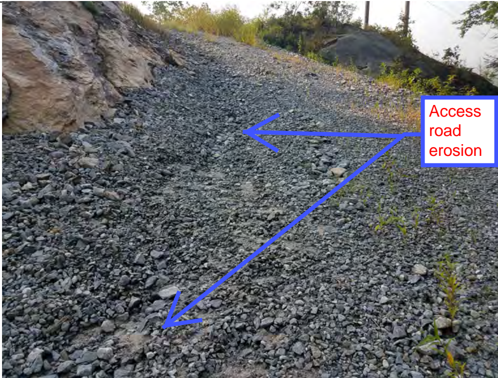
Photo 15: 08/17/2018: Thomaston, Map 17, Structure Str 47, access road erosion and sediment buildup in water bar.
