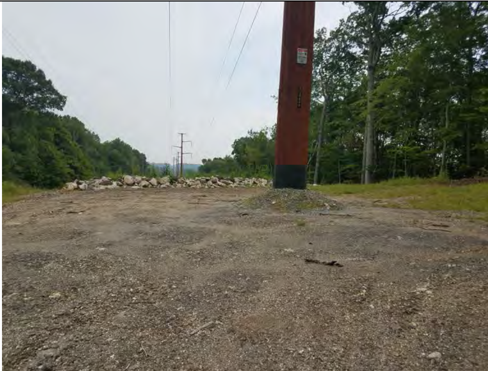
Photo 23: 08/17/2018: Thomaston, Map 20A, Structure Str 59, typical pad construction (native materials) in this area of the ROW.
