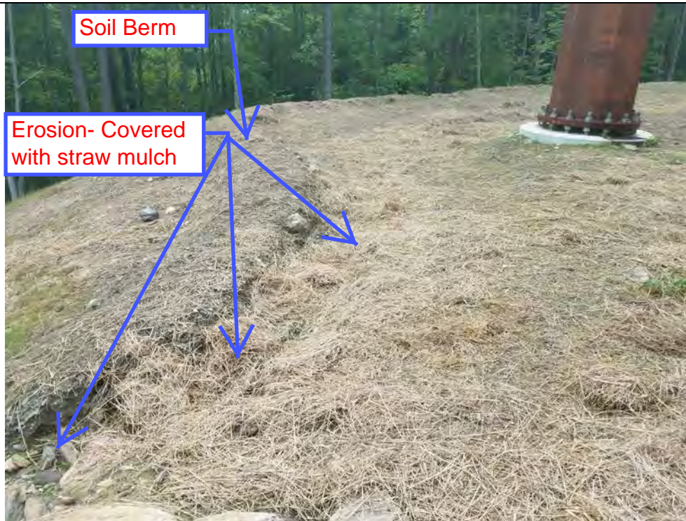
Photo 29: 08/17/2018: Thomaston, Map 24, Structure Str 69, Seeding and straw mulch cover on pad, soil berm constructed along top edge of slope, erosion off and around open edge of slope.
