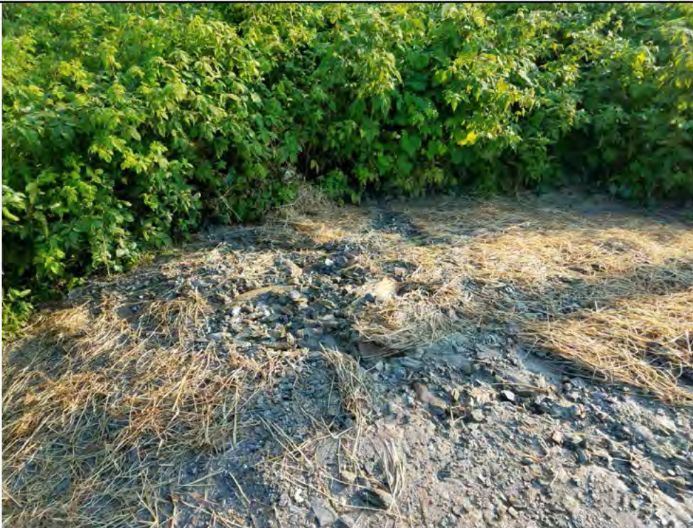
Photo 14: 07/27/2018, Watertown: Map 08, Str20 pad and slope area, slope erosion at north corner of pad. Straw mulch placed on slope surfaces, no seeding of slope.
