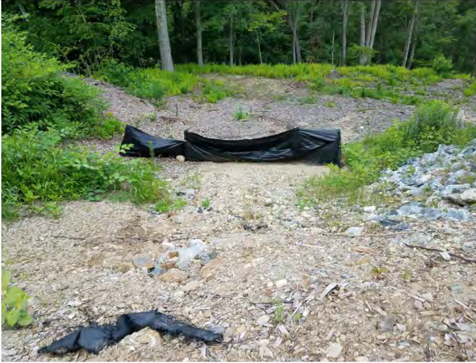
Photo 1: Interim Report # 42, Photo 2: 07/06/2018, Watertown: Map 01, Str1A pad slope erosion, no stabilization. Photo taken facing north CT wetland. SEE PHOTO 1A and 1B FOR CORRECTIVE ACTIONS, PERMANENT BMPs.
