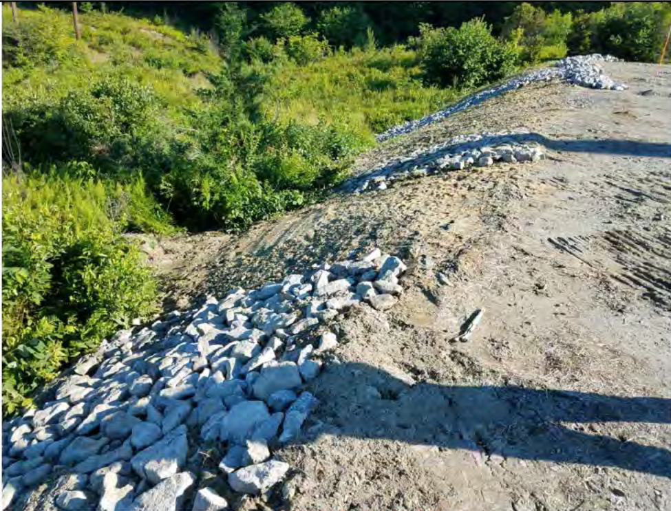
Photo 2A: 07/20/2018, Watertown: Map 03, Str07, CORRECTIVE ACTION - Rip rap armored slope in areas of slope erosion as shown in Photo 2.
