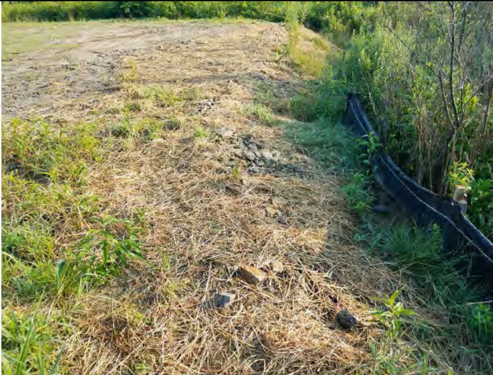
Photo 11: 07/27/2018, Watertown: Map 07, Str18 work pad and slope, slope erosion occurring, silt fence maintenance needed (tattered and sagging due to sediment buildup). Stabilization measures in place consists of a single layer of stone (inconsistently placed with areas of exposed soils) and straw mulch placed on slope (no grass seed applied to pad slopes). Sediments have accumulated at the toe of the slope due to recent heavy rainfall events. Photo taken facing east. See Photo 12 for additional view.
