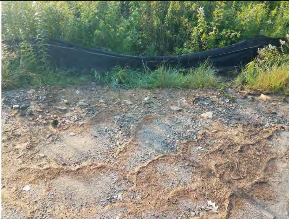
Photo 9: 07/27/2018, Watertown: Map 07, Str18 work pad, fine sediments continue to wash out of exposed non-stabilized/non-vegetated soils and slope erosion is occurring. Observed failing E&S with sediments passing under/through silt fence (see Photo 10). Silt fence maintenance is needed per the BMPs.
