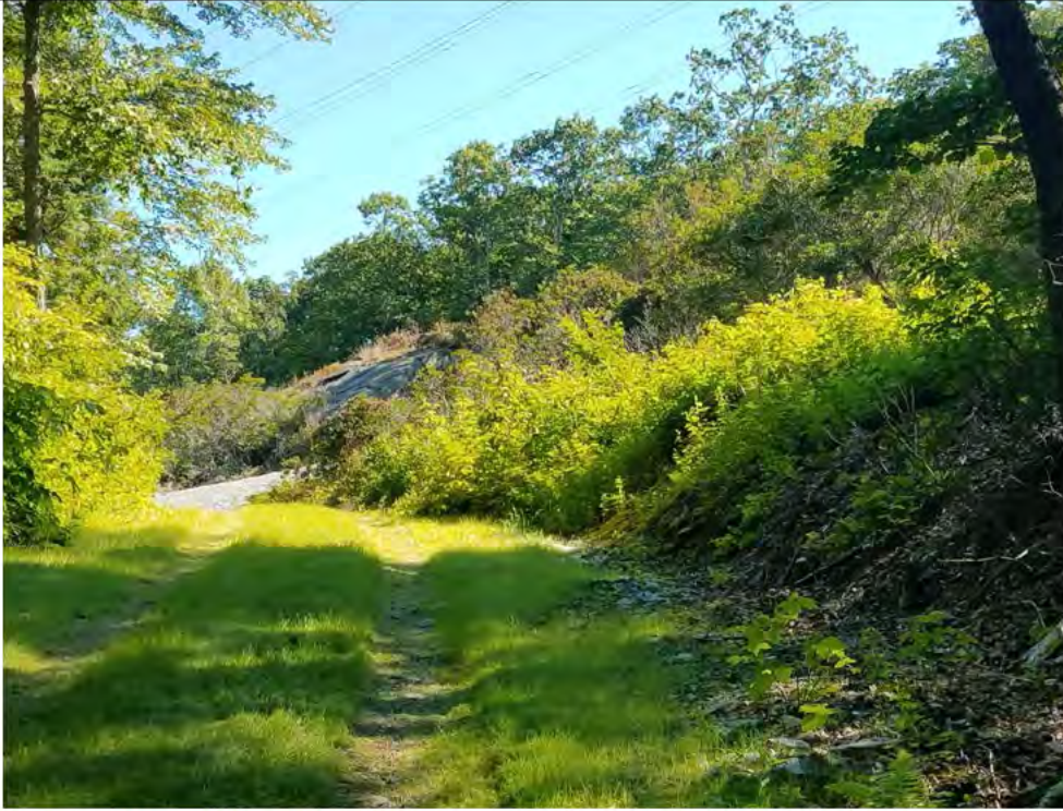
Photo 3: 07/20/2018, Watertown: Maps 11-13, access roads between Str32 and Str38, observed multiple stretches of the access road with varying degrees of vegetation (grass) growth.
