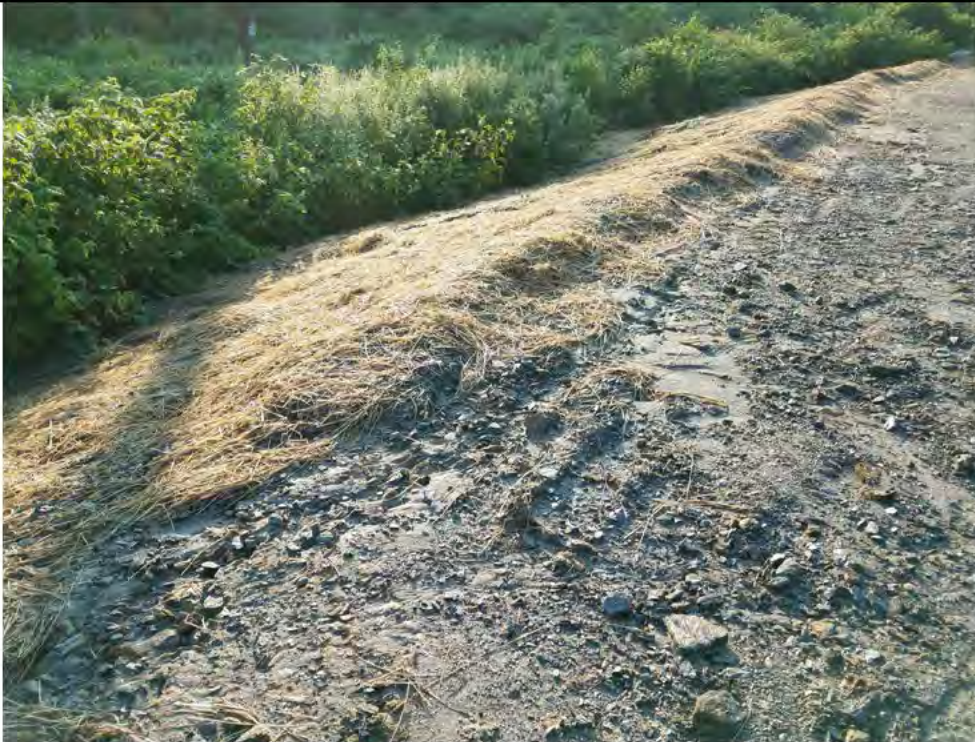
Photo 13: 07/27/2018, Watertown: Map 08, Str20 pad and slope area, erosion off end of berm area (north to east corner of work pad). Photos 13-16 are additional views of conditions at Str20.
