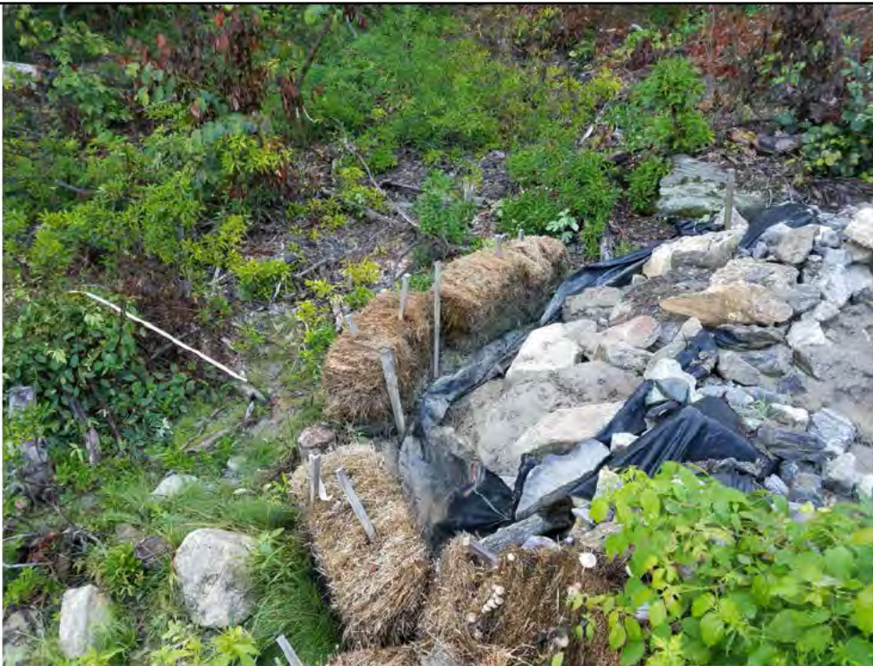
Photo 22: 07/27/2018, Watertown: Map 12, access road between Str34 and Str35, water bar and sediment trap, overloaded with fines, failing silt fence and degraded straw bales, sediments breaking through and moving toward wetland W-C15.
