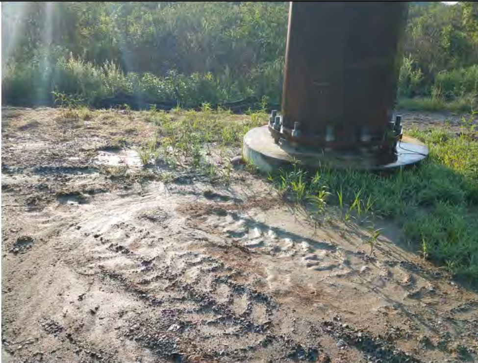
Photo 8: 07/27/2018, Watertown: Map 07, Str18 work pad, fine sediments continue to wash out of exposed non-stabilized/non-vegetated soils during rain events. Sediments appear to be accumulating on the upland side of the structure foundation. Photo taken facing southeast.
