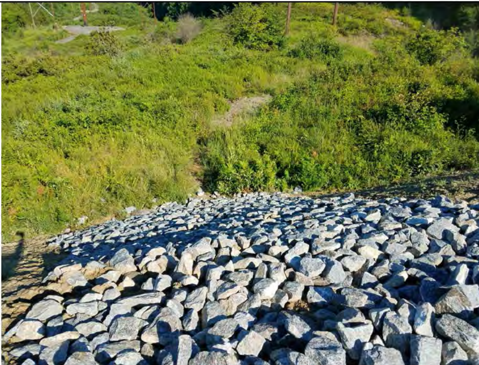
Photo 2C: 07/20/2018, Watertown: Map 03, Str07, CORRECTIVE ACTION - Rip rap armored slope in areas of slope erosion as shown in Photos 2 and 2B.
