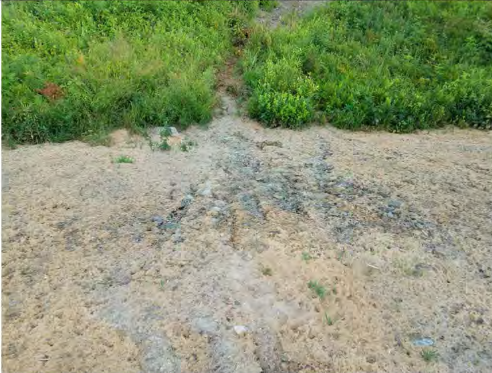
Photo 2B: Interim Report # 42, Photo 4: 07/06/2018, Watertown: Map 03, Str05 pad and slope erosion, no stabilization. Photo taken facing north.
