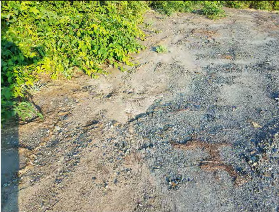
Photo 16: 07/27/2018, Watertown: Map 08, Str20 access road erosion (as shown in Photo 15), fines moving off of south corner of work pad.
