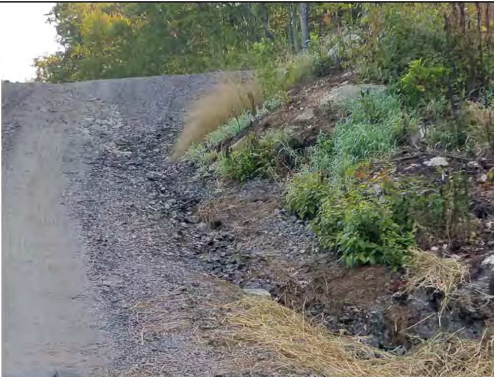
Photo 18: 07/27/2018, Watertown: Map 11, south of Str30, access road erosion immediately upland of constructed rip rap swale and sediment trap (as shown in Photo 17).
