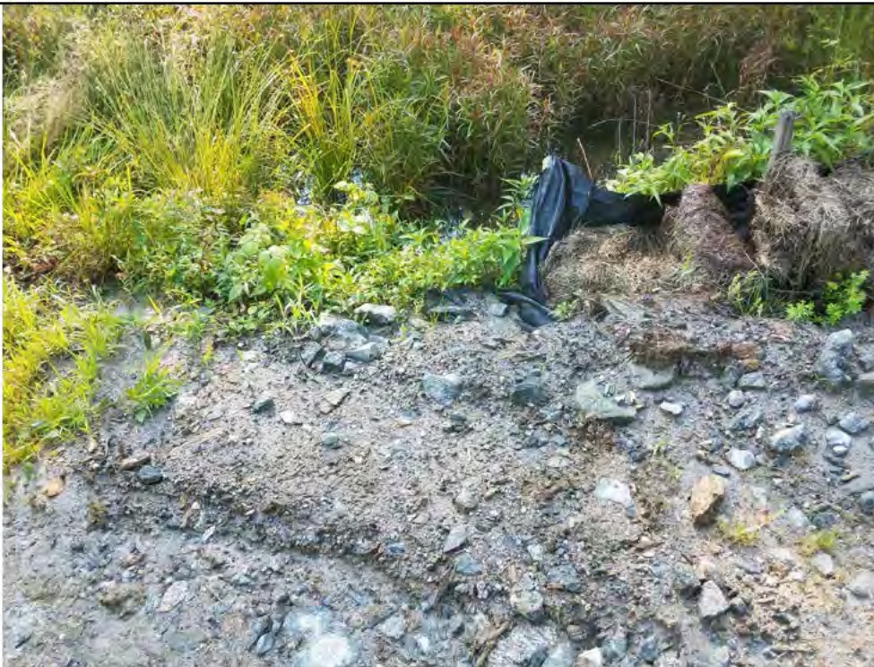
Photo 34: 07/27/2018, Watertown: Map 14, access road north of Str39 crossing wetland/vernal pool W-C20/VP-C20-1, continued movement of fine sediments during rain events impacting wetland/vernal pool. Failing E&S controls. Photo taken facing south into the wetland/vernal pool from the access road.
