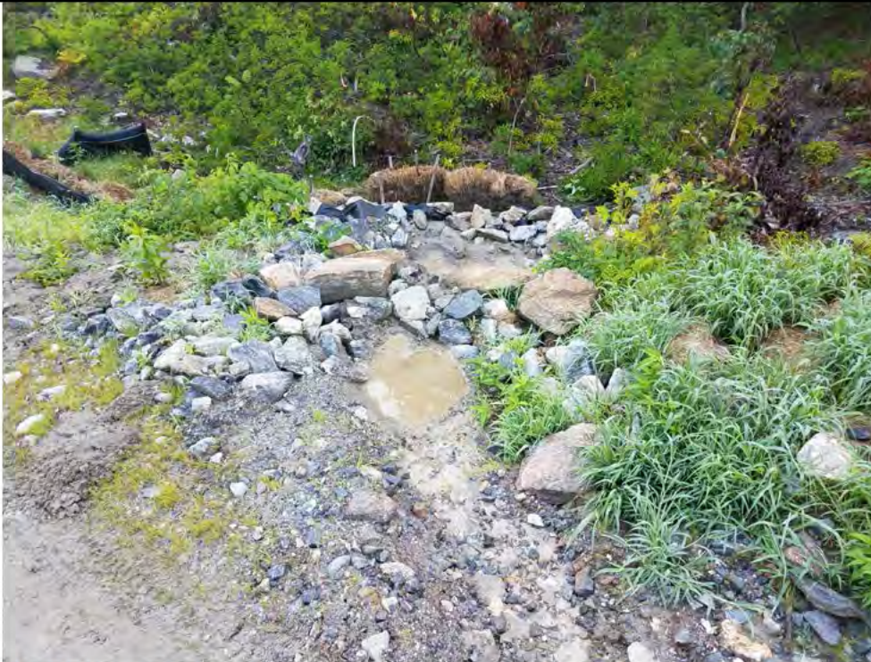
Photo 21: 07/27/2018, Watertown: Map 12, access road between Str34 and Str35, water bar and sediment trap, overloaded with fines, failing silt fence and degraded straw bales, sediments breaking through and moving toward wetland W-C15. See Photo 22 for additional view.
