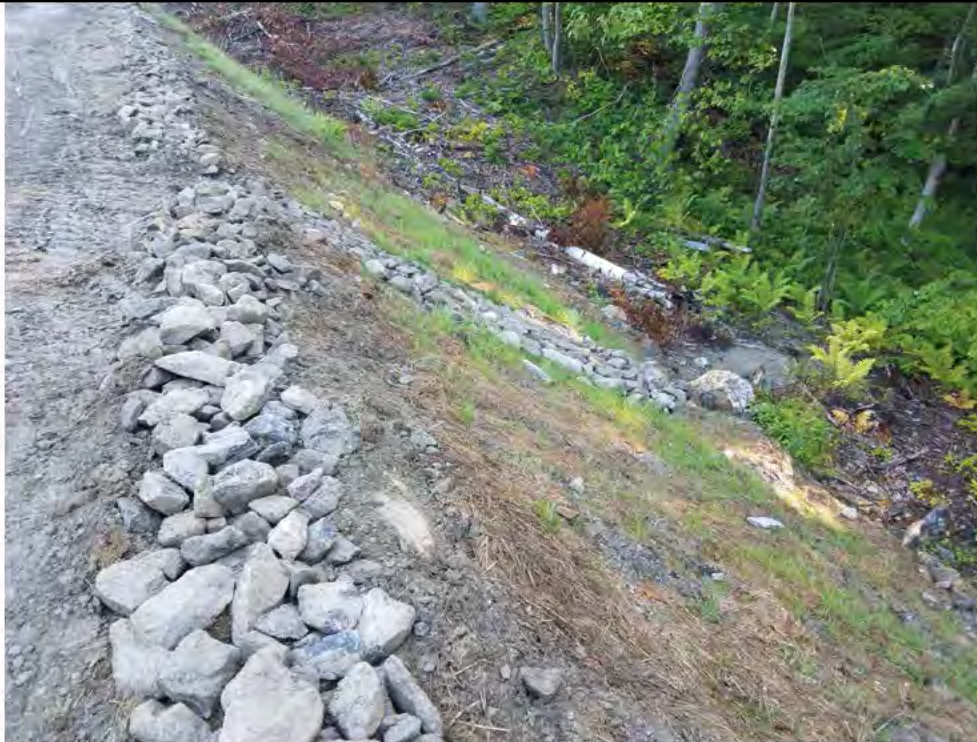
Photo 19: 07/27/2018, Watertown: Map 12, Str33 pad and slope, rip rap berm and leak offs constructed along east side of work pad. Washed out sediments observed off of the pad/slope. See Photo 20 for additional view.
