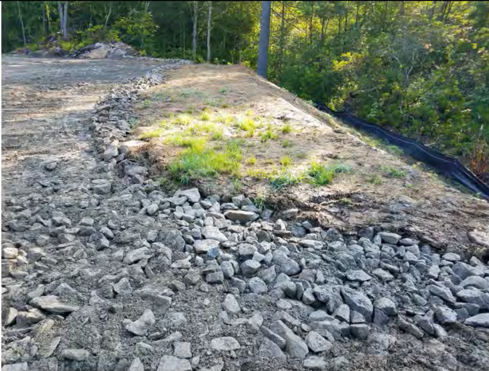
Photo 26: 07/27/2018, Watertown: Map 12, Str35 rip rap berm and swale constructed along south edge of work pad. Photo taken facing northeast. Area appeared to have performed properly during heavy rainfall events.
