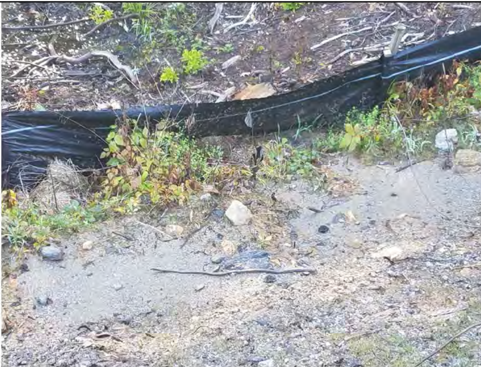
Photo 30: 07/27/2018, Watertown: Map 14, Str39, continued erosion of east slope abutting wetland/vernal pool W-C20/VP-C20-1. Sediment buildup at toe of slope against silt fence abutting wetland/vernal pool.
