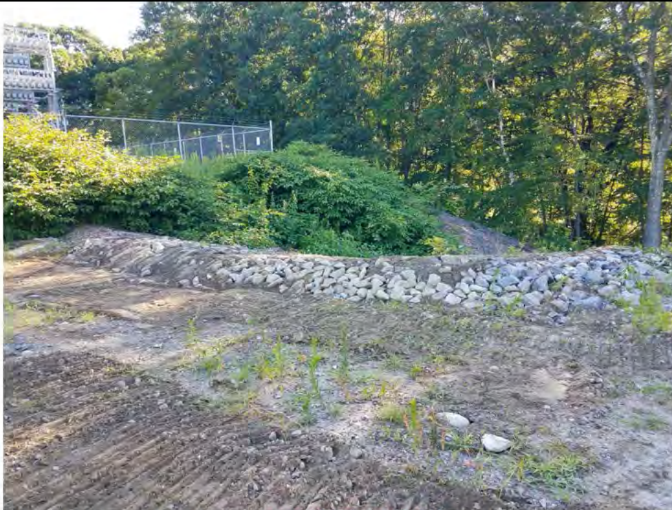
Photo 1B: 07/20/2018, Watertown: Map 01, Str1A, CORRECTIVE ACTION - Constructed berm at edge of pad upland of slope erosion area shown in Photos 1 and 1A.
