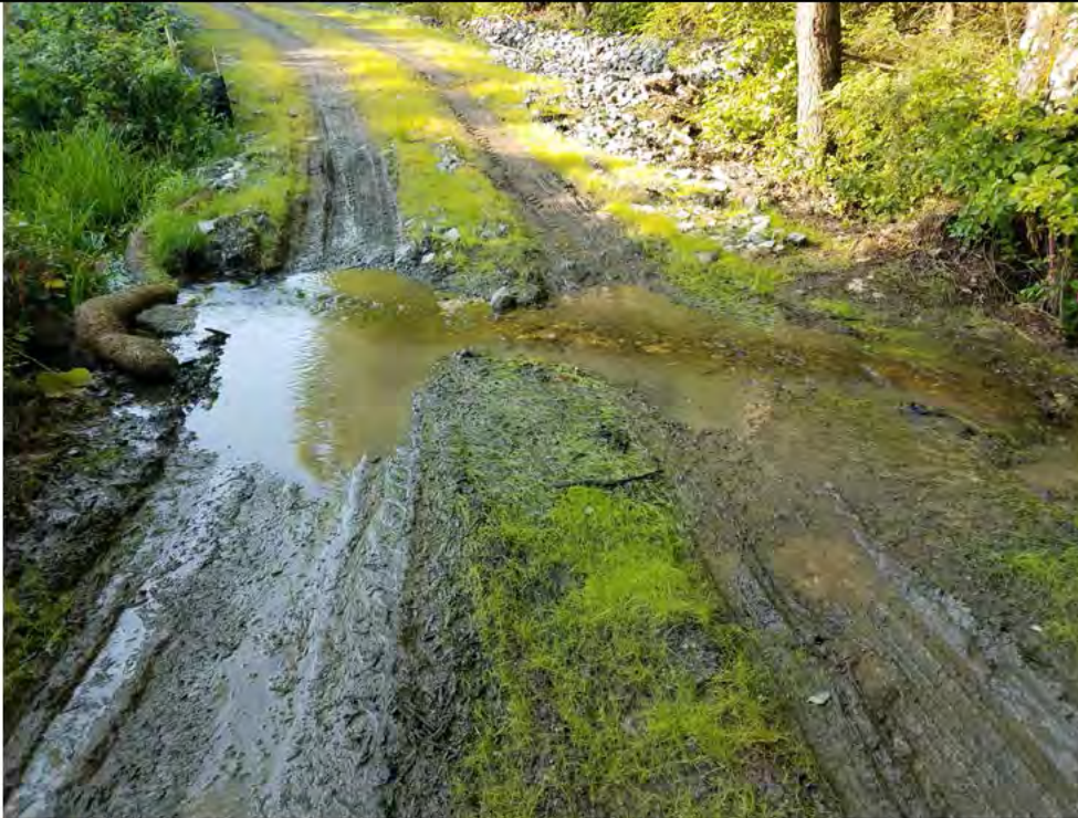
Photo 24: 07/27/2018, Watertown: Map 12, access road between Str34 and Str35 at watercourse/wetland S-C4/W-C15, muddy conditions, turbidity at crossing.
