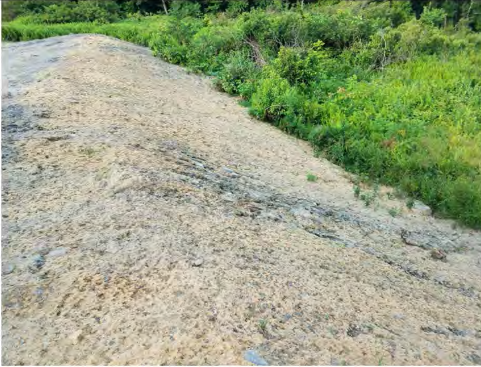
Photo 2: Interim Report # 42, Photo 6: 07/06/2018, Watertown: Map 03, Str07 pad and slope erosion, hydro seed application last fall, no visible growth. Photo taken facing east off of the south slope of pad. SEE PHOTOS 2A, 2B, 2C, and 2D FOR CORRECTIVE ACTIONS, PERMANENT BMPs.
