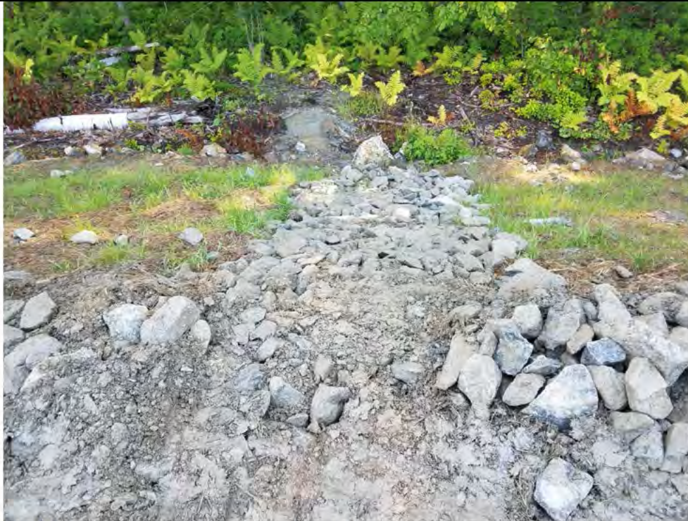
Photo 20: 07/27/2018, Watertown: Map 12, Str33 pad and slope, rip rap berm and leak offs constructed. Stone dust and fines washed out of the rip rap and travelled off the pad. No impacts to wetlands or watercourse in this area.
