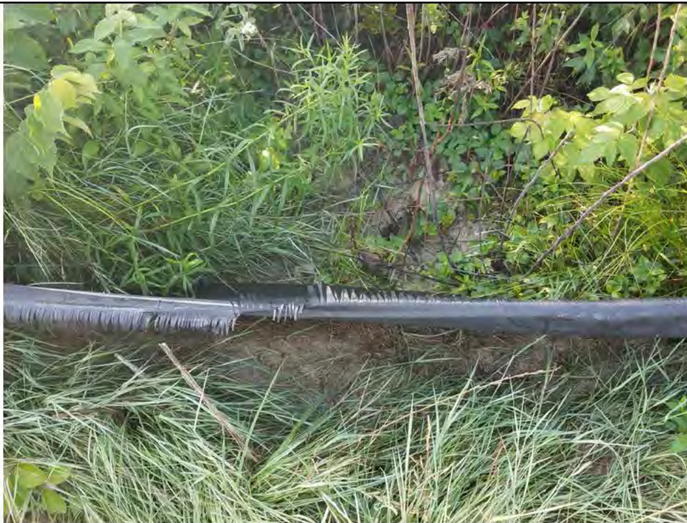
Photo 10: 07/27/2018, Watertown: Map 07, Str18, failing E&S and sediments passing under/through silt fence near or into wetland W-B6. Silt fence maintenance needed per the BMPs. Photo taken facing southeast.
