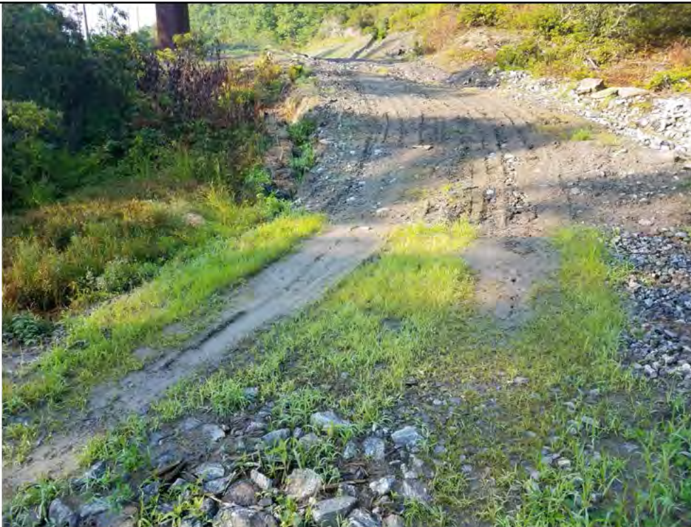
Photo 32: 07/27/2018, Watertown: Map 14, access road north of Str39 crossing wetland/vernal pool W-C20/VP-C20-1, continued movement of fine sediments during rain events impacting wetland/vernal pool. Photo taken facing southwest.
