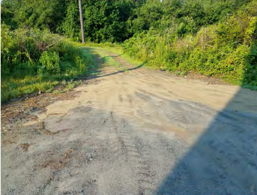
Photo 15: 07/27/2018, Watertown: Map 08, Str20 access road erosion onto the work pad and off of the south corner of the pad (see Photo 16).
