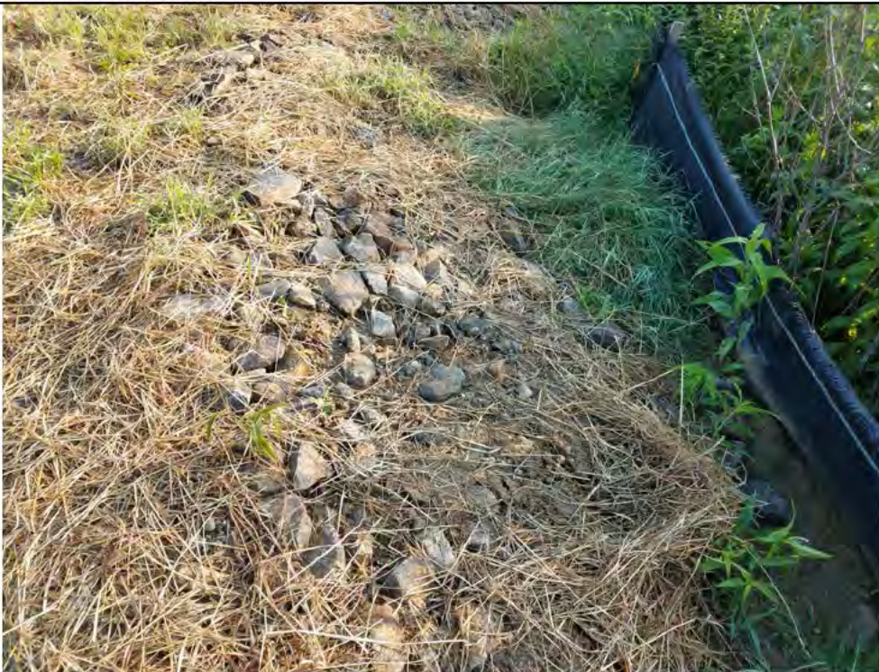
Photo 12: 07/27/2018, Watertown: Map 07, Str18 work pad and slope, close up view of area as shown in Photo 11.
