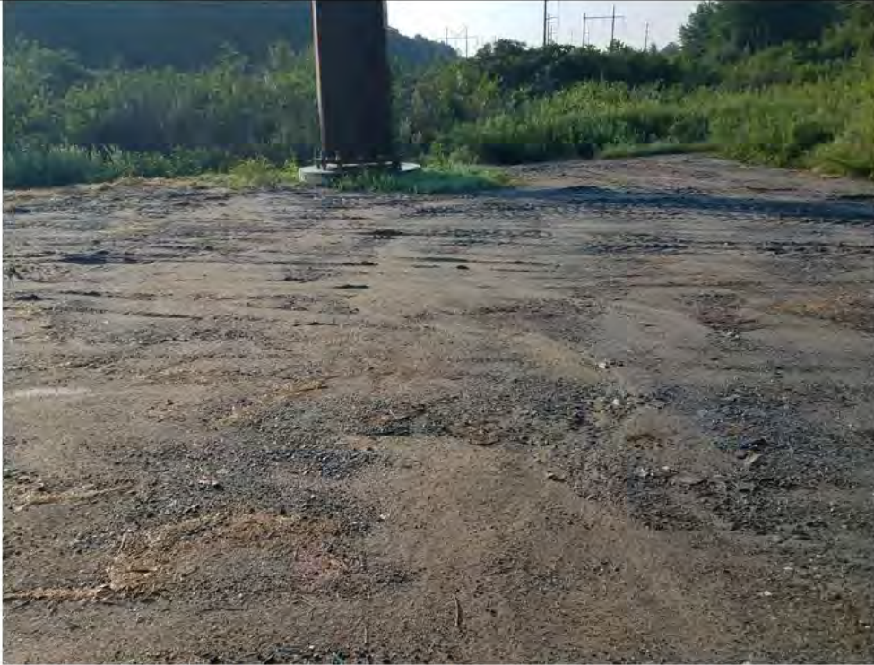
Photo 7: 07/27/2018, Watertown: Map 07, Str18 work pad, fine sediments continue to wash out of exposed non-stabilized/non-vegetated soils during rain events. Sediments are moving to the southeast toward the abutting wetland (W-B6). Photo taken facing southeast. Photos 8-12 are additional views of conditions at Str18.
