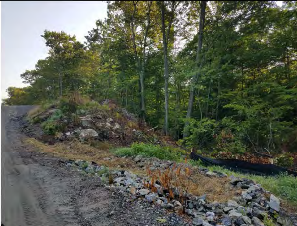
Photo 17: 07/27/2018, Watertown: Map 11, south of Str30, access road erosion into constructed rip rap swale and sediment trap. Photo taken facing north toward Str30. See Photo 18 for additional view.
