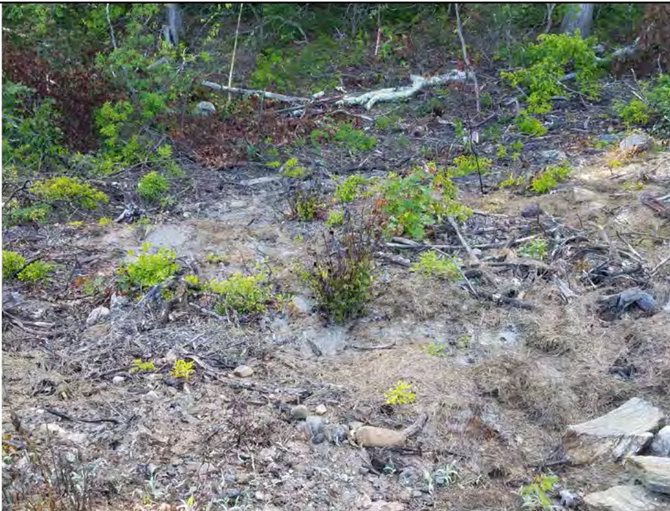
Photo 28: 07/27/2018, Watertown: Map 13, Str38, continued erosion of north slope with buildup of sediments at toe of slope.
