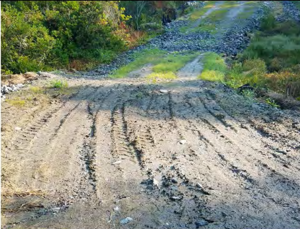
Photo 31: 07/27/2018, Watertown: Map 14, access road north of Str39 crossing wetland/vernal pool W-C20/VP-C20-1, continued movement of fine during rain events impacting wetland/vernal pool. Photo taken facing northeast. See Photos 32, 33, and 34 for additional views of conditions in this area.
