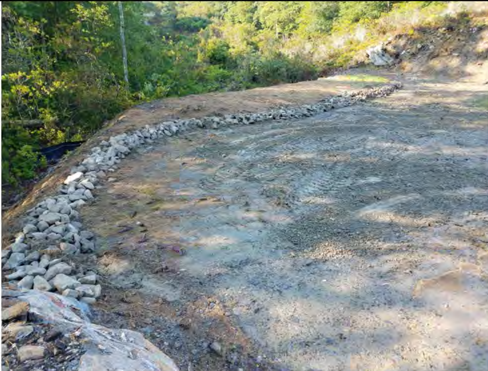
Photo 25: 07/27/2018, Watertown: Map 12, Str35, Permanent BMPs installed at this location. BluRoc constructed a rip rap berm and swale along the south edge of work pad to help prevent slope erosion. See Photo 26 for additional view.
