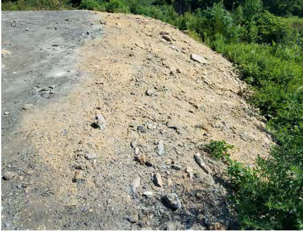
Photo 22: 07/13/2018, Watertown: Map 04, Str05 slope stabilization. Hydro seed applied to the down gradient slope.
