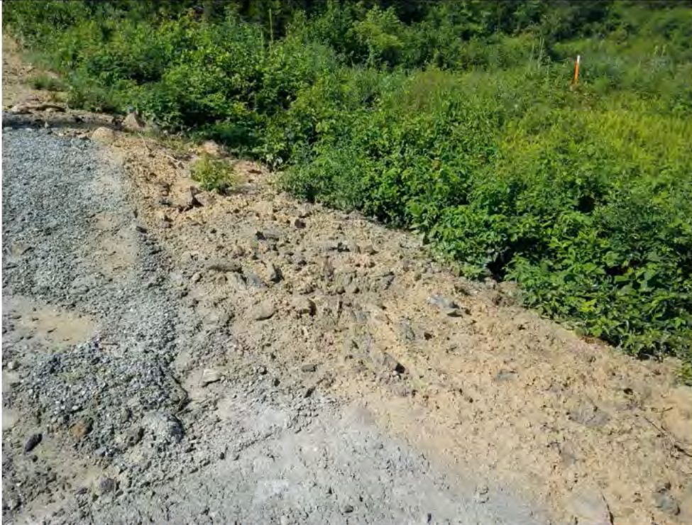
Photo 24: 07/13/2018, Watertown: Map 04, Str05 slope stabilization. Hydro seed applied to the pad slope, erosion area shown previously in Photo #4. Photo taken facing northwest.
