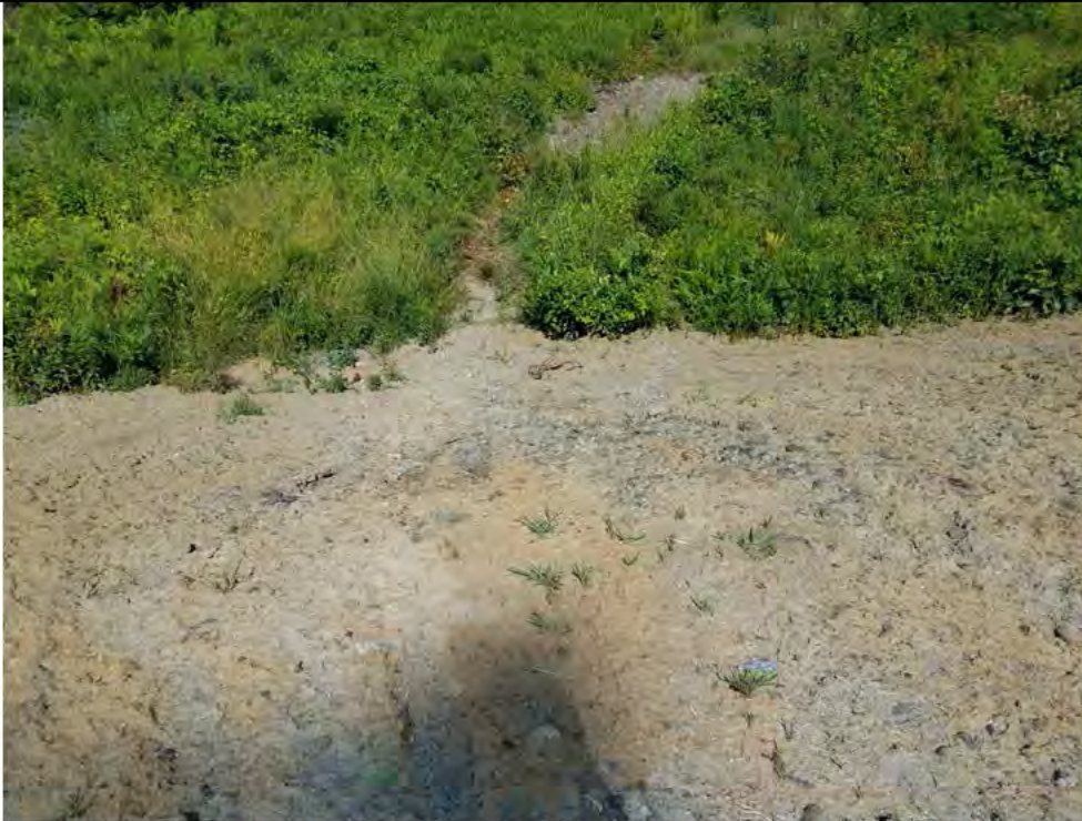
Photo 29: 07/13/2018, Watertown: Map 03, Str07 slope stabilization. Hydro seed applied to the pad slope, erosion area shown previously in Photo #6. Photo taken north off of the top of the work pad.
