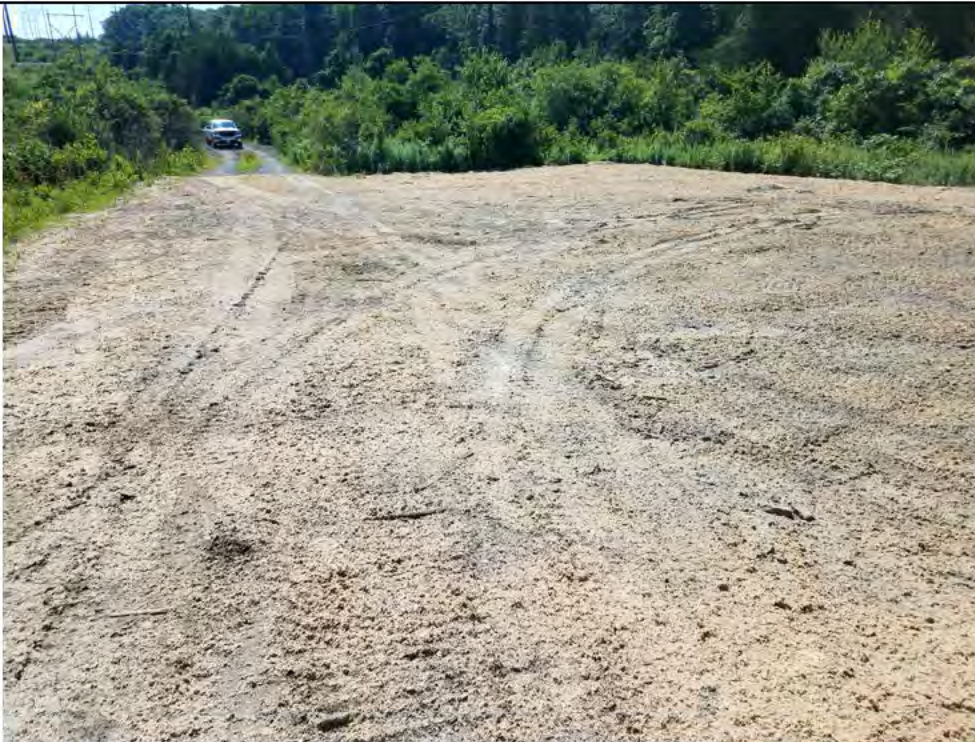
Photo 27: 07/13/2018, Watertown: Map 04, Str09, work pad and access hydro seeded. Area previously shown in Photo #10. Photo taken facing east.
