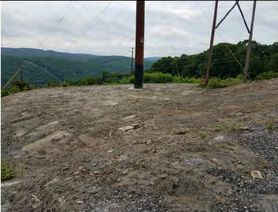
Photo 3: 07/06/2018, Watertown: Map 04, Str05 slope erosion, fine sediments continue to wash out of exposed, unstabilized/unvegetated soils during rain events. Photo taken facing north.
