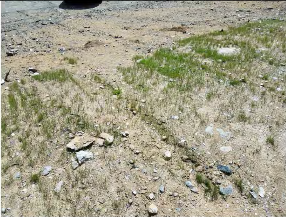
Photo 31: 07/13/2018, Litchfield: Map 29, Str83, upland slope facing down to the Str83 work pad, minimal vegetation growth from previous stabilization measures, erosion visible. Area previously shown in Photo 16. Photo taken facing east, down the upland slope.
