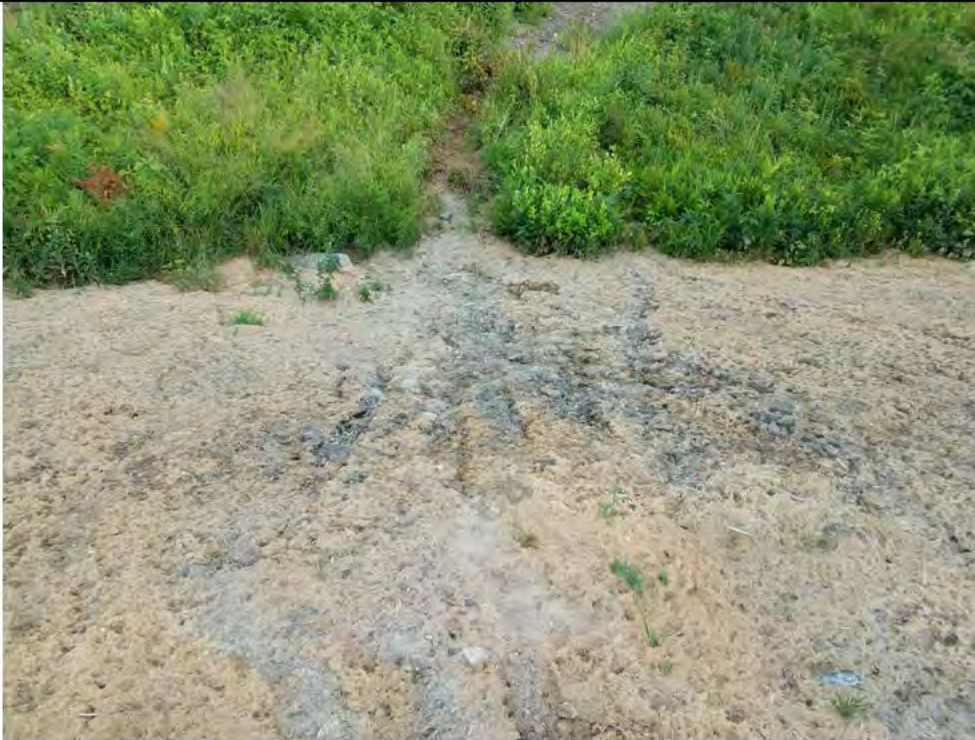
Photo 4: 07/06/2018, Watertown: Map 03, Str05 slope erosion, no stabilization. Photo taken facing north.
