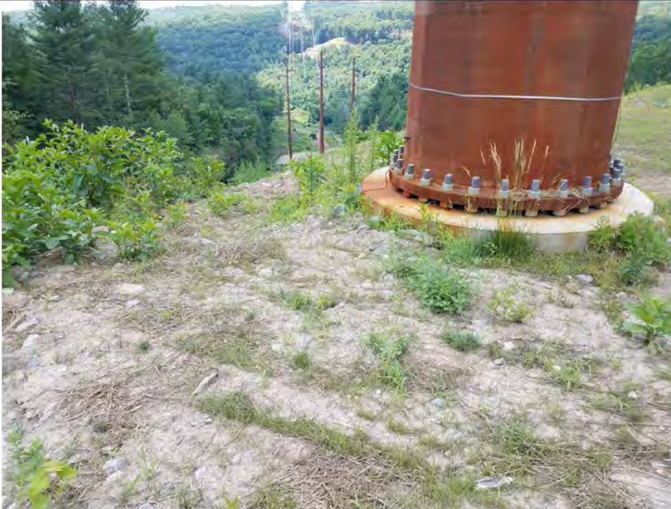
Photo 34: 07/13/2018, Harwinton: Map 32, Str88 work pad, visible erosion occurring on pad and down north slope. Light vegetation growth from previous stabilization measures.
