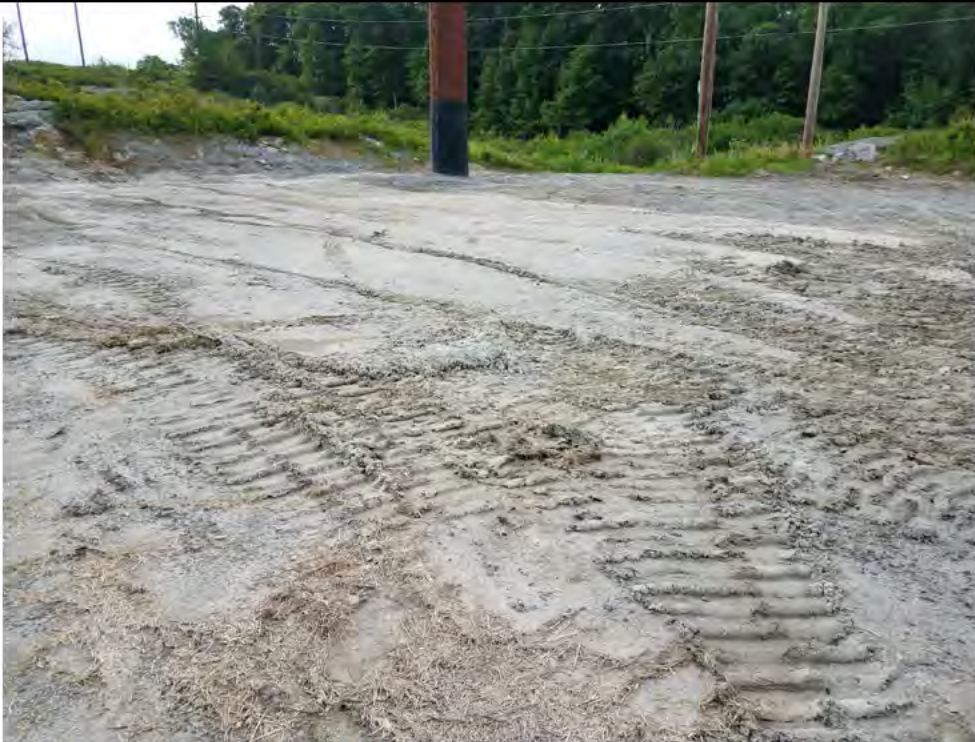
Photo 5: 07/06/2018, Watertown: Map 03, Str07, fine sediments continue to wash out of exposed, unstabilized/unvegetated soils during rain events. Photo taken facing northeast.
