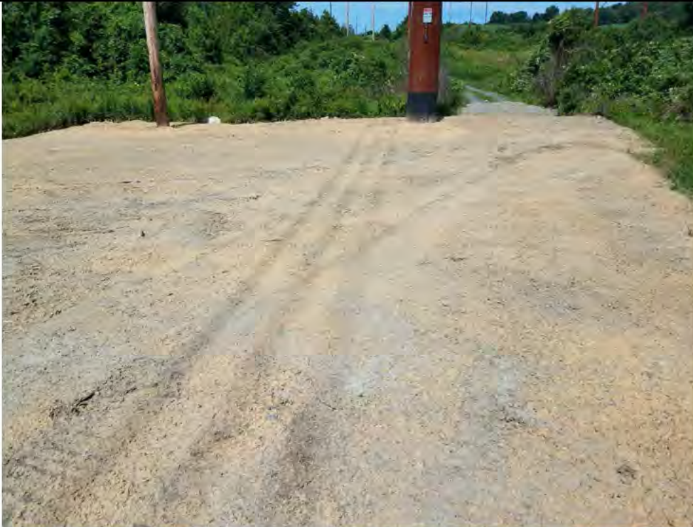
Photo 26: 07/13/2018, Watertown: Map 04, Str09, work pad and access hydro seeded. Area previously shown in Photo #9. Photo taken facing west toward S-A5.
