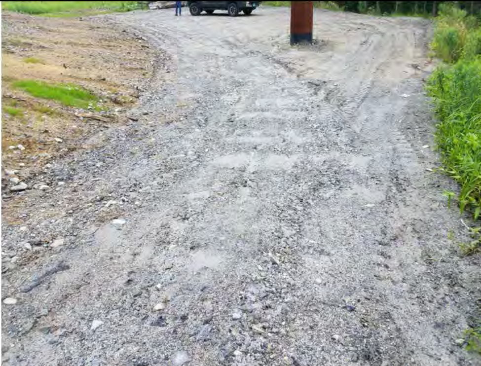
Photo 17: 07/06/2018, Litchfield: Map 29, Str83, fine sediments continue to wash out of exposed, unstabilized/unvegetated soils during rain events and access road erosion due to uncontrolled surface water flow from upland areas. Photo taken facing east.
