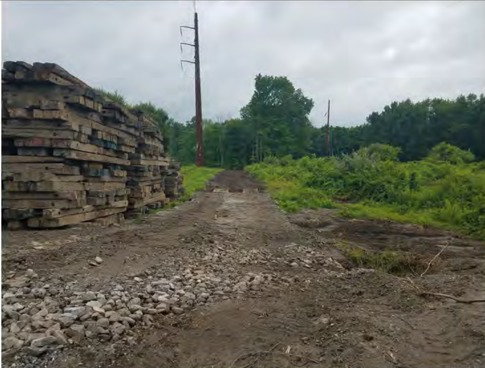
Photo 13: 07/06/2018, Thomaston: Map 22, Str63-Str64 timber mats being removed. Photo taken facing north from Walnut Hill Road access.
