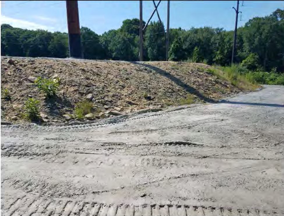
Photo 25: 07/13/2018, Watertown: Map 04, Str08, slope stabilization. Hydro seed applied to the pad slope, erosion area shown previously in Photo #8.
