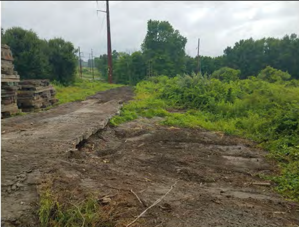
Photo 14: 07/06/2018, Thomaston: Map 22, Str63-Str64 timber mats being removed. Photo taken facing north from Walnut Hill Road access.
