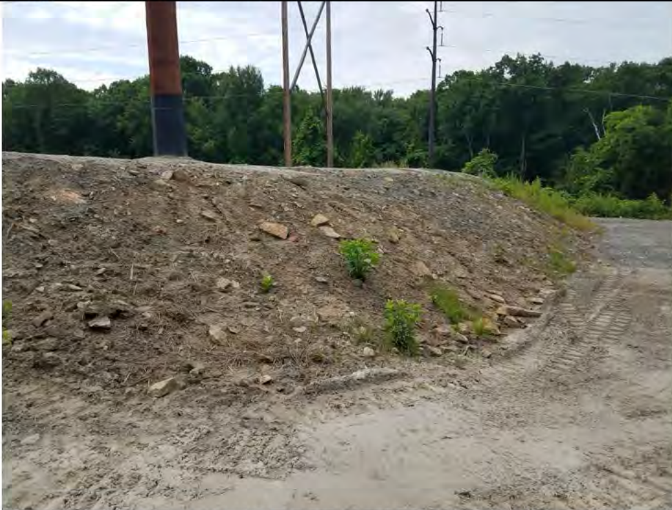
Photo 8: 07/06/2018, Watertown: Map 04, Str08, slope erosion, no stabilization. Photo taken facing northwest.
