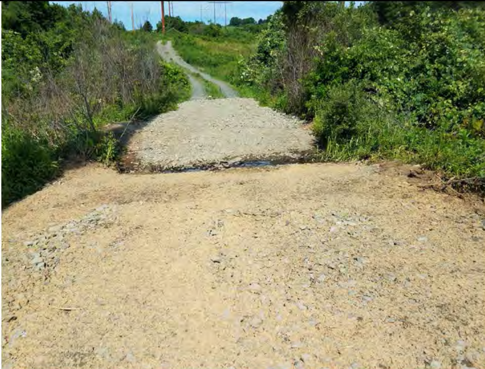
Photo 28: 07/13/2018, Watertown: Map 04, Str09 and S-A5, timber mat crossing removed, access road hydro seeded, stream crossing graded and improved. Photo taken facing west toward S-A5 from west end of Str09.
