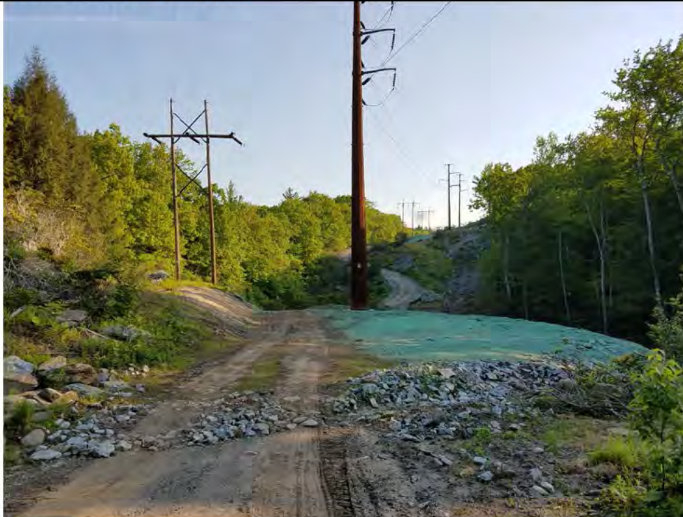
Photo 2: 05/25/2018, Watertown: Map 14, Str39, pad stabilization measures (graded and hydro seeded). Photo taken facing north along the access road and work pad.
