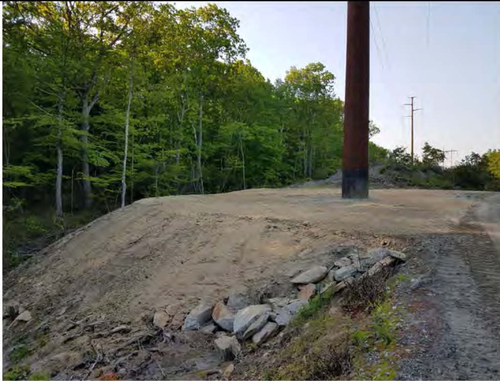
Photo 1: 05/25/2018, Watertown: Map 13, Str38, pad stabilization measures (graded and hydro seeded). Photo taken facing south along the access road and work pad.
