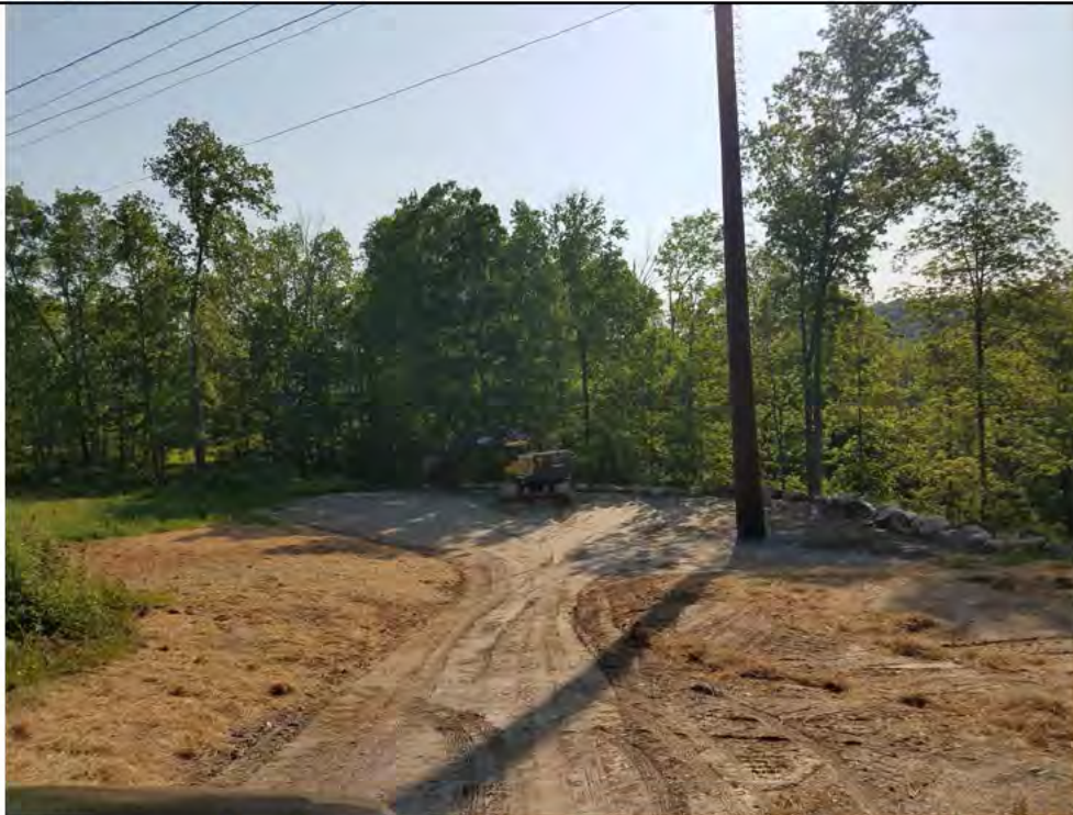
Photo 6: 05/25/2018, Watertown: Map 23, Str65, pad stabilization measures in progress. Photo taken facing east along the access road and work pad.
