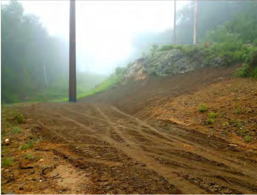
Photo 7: 06/01/2018, Thomaston: Map 21, Str60, grade at base of rock outcrop raised approximately 8 to 10 feet (up from top grade of structure base) and gently sloped away from the rock face to match surrounding slope and grades.
