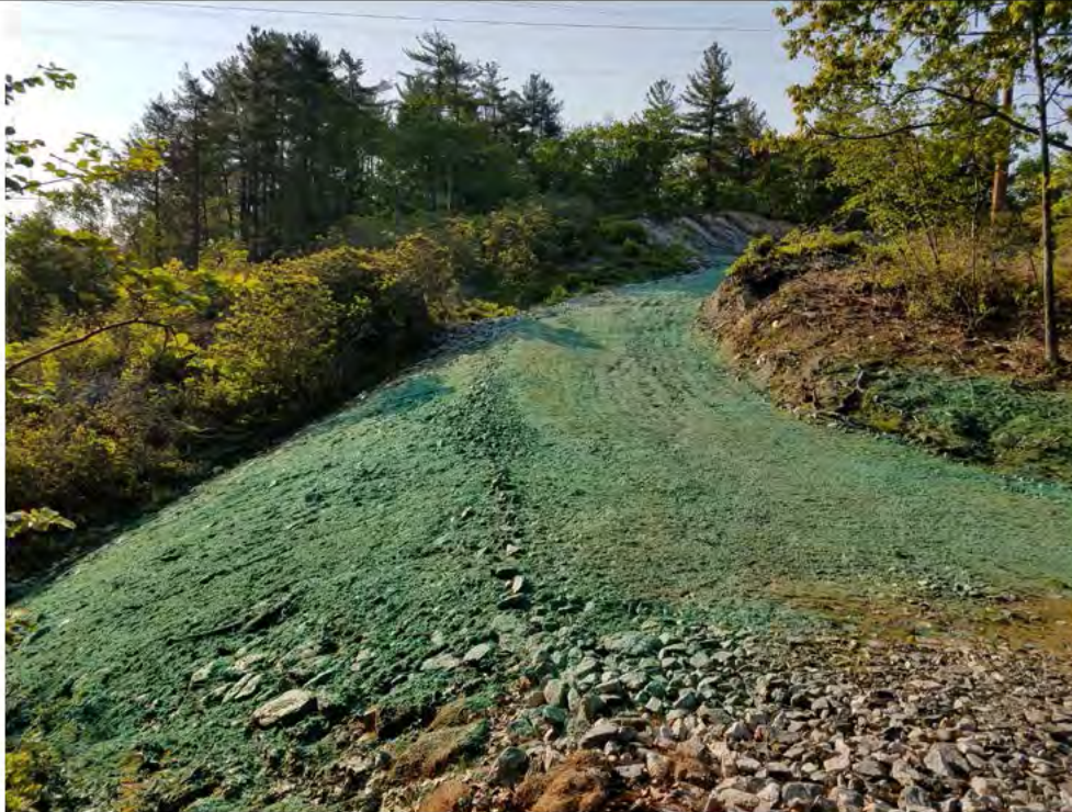
Photo 3: 05/25/2018, Watertown: Map 14, Str41, pad stabilization measures (graded and hydro seeded). Photo taken facing east along the access road to the work pad upland.
