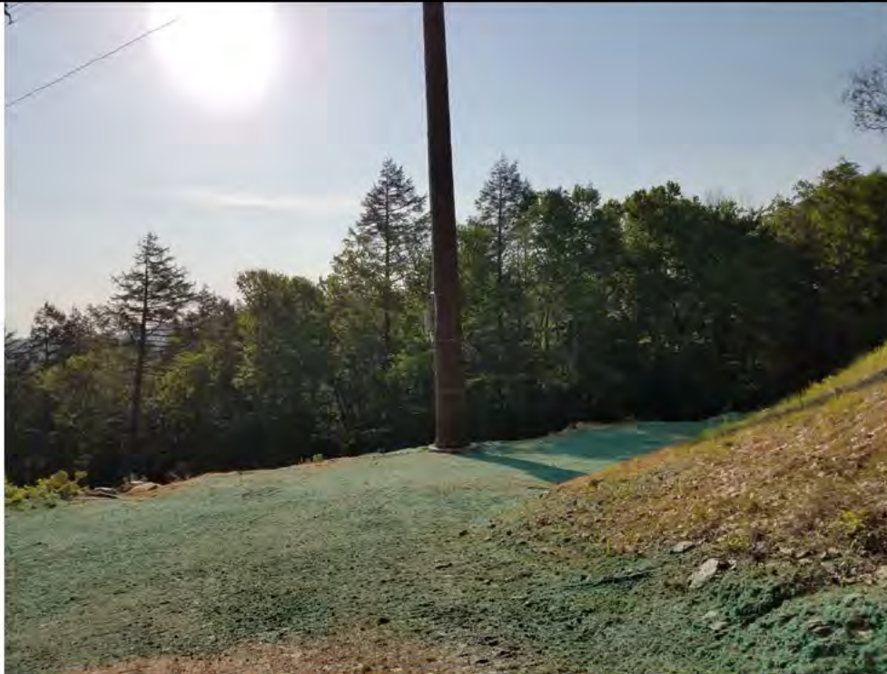
Photo 5: 05/25/2018, Watertown: Map 16, Str46, pad stabilization measures (graded and hydro seeded). Photo taken facing south along the access road and work pad.
