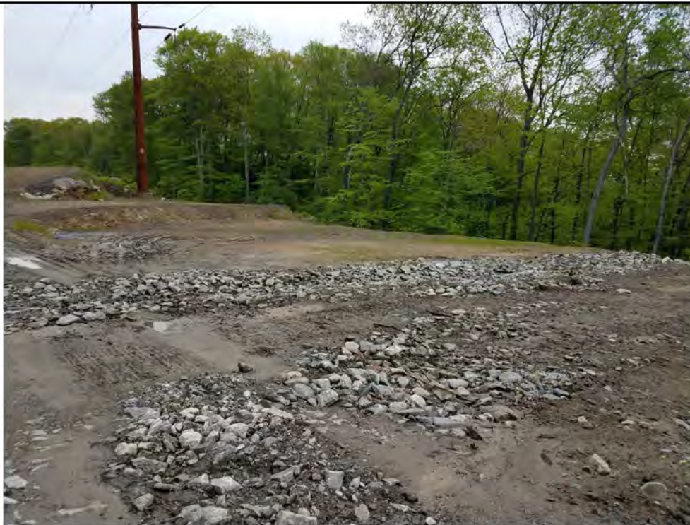
Photo 2: 05/18/2018, Watertown: Map 10, combined work pads Str27-Str28, area regraded and the rock filled swale reconstructed. Photo taken facing north along the access road, Str28 in the distance.
