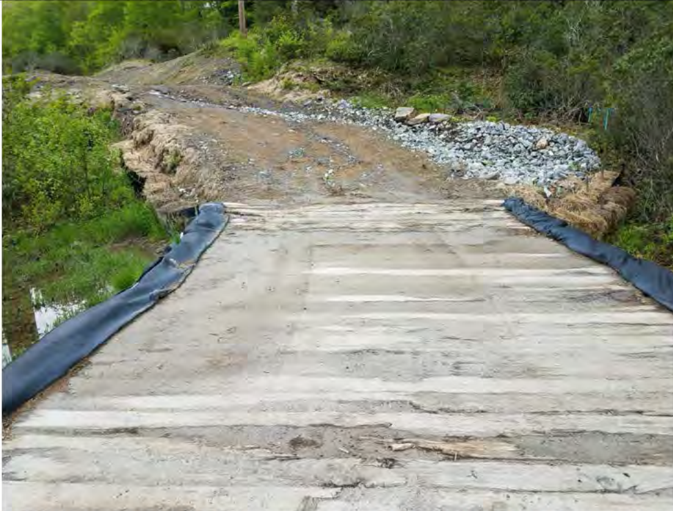
Photo 15: 05/18/2018, Watertown: Map 14, timber mat crossing at W-C20/VP-C20-1, access road erosion, water bar failure, heavy sedimentation on timber mats, and visible impacts to surrounding area (w-C20/VP-C20-1). Photo taken facing south toward Str39.
