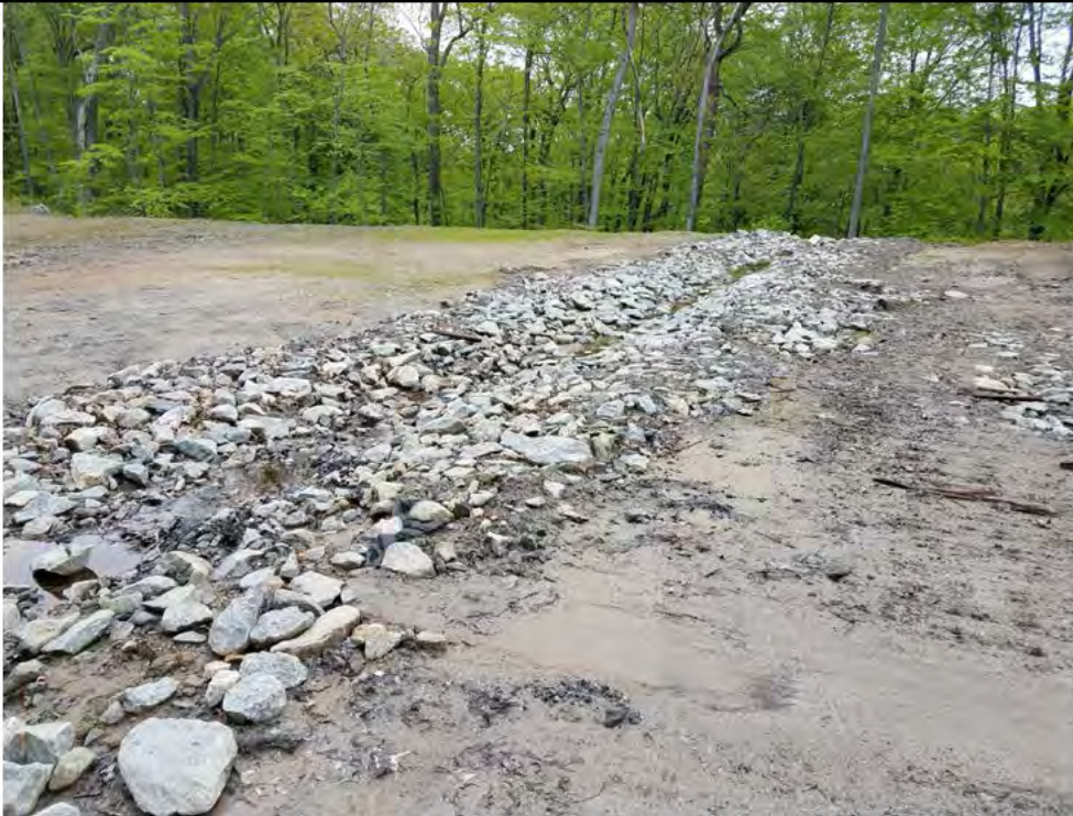
Photo 3: 05/18/2018, Watertown: Map 10, combined work pads Str27-Str28, area has been regraded and the rock filled swale reconstructed. Photo taken facing east across the pad.
