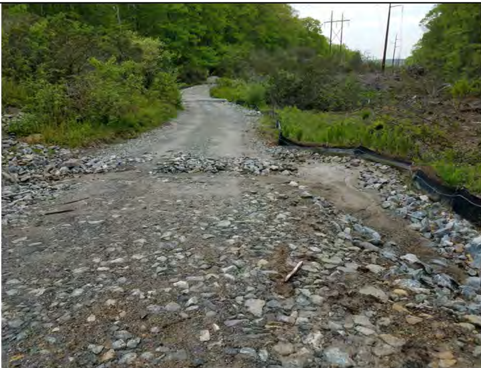
Photo 6: 05/18/2018, Watertown: Map 11, north of Str32 sediment trap filled to capacity, failing silt fence and degraded hay bales, stone filled water bar packed with sediment. Photo taken facing north along the access road in the direction of Str33.
