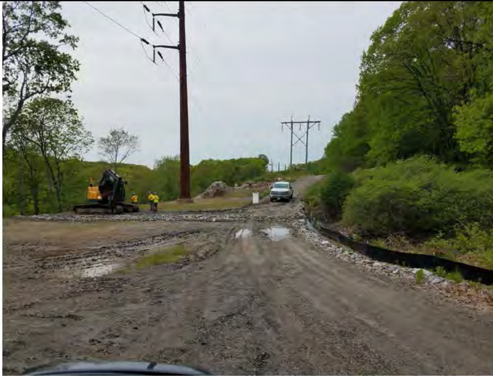
Photo 1: 05/18/2018, Watertown: Map 10, combined work pads Str27-Str28, BluRoc setting up to resume stabilization/restoration work. Photo taken facing south along the access road, Str27 in the distance.
