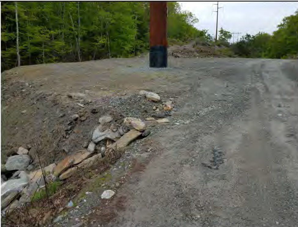
Photo 14: 05/18/2018, Watertown: Map 13, northwest corner of the Str38 work pad, pad and slope erosion, pad stabilization measures (seeded last fall) failed. Photo taken facing south along the access road and work pad.
