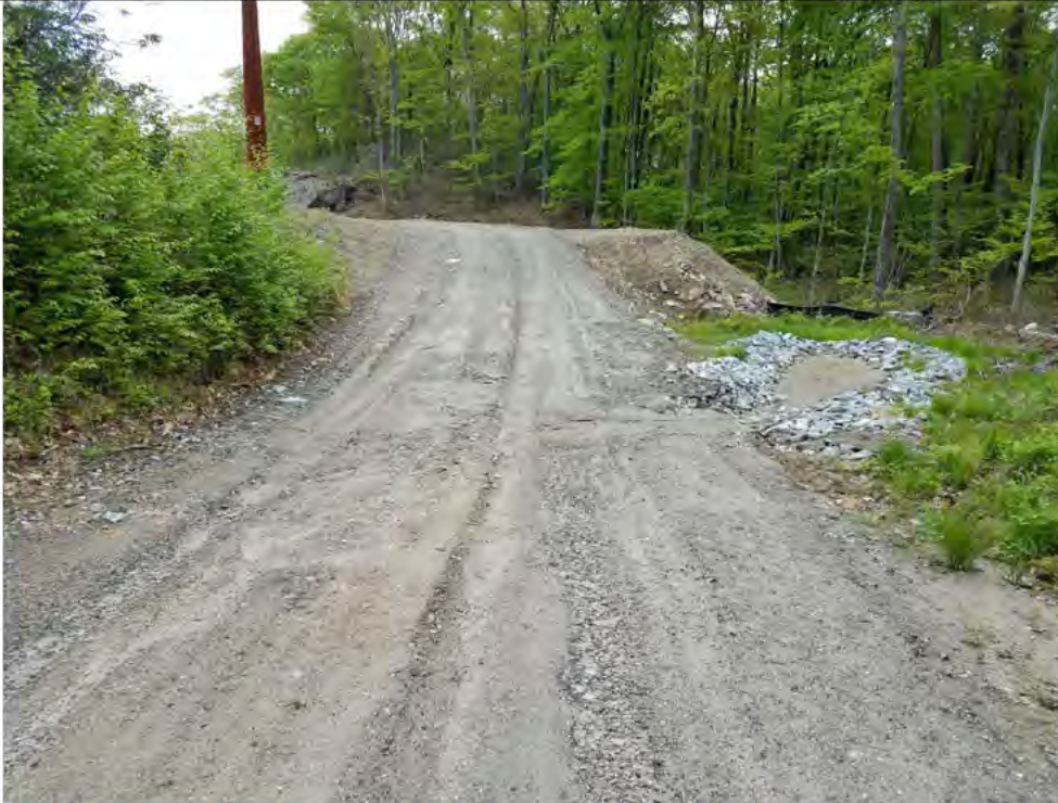
Photo 7: 05/18/2018, Watertown: Map 12, south of Str33 sediment trap filled to capacity and visible access road erosion (rills). Photo taken facing north along the access road, Str33 in the distance.
