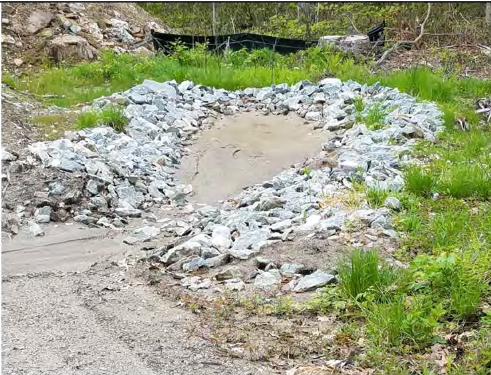
Photo 8: 05/18/2018, Watertown: Map 12, south of Str33 sediment trap filled to capacity. Photo taken facing east along the east side of the access road to Str33.
