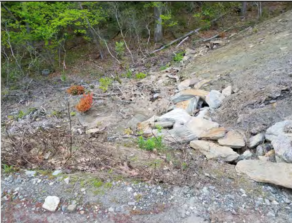
Photo 12: 05/18/2018, Watertown: Map 13, northwest corner of the Str38 work pad, pad and slope erosion. Photo taken facing northeast off the access road and down the pad slope.
