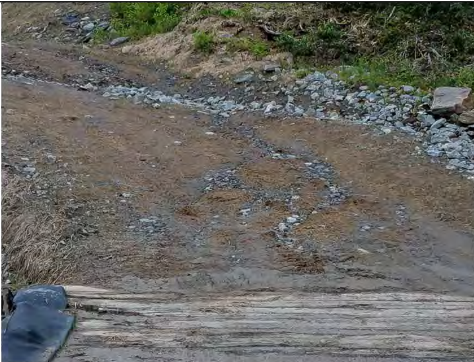
Photo 16: 05/18/2018, Watertown: Map 14, south of timber mat crossing at W-C20/VP-C20-1, access road erosion, water bar failure, causing heavy sedimentation on timber mats, and visible impacts to surrounding area (w-C20/VP-C20-1). Stabilization measures were in place last fall but were not maintained throughout the winter months.
