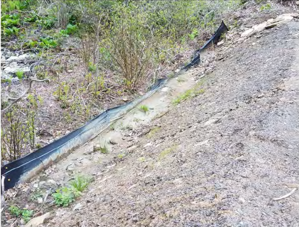
Photo 9: 05/18/2018, Watertown: Map 12, east side of the Str35 work pad, failing silt fence, excessive sediment buildup on silt fence, visible slope erosion (rills), and no pad stabilization measures. Photo taken facing southeast from the pad toward the abutting wetland (W-C15).
