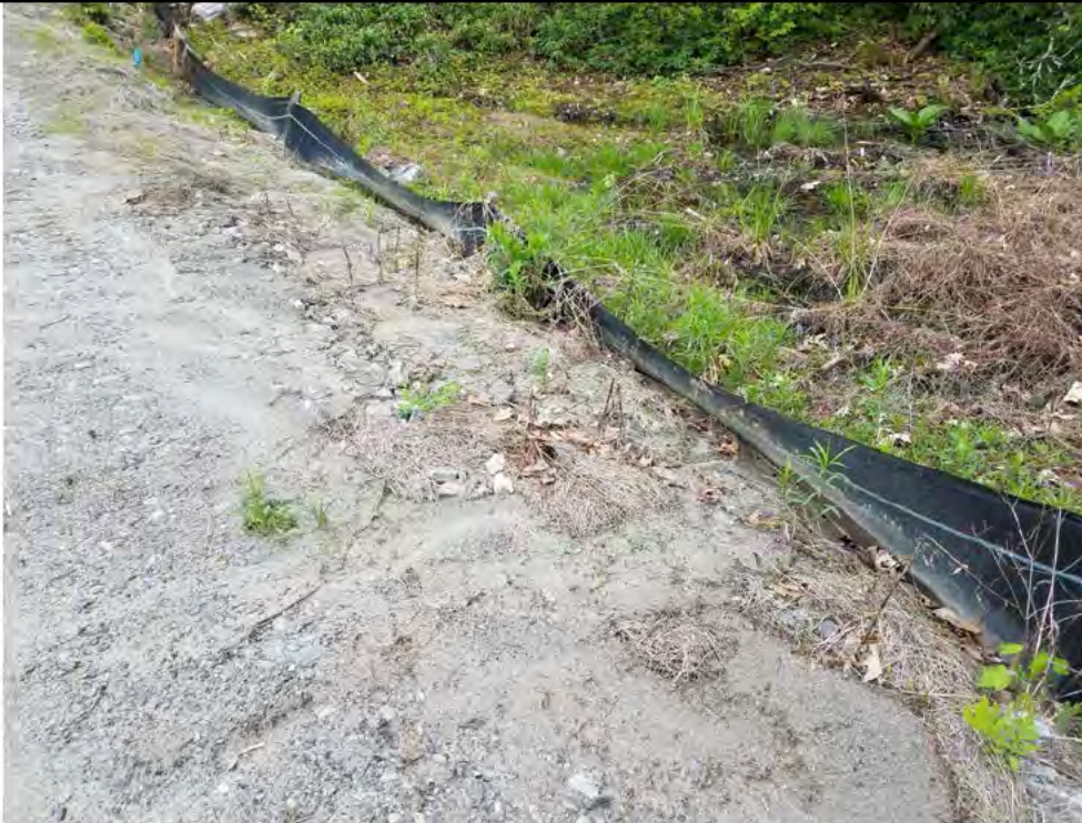
Photo 11: 05/18/2018, Watertown: Map 13, access road south of Str36, failing silt fence abutting wetland W-C15 and access road erosion. Photo taken facing east along the access road toward Wetland W-C15.
