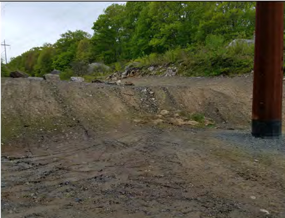
Photo 4: 05/18/2018, Watertown: Map 11, Str32 upland slope and pad not stabilized, visible erosion of the slope and lower pad is occurring. Photo taken facing south from the access road.
