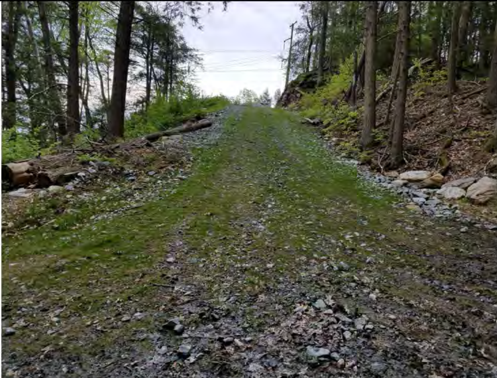
Photo 17: 05/18/2018, Watertown: Map 16, access road to Str45, stabilized last fall with hydro seed applications. Good growth at this time, no visible erosion. Photo taken facing upland, southeast toward Str45.
