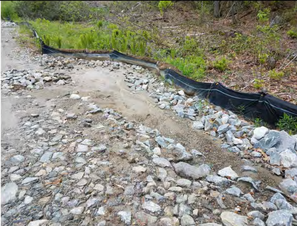
Photo 5: 05/18/2018, Watertown: Map 11, north of Str32 sediment trap filled to capacity and failing silt fence and degraded hay bales. Photo taken facing north along the east side of the access road.
