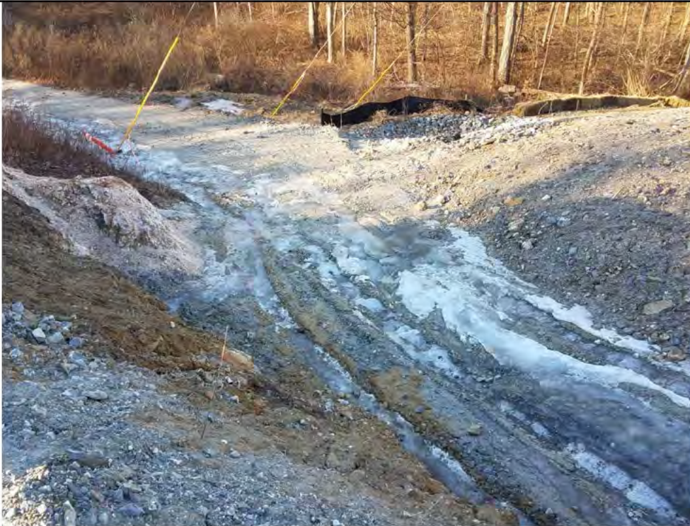
Photo 2: 01/26/2018, Litchfield: Map 26, ice sheet and visible rills on the access road below Str73 down to wetland W-E2, runoff from upland drainage and from the pad for structure Str73.
