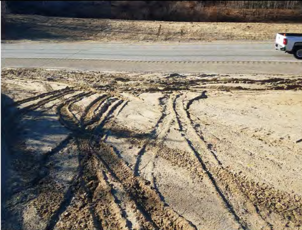
Photo 3: 01/26/2018, Litchfield: Map 31, access road to Str85 of Route 8 north, visible tire ruts and sedimentation.
