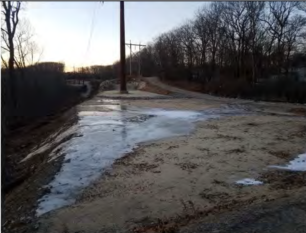
Photo 4: 01/26/2018, Watertown: Map 26, ice sheet and minor slope erosion at Str27-Str28, caused by drainage from W-C3 across the access road and over the pad for Str28. Due to surface grades the drainage is not getting to the rip rap swale that runs through the middle of the combined Str27-Str28 pad (swale can be seen in the photo in distance past the ice sheet).
