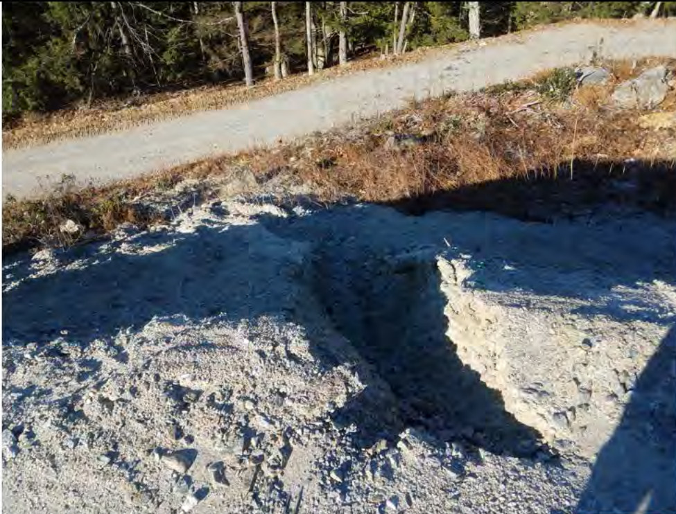
Photo 7: 01/26/2018, Litchfield: Map 30, Str85, significant rill formed and slope erosion visible, non-stabilized pad and slope.
