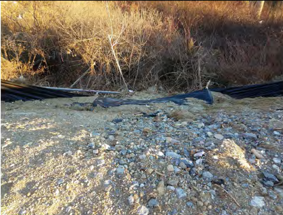
Photo 5: 01/26/2018, Watertown: Map 01, Str2 pad, failed silt fence at toe of slope abutting S-A1 and sedimentation into watercourse, non-stabilized slope and pad.
