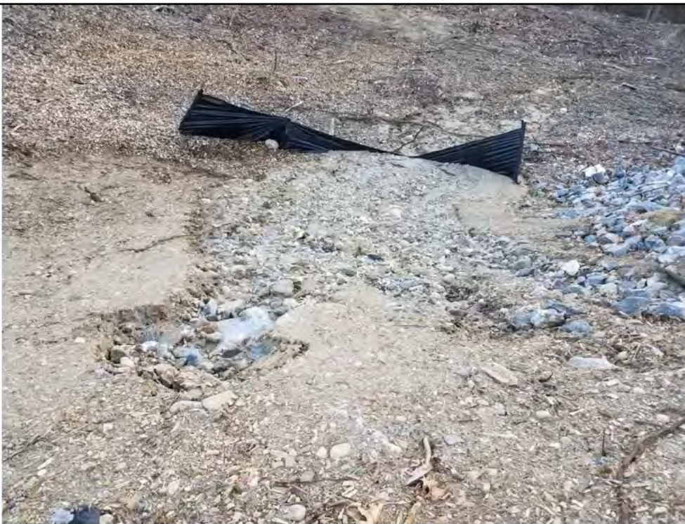
Photo 6: 01/26/2018, Watertown: Map 01, Str1A pad, failed silt fence at toe of slope, significant rills for a great distance down gradient towards Connecticut Designated Wetland Area.
