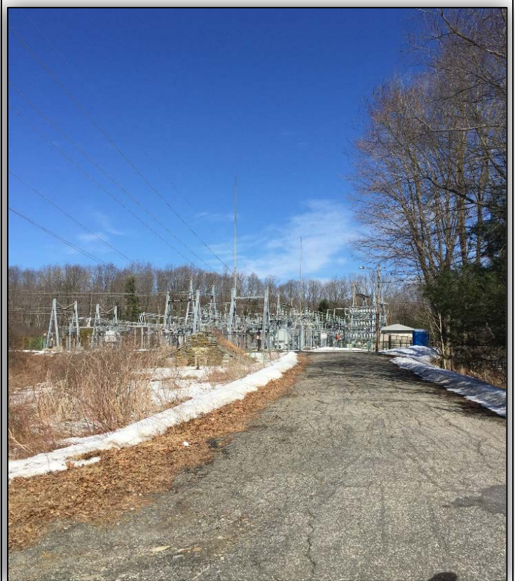
Photo 12: Campville Substation, Harwinton. View of substation, looking north from station access road off Wildcat Hill Road
