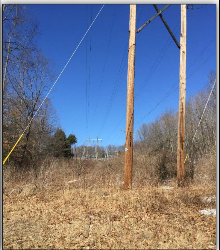
Photo 22: Wildcat Hill Road, Harwinton. View east along ROW toward Campville Substation.
