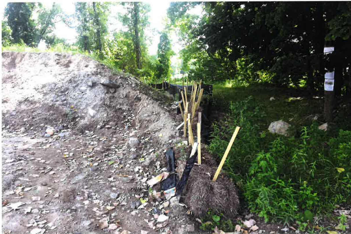
Photo 6: View of haybales added at west end of silt fence (completed CA #5) looking south.
