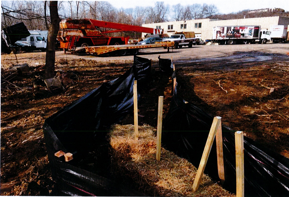
Photo 5: View of CA #4 at west end of erosion controls - complete installation of hay bales to edge of pavement, looking north. Photo taken on April 3, 2017.
