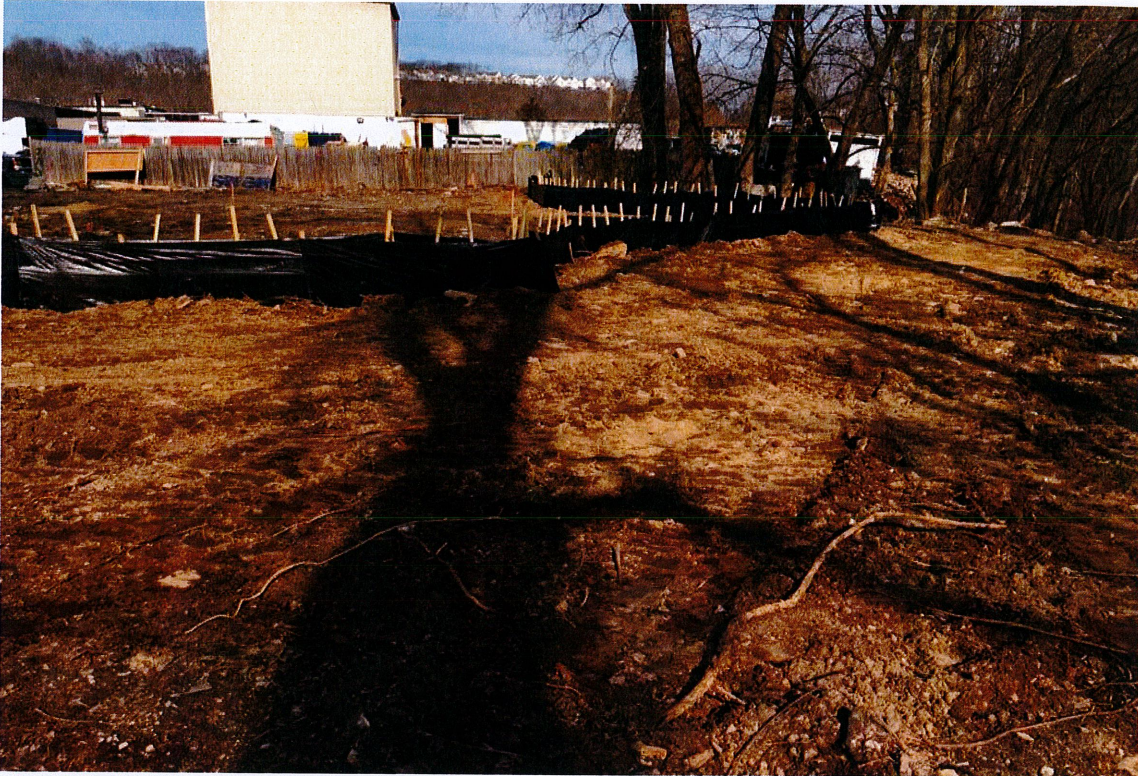
Photo 3: View of CA #3 - seed and mulch exposed soils outside of erosion controls, looking east.
