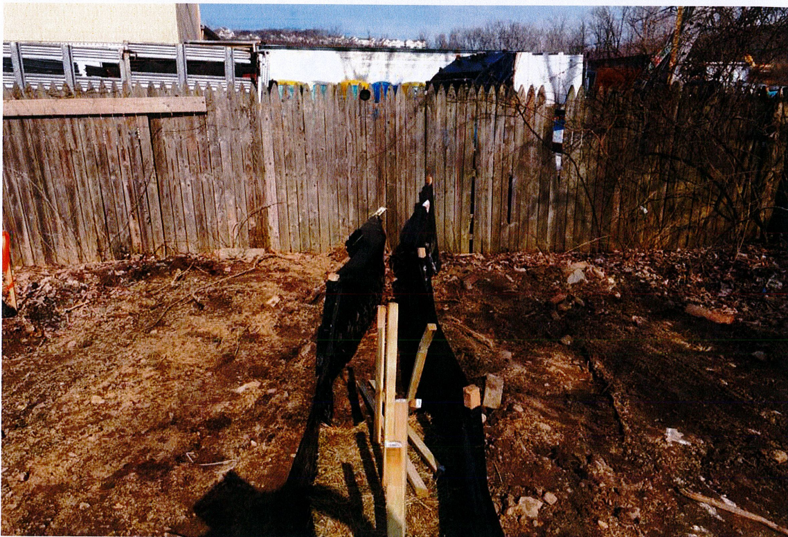
Photo 2: View of CA #2 at east end of erosion controls – complete installation of hay bales to wooden stockade fence, looking east.
