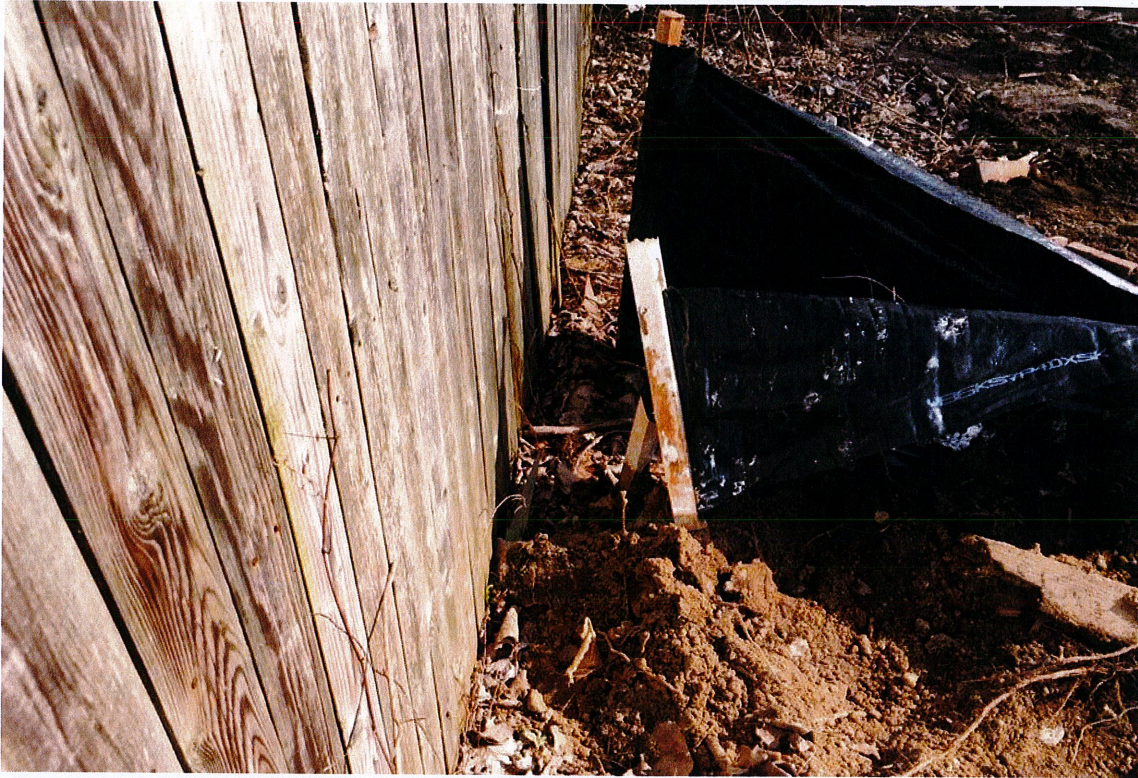
Photo 1: View of corrective action (“CA”) #1 - silt fence needs to be tight against wooden stockade fence at east end of erosion controls, looking south.
