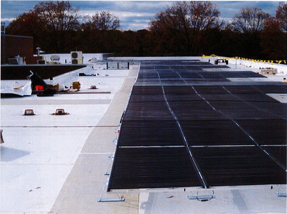
95 kW system installed at Glenville School, Greenwich CT – 2009-10
