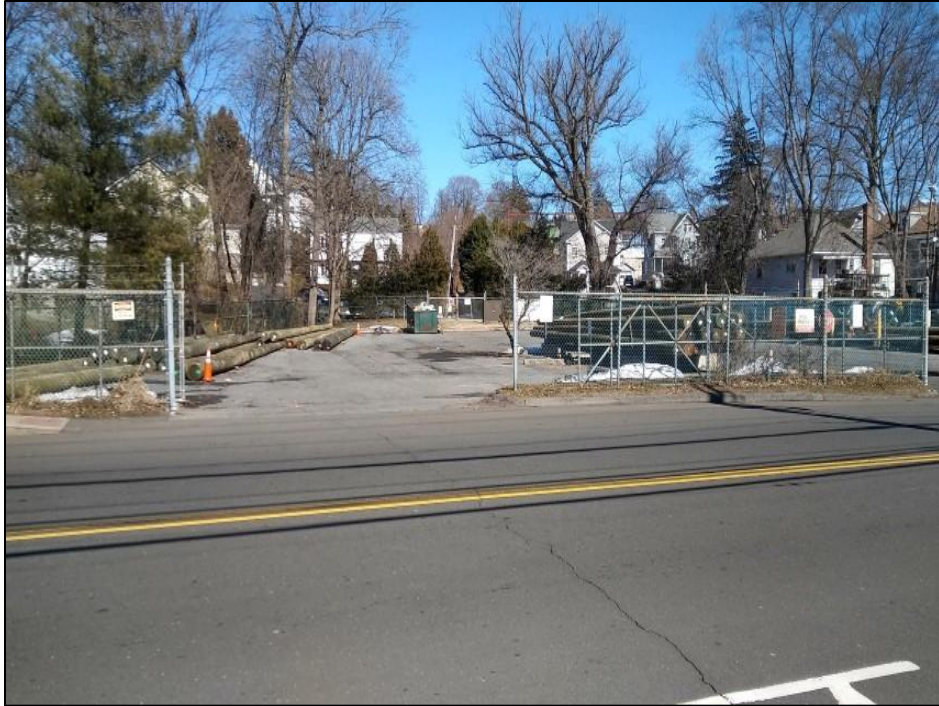
Photo 1. Overview photo of the proposed Greenwich Substation location at 281 Railroad Avenue facing north.
