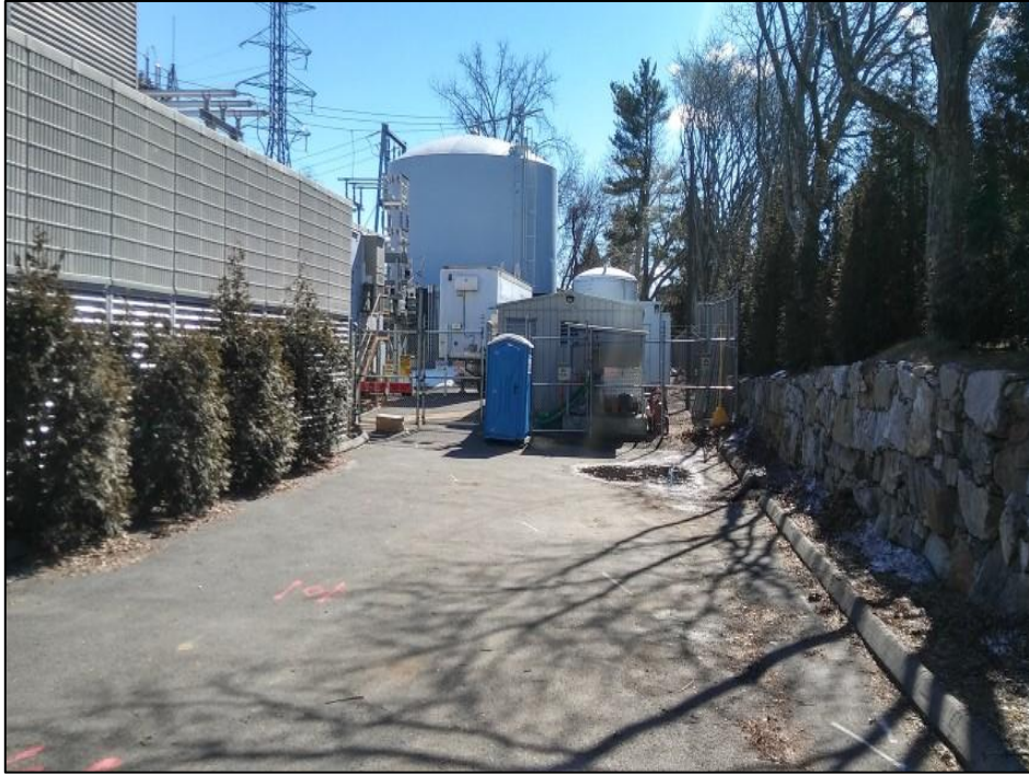
Photo 15. Overview photo of the termination point of the proposed underground transmission line at the existing Cos Cob Substation facing south.
