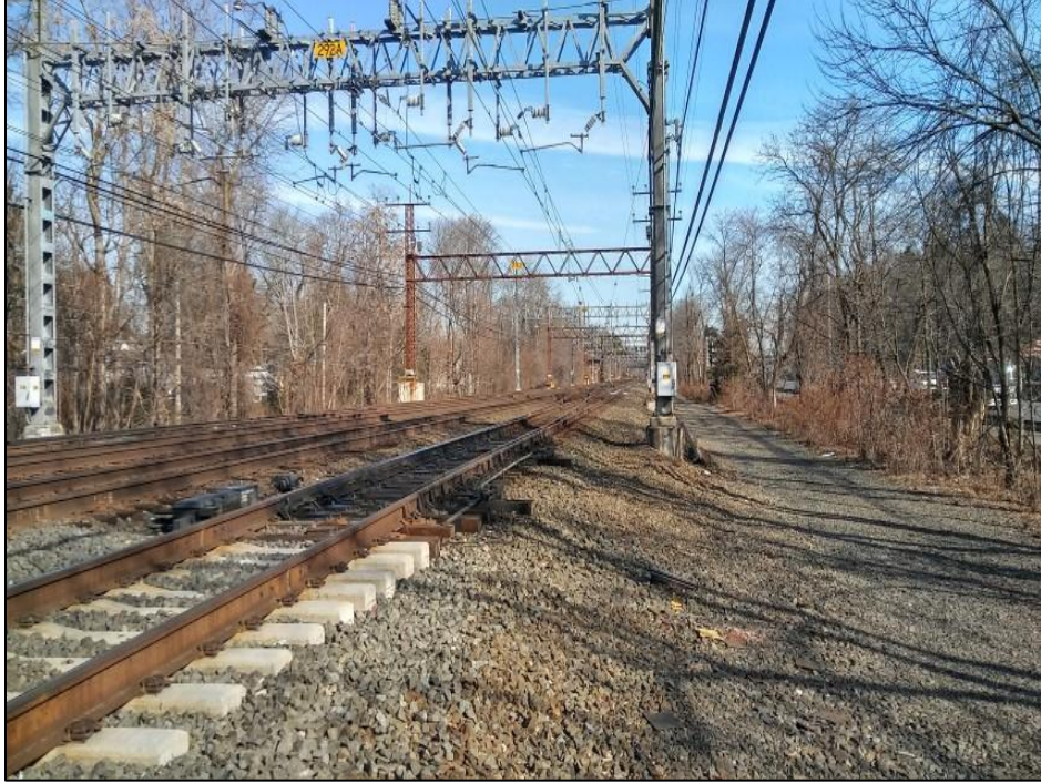
Photo 9. Overview photo of the central portion of the overhead transmission line facing east.
