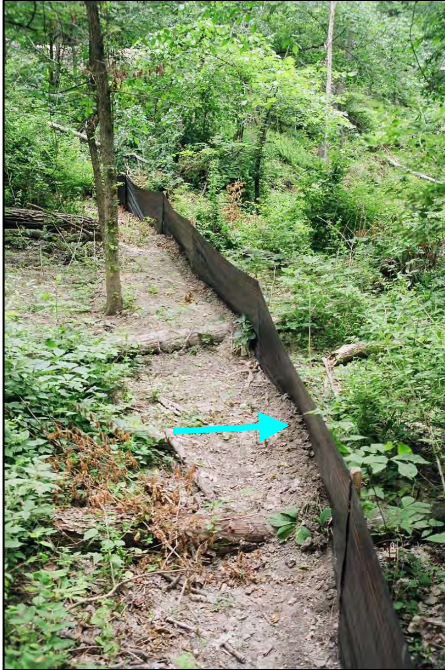
Properly installed and functioning silt fence. Direction of flow indicated by blue arrow.
