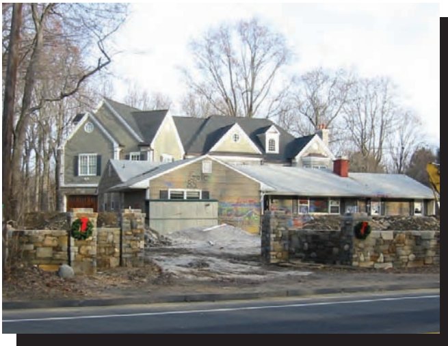
A 1950's era ranch house being replaced by the larger house behind it
