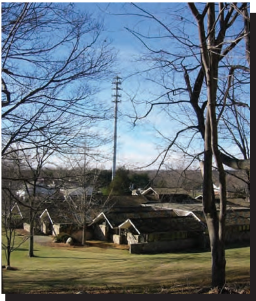
Cellular tower, Weston
