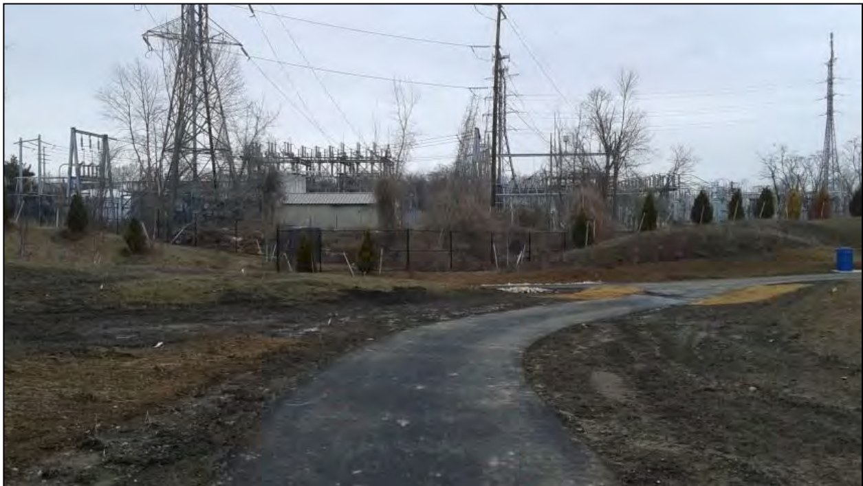
Photo 6. Overview photo of the Cos Cob Power Substation facing north (note this area once contained the Cos Cob Power Plant, a National Register of Historic Places property that has been demolished).
