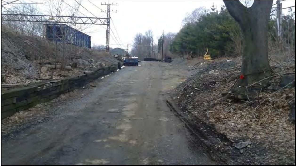
Photo 11. Overview photo of the project corridor along Station Road facing east (note construction in this area).
