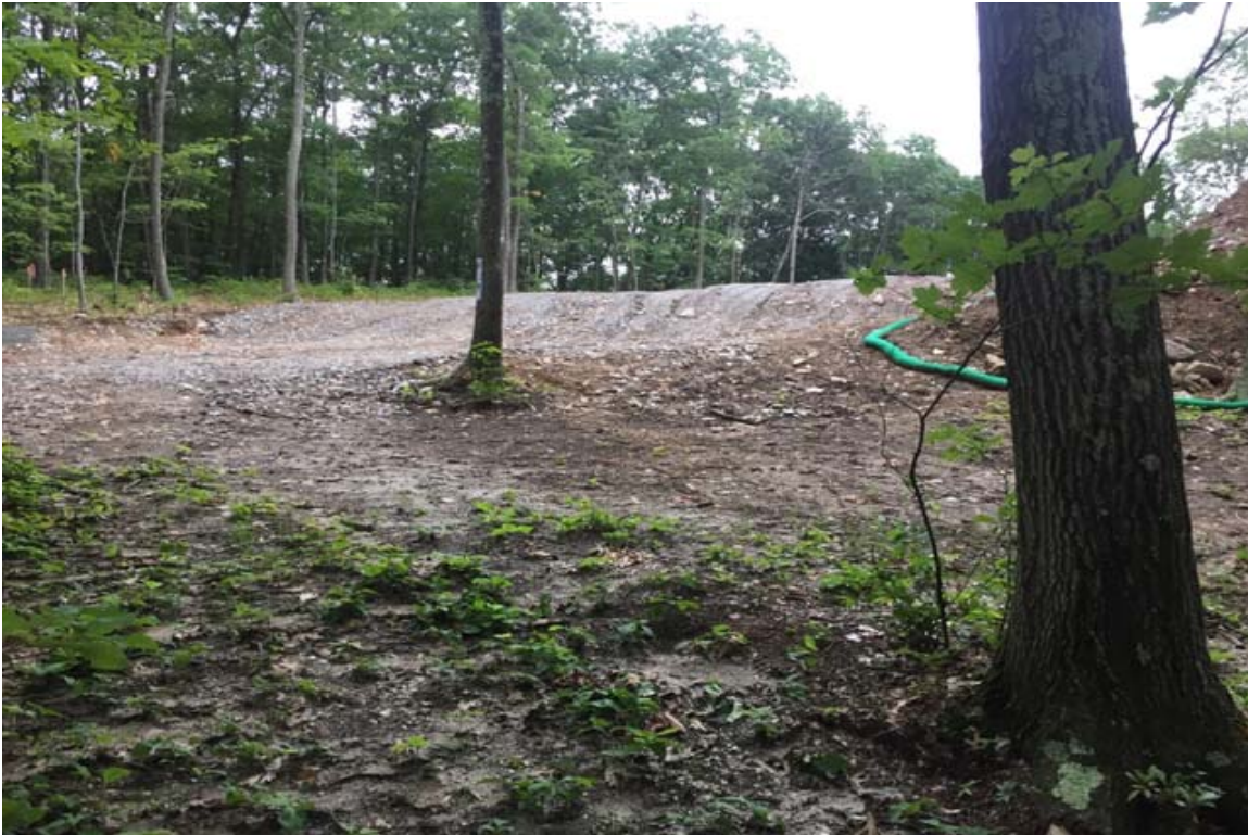
Photo 5: View of compost filter sock along portion of west side of compound. CA#3 implemented. Perimeter control needs to extend further to north to control rill erosion - CA#5.
