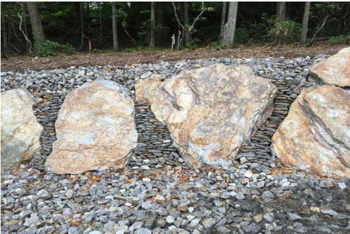
Photo 2: View of drainage swale and stone retaining wall on north side of access.
