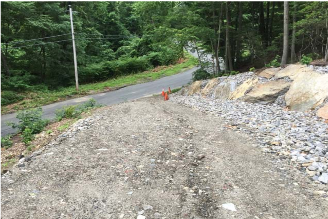
Photo 4: View of drainage swale along north side of access road preventing siltation onto Keegan Road. CA #2 implemented.
