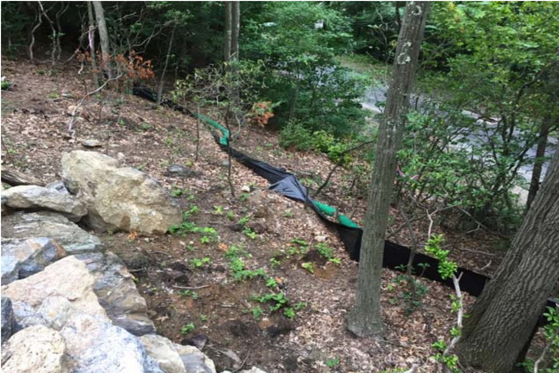
Photo 8: Repair silt fence along access road entrance perimeter control south end, looking southwest with Keegan Road in background.
