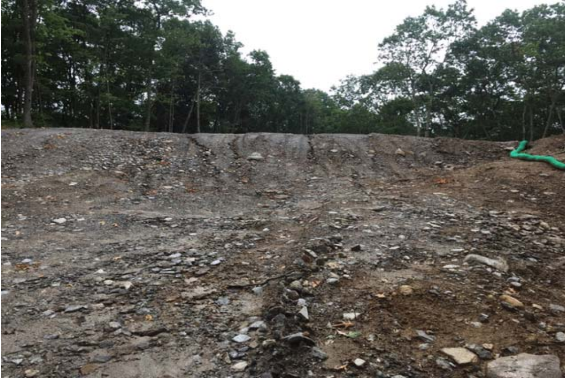
Photo 7: View of minor rill erosion along west side of compound, south of access road - add perimeter control – CA #5.
