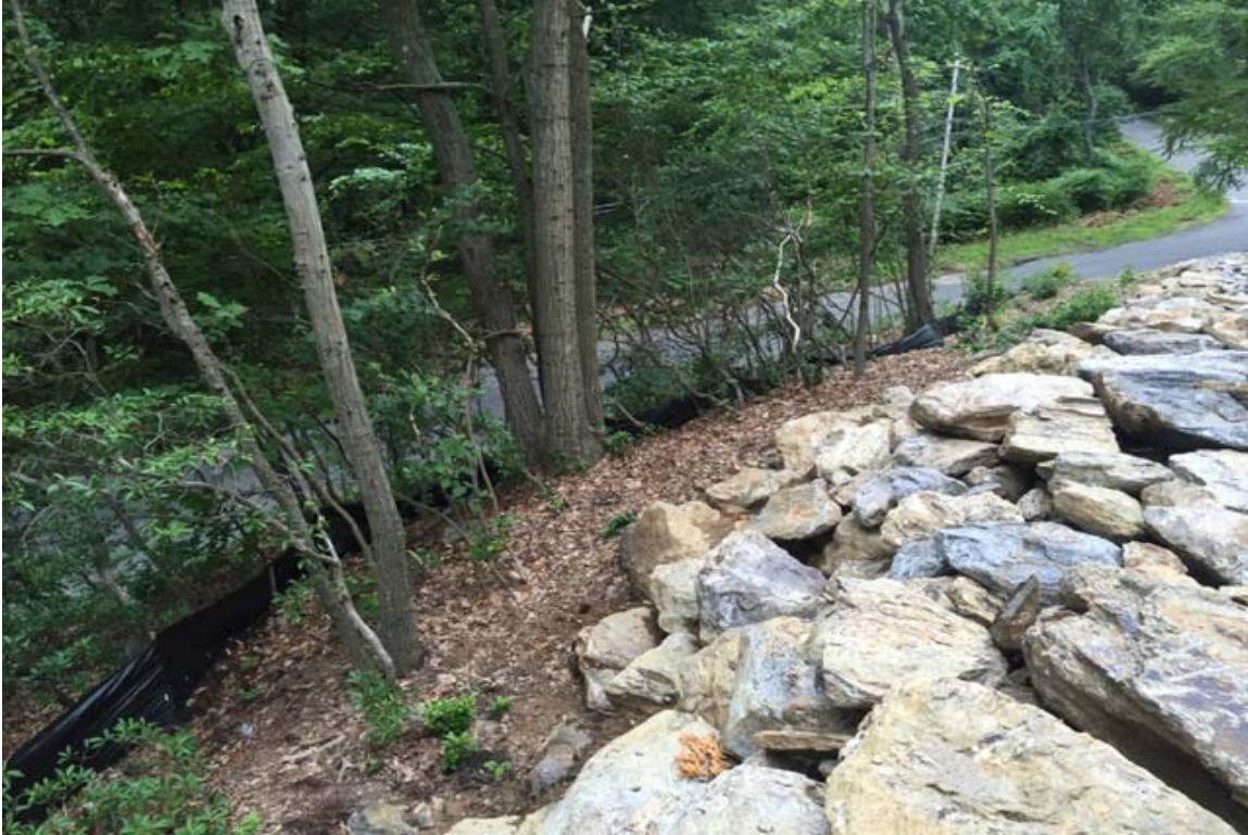
Photo 3: View of silt fence along west of access road entrance in good condition. CA #1 implemented.
