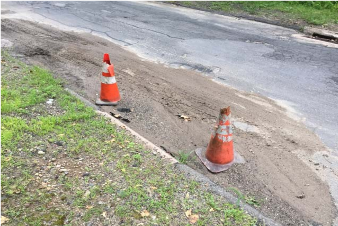
Photo 9: Clean out sediment clogged catch basin silt sock – CA #7.
