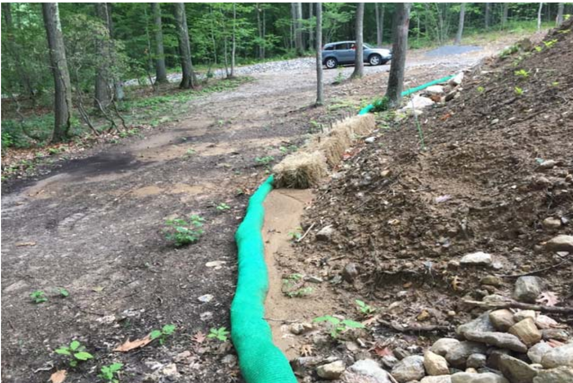
Photo 6: Clean out sediment buildup around west side soil stockpile and temporary seed stockpile looking north – CA #4.
