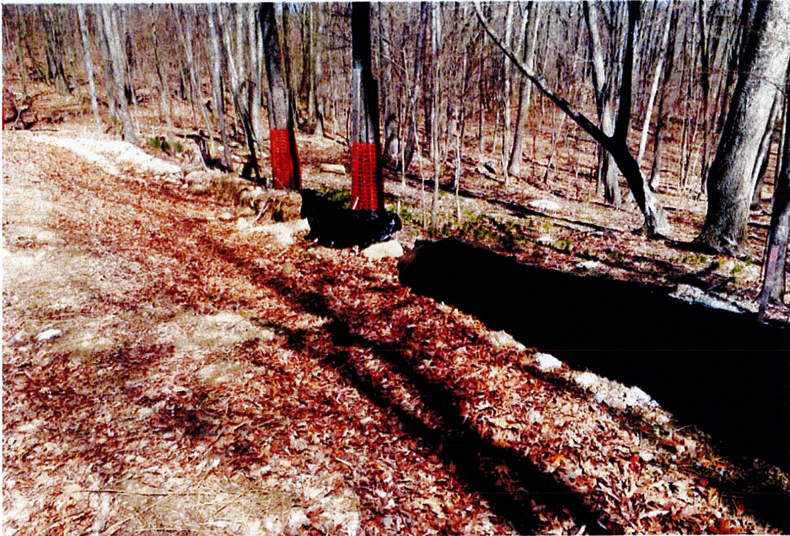
Photo 3: View of broken silt fencing looking north.
