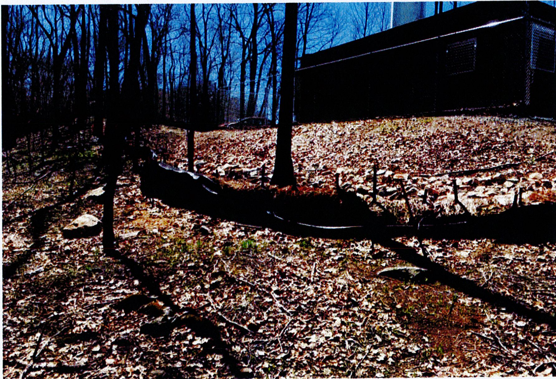
Photo 7: View of broken silt fencing looking southwest.
