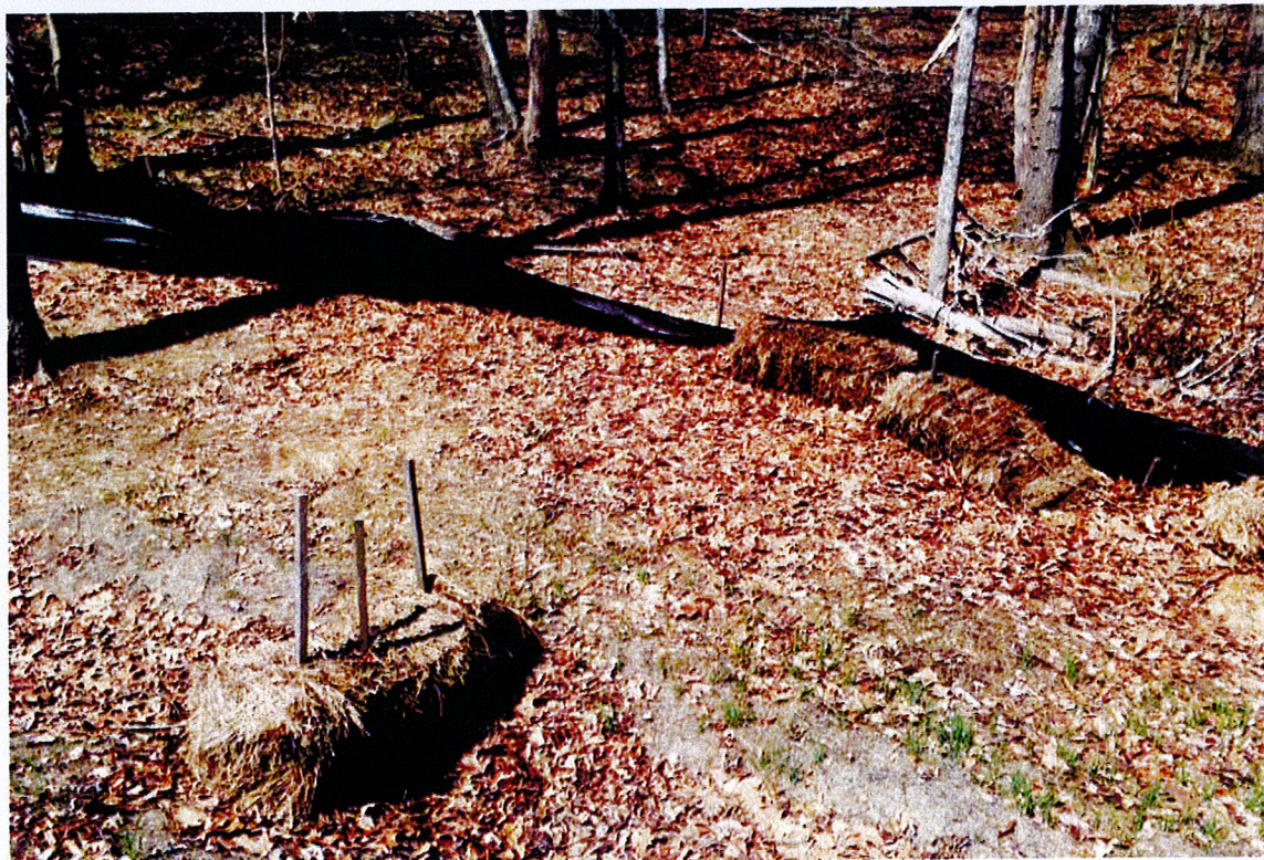
Photo 6: View of broken silt fencing looking north.
