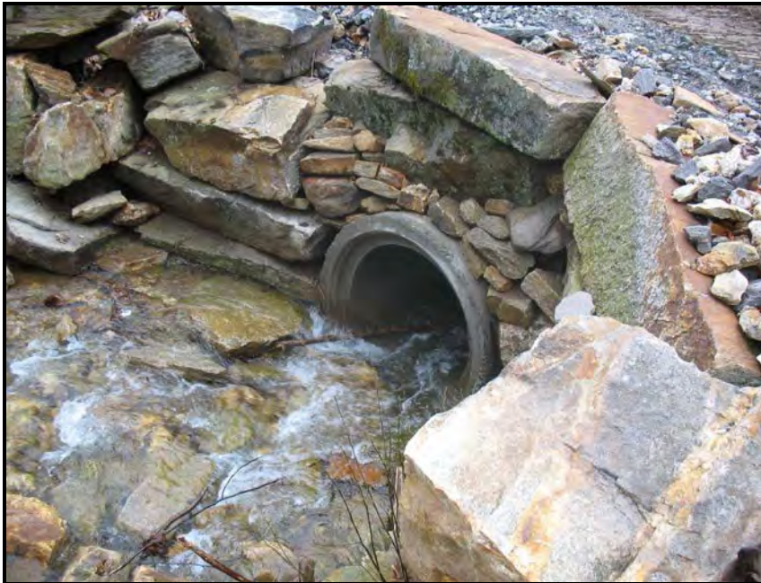
Culvert and riprap for stream crossing.
