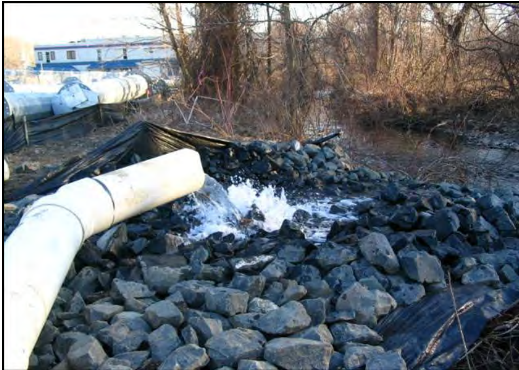
Riprap underlain by geotextile fabric
