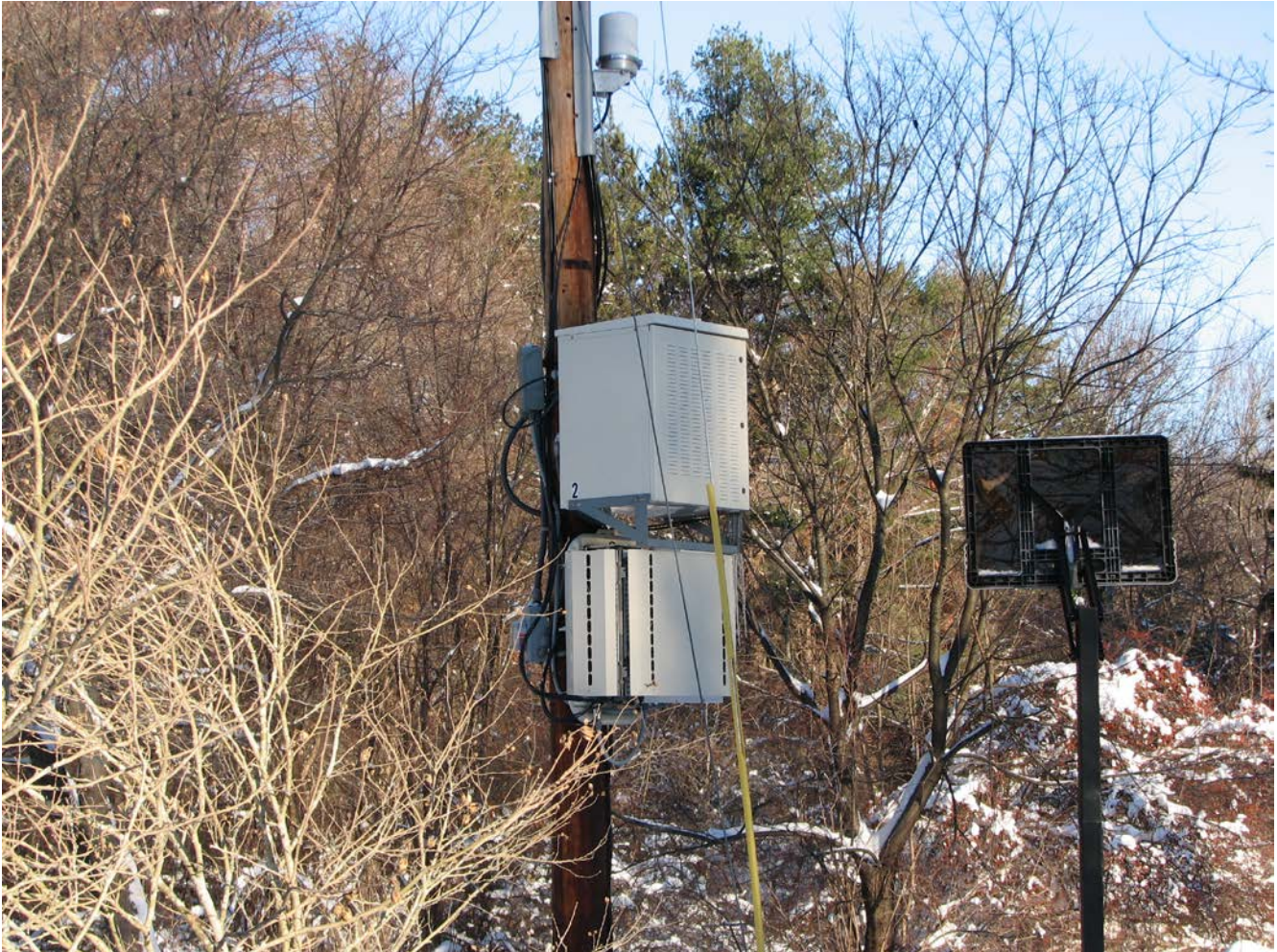
Figure 2: Typical DAS Node Equipment
