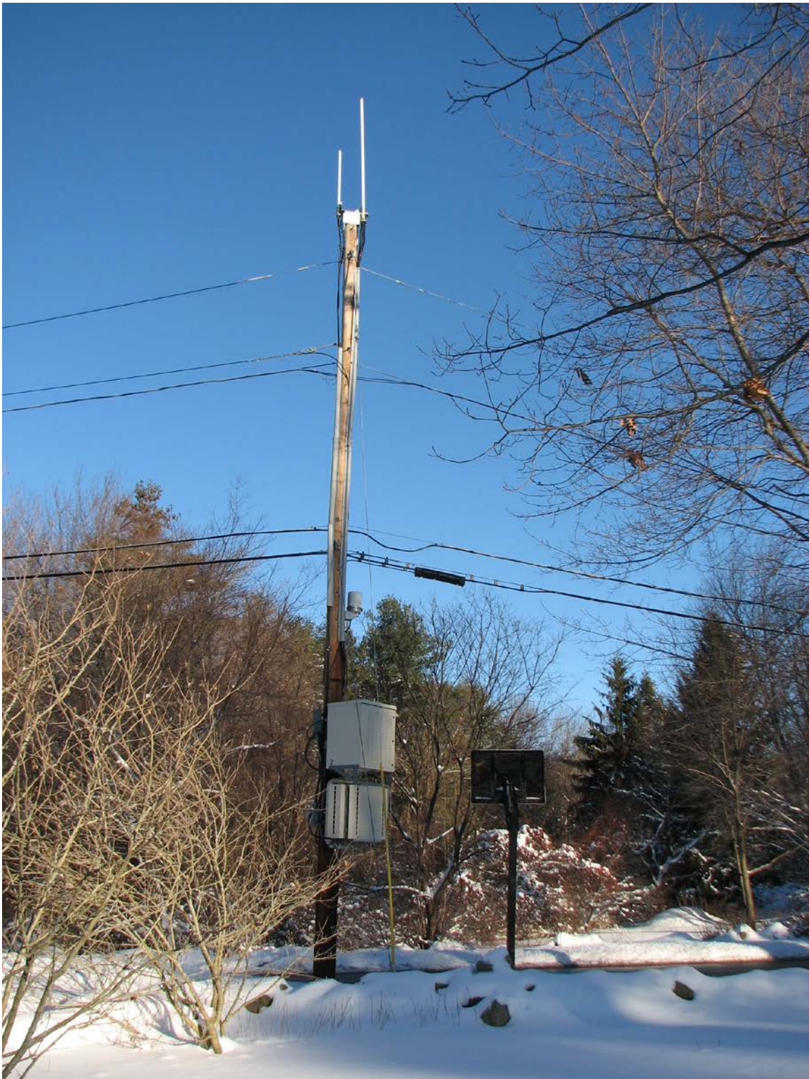
Figure 1: Typical DAS Node 1
