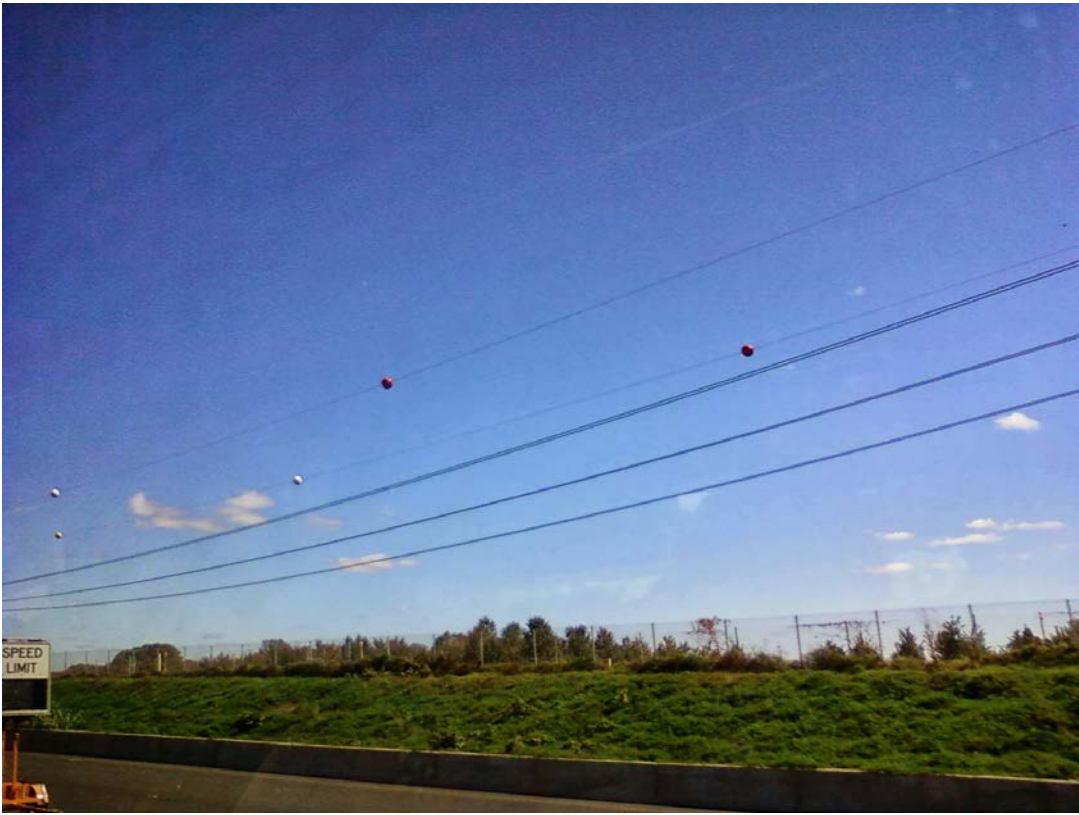
Figure 2 Representative Examples of Marker Balls on Transmission Lines
