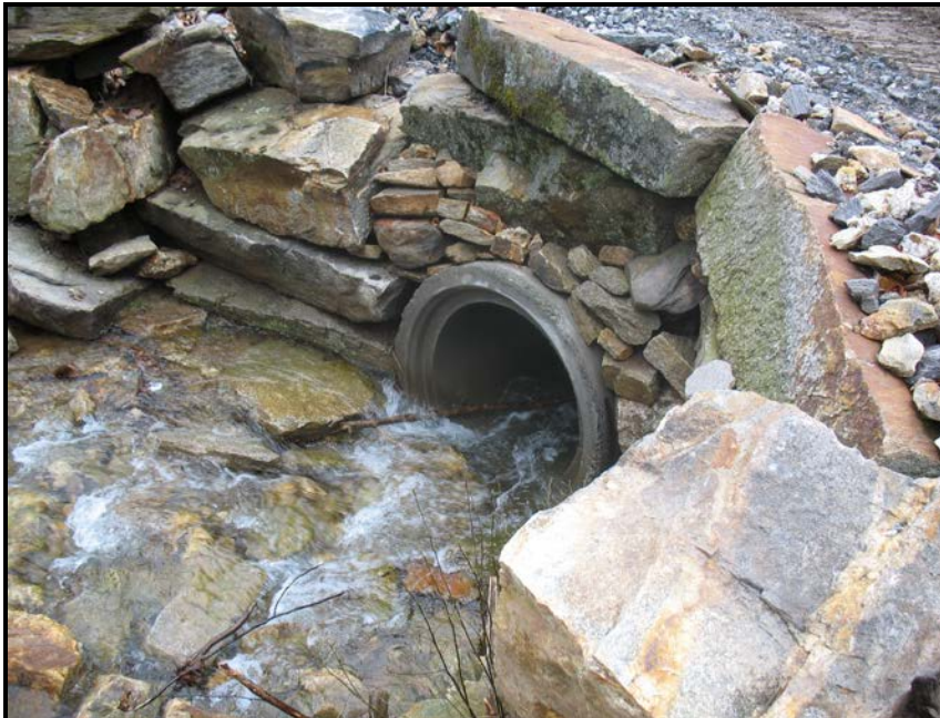
Culvert and riprap for stream crossing.
