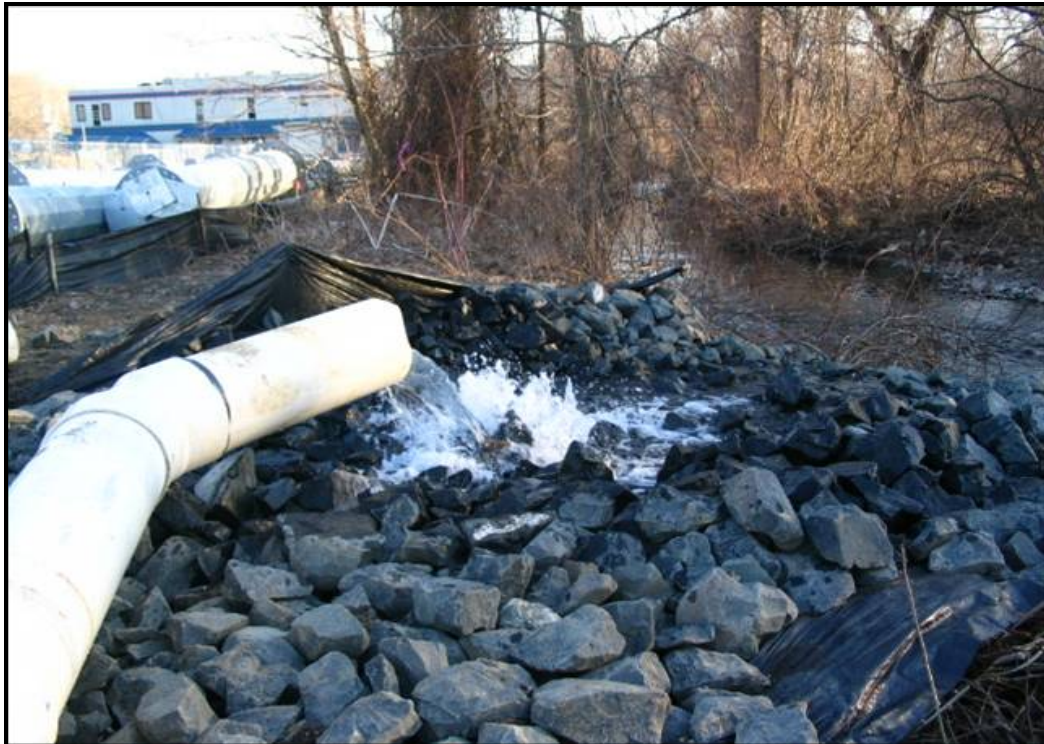
Riprap underlain by geotextile fabric
