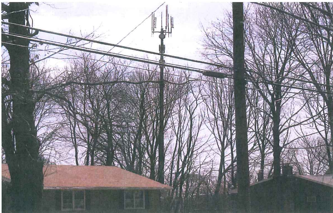
Figure 10: Photo-simulation of proposed tower at Killian Ave/Main Street intersection. Existing tower not discernable. Map location 13.
