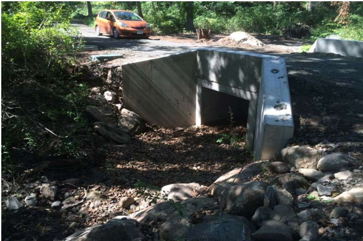
Photo 2: View of culvert outlet looking northwest, culvert set a proper elevation and backfilled with 1 foot of streambed material.
