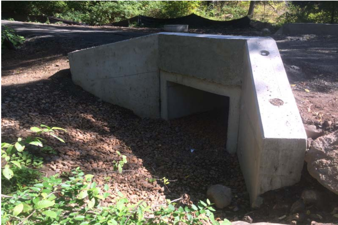
Photo 1: View of stream crossing new culvert inlet looking southeast, culvert set a proper elevation and backfilled with 1 foot of streambed material.
