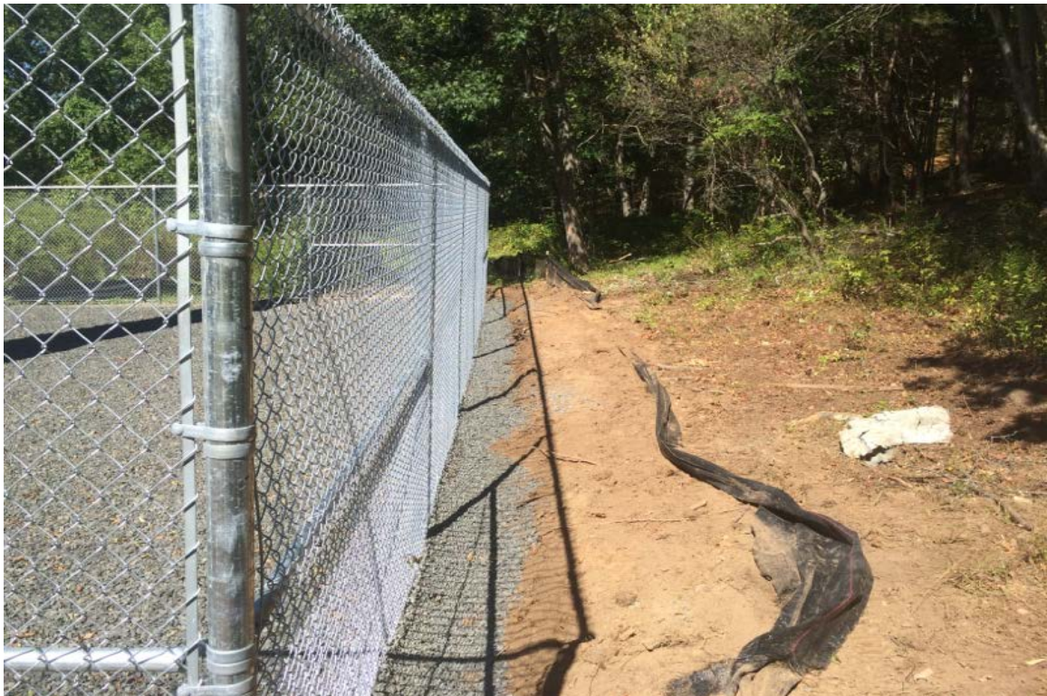
Photo 6: View of west side of compound looking north, silt fence needs to be reestablished around compound.
