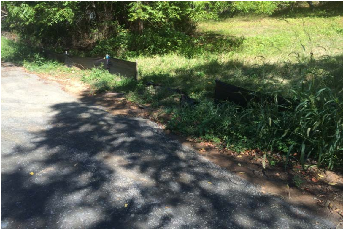
Photo 5: View of small break in silt fencing (typ.) that needs to be corrected, looking east.
