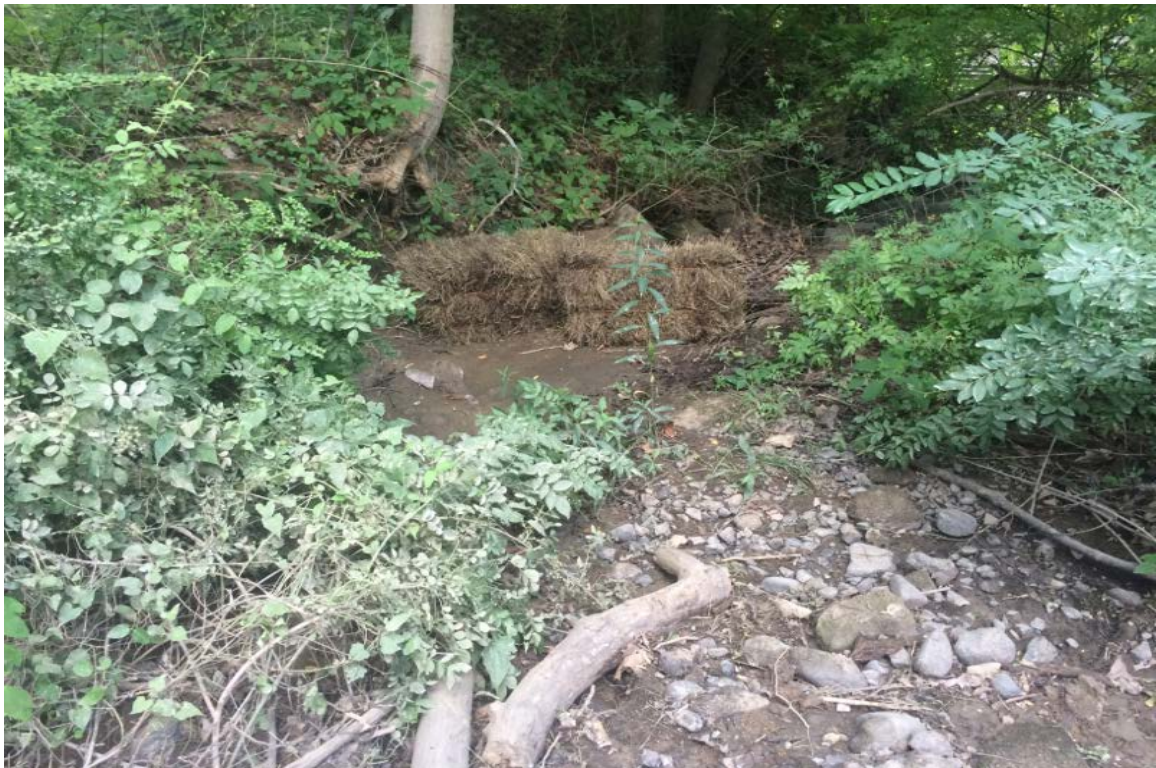
Photo 2: View of hay bale check dam in streambed south side (dry streambed, no flows) looking south.
