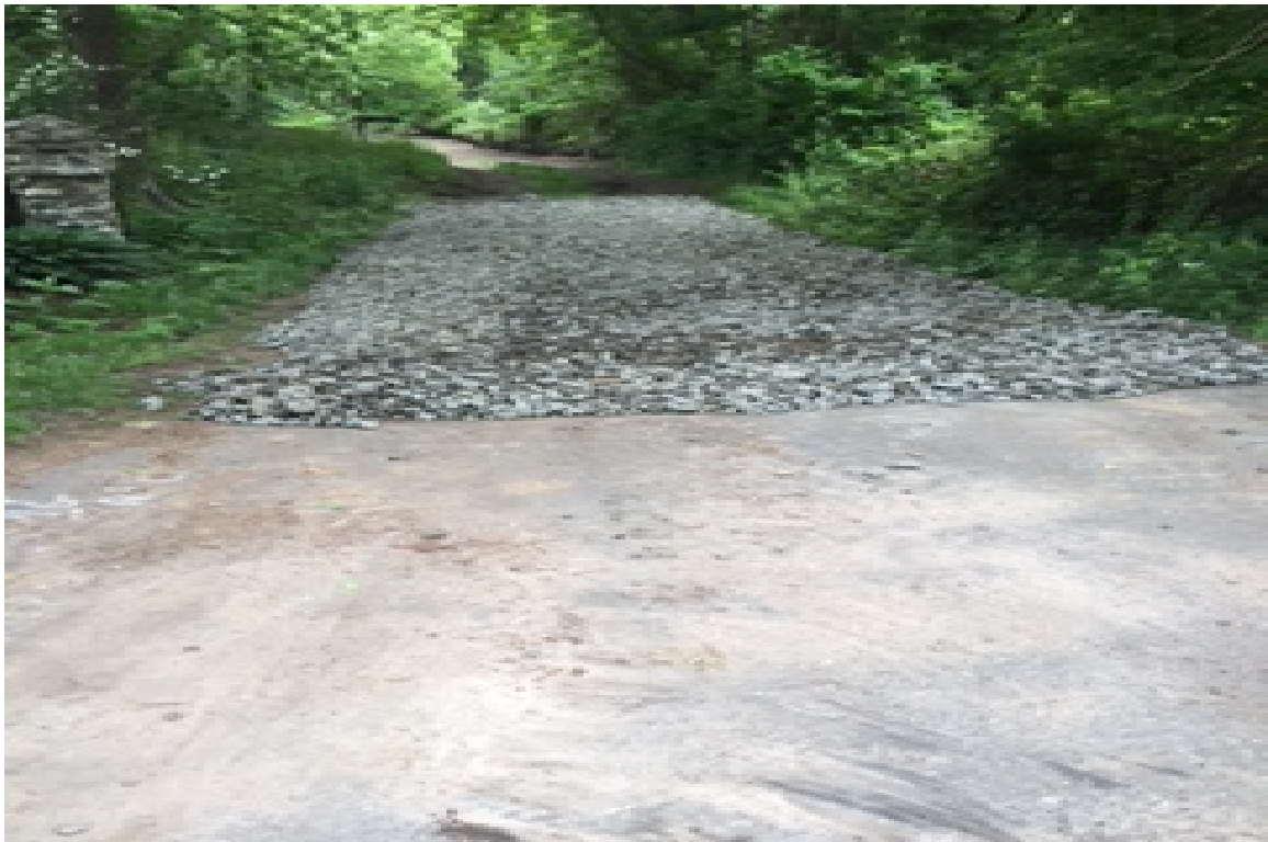
Photo 6: View of anti-tracking pad at construction entrance looking east from Moose Hill Road.
