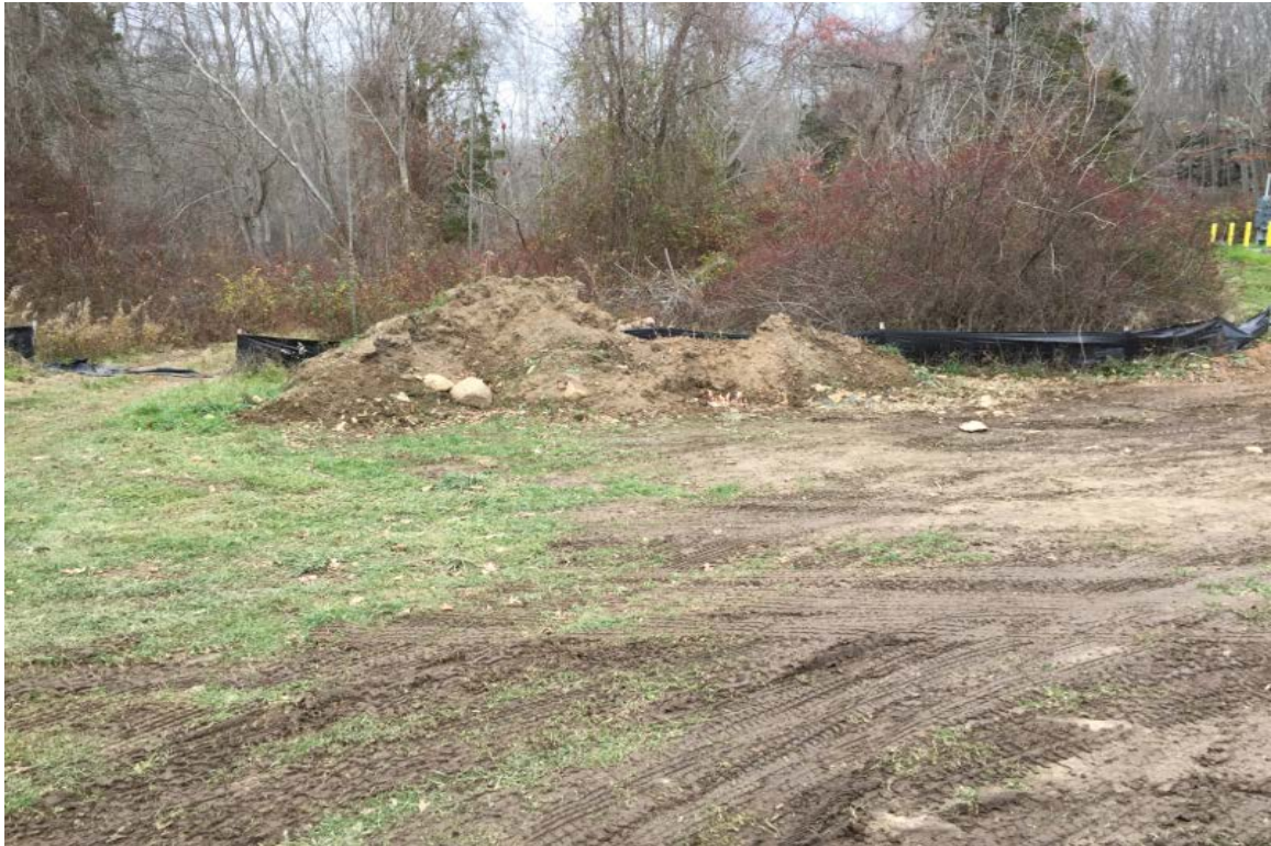
Photo 7: View of construction staging area and topsoil pile looking north. Area needs to be stabilized with seed and mulch.
