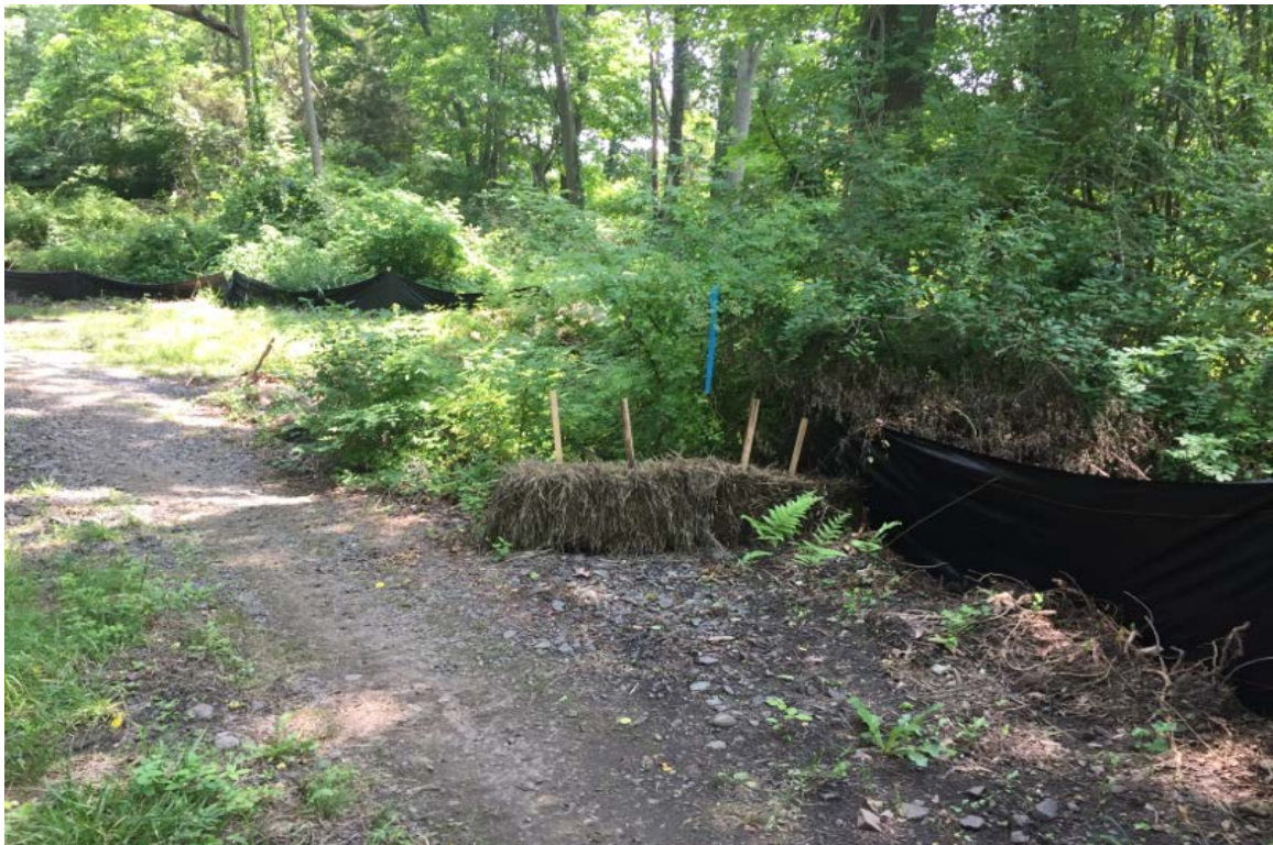
Photo 2: View of southwest side of culvert looking southeast at staked check dam.
