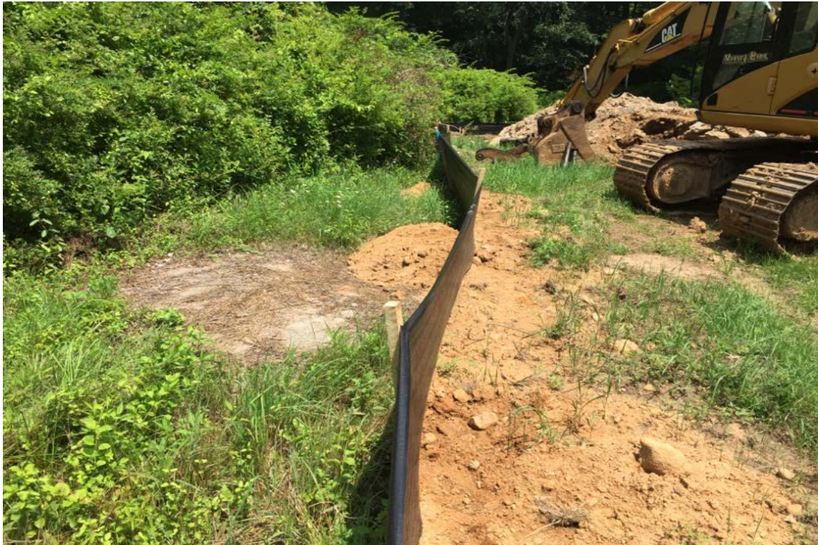
Photo 3: View of silt fence properly buried in exposed bedrock area looking northeast.
