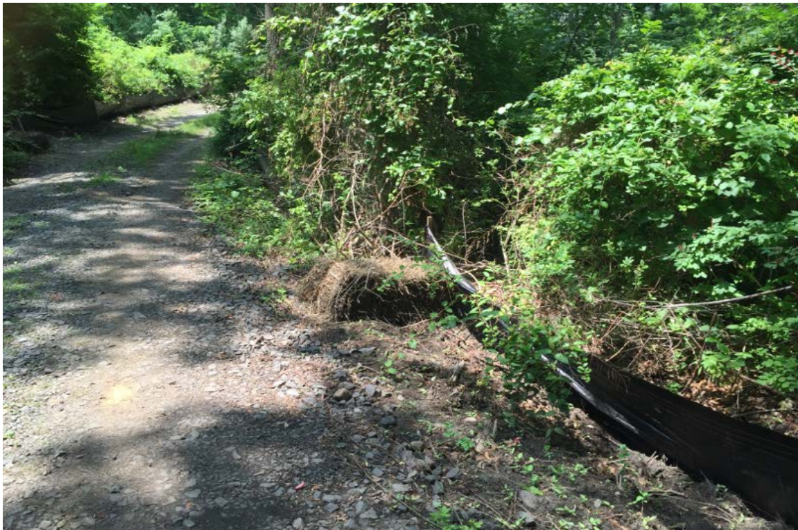
Photo 6: View of northeast side of culvert looking west correction area #2 stake bale needs to be staked down.
