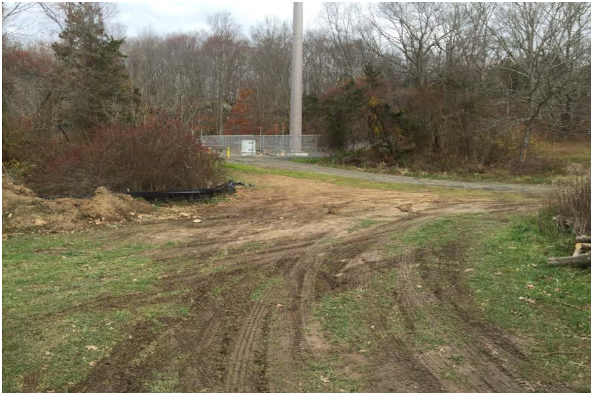
Photo 8: View of construction staging area and topsoil pile looking northeast. Area needs to be stabilized with seed and mulch.
