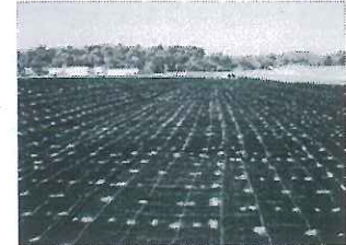
P550 was installed to provide long term erosion control protection for the Illinois DOT stormwater channel.
