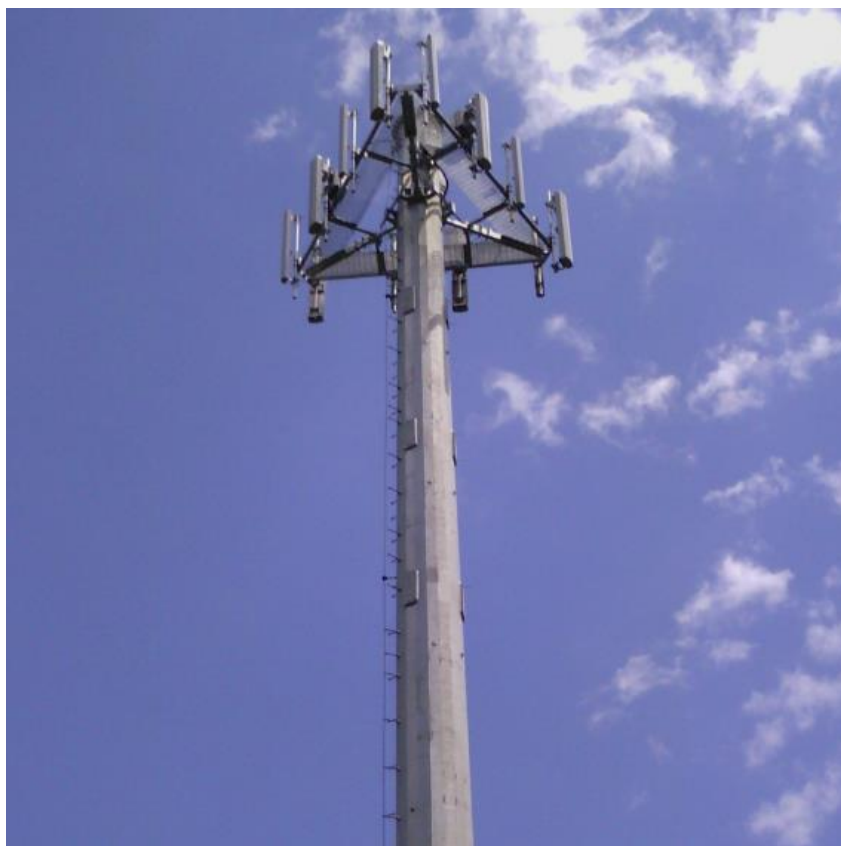
Cellco antenna array.
