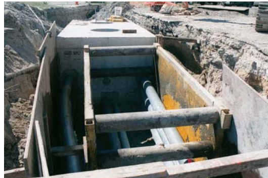
Ducts entering a single, pre-cast concrete splicing vault
