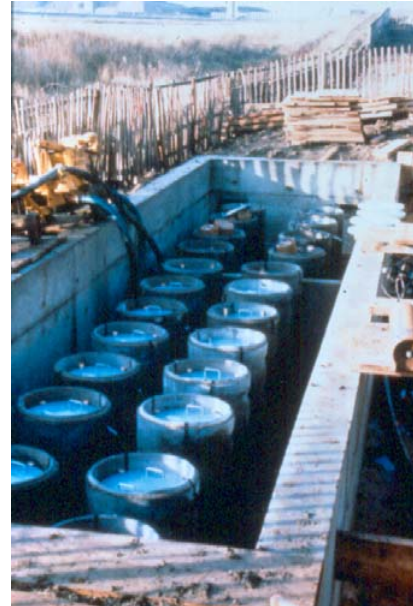
Pit housing fluid feed tanks
