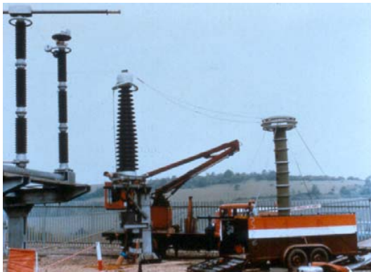
High voltage test set connected to SCFF terminal
