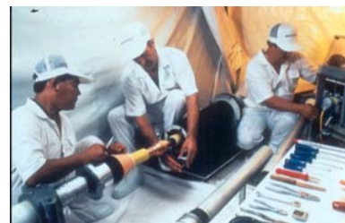
Connecting XLPE cables together in an ultra-clean environment within a buried joint bay
