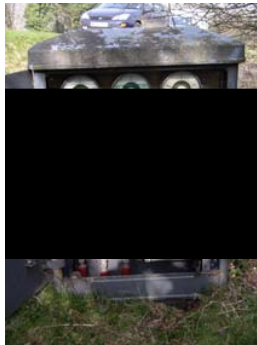
Kiosk containing pressure gauges and fluid leak alarms
