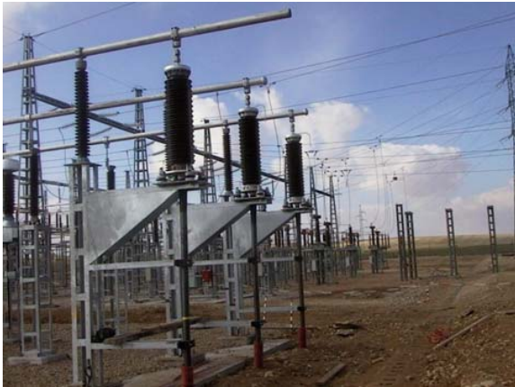
115kV cable system terminations
