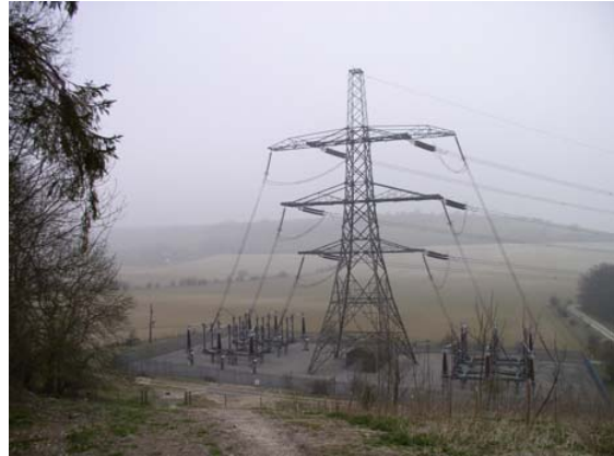
Transition stations are used to connect lines and cables together
