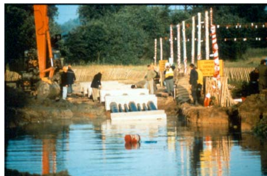
Installation of ducts to house the cables that will cross the river
