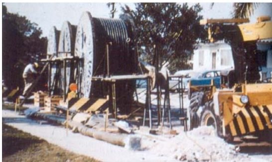
Three reels of cable are parked in the street ready to be pulled into a steel pipe
