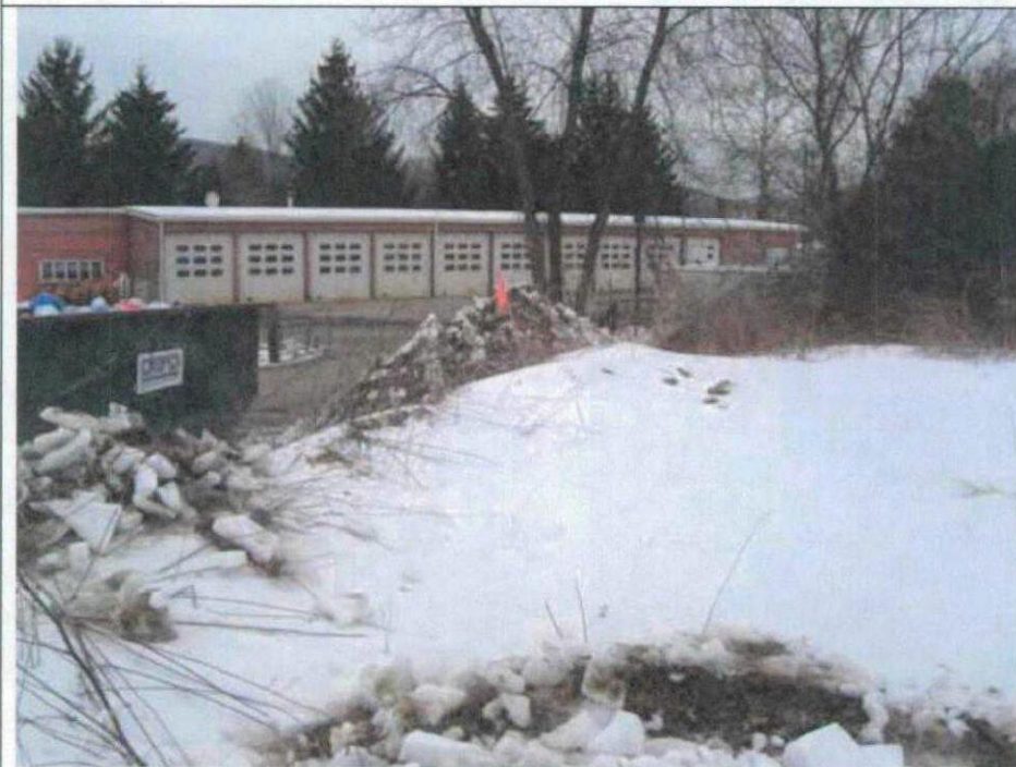
2. Proposed tower site, with the main garage in the background, facing north.
