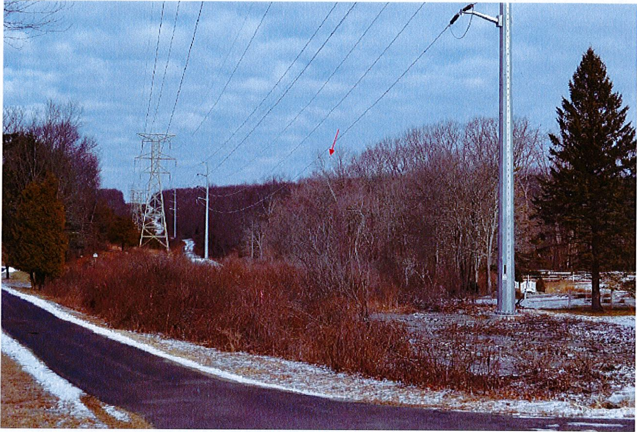
Photograph 4: Prokop Transmission ROW
