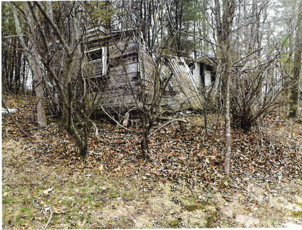
Photograph 25. Survey Area 4: collapsed summer house west of Lake Road. View to the north (Photographer S.A. Reeve, March 16, 2016).
