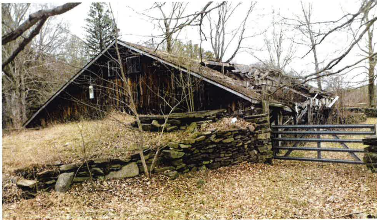
Photograph 5. Survey Area 2: barn east of Lake Road, fieldstone foundations and collapsing roof. View to the north (Photographer S.A. Reeve, March 16, 2016).
