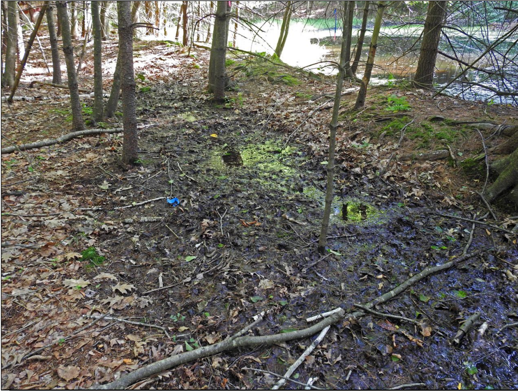
Photo 5: Active seepage area adjacent to man-made pond during a moderate drought; 7-21-16; facing southerly
