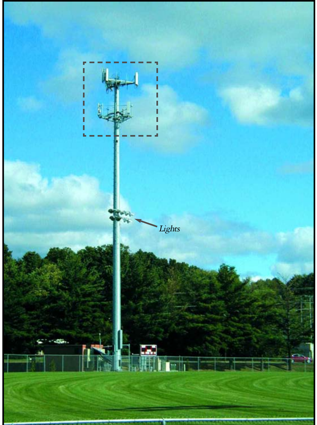
Park lights share a structure with wireless telecommunications antennas at Chelsey Park in New Britain, CT. Photograph taken in September of 2006.
