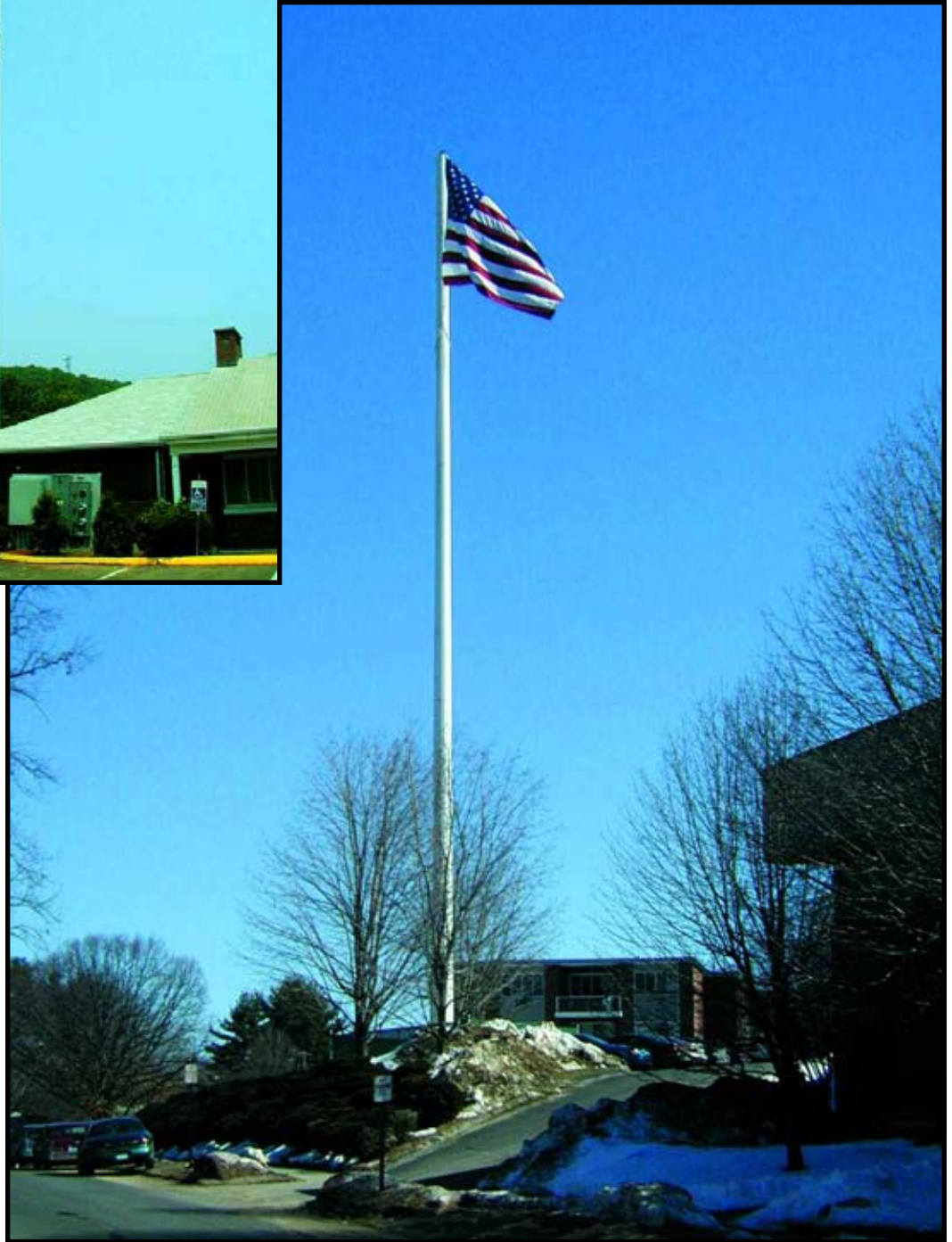
985 Farmington Avenue in Bristol, CT. Antennas are located within the flagpole structure and equipment is at the base of the structure.
