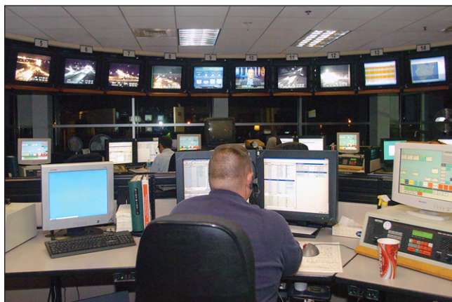
Figure 3.1—The Pennsylvania Turnpike Commission traffic control center.
