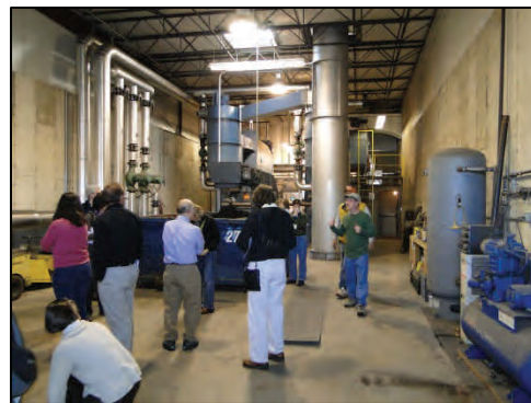
Figure 6. Joe Geremia and Phil Banning discuss the biomass boilers at Geremia Greenhouse.
