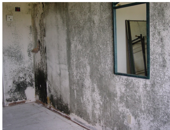
Fig 1. Moldy hotel room after the building roof and envelop were damaged by a hurricane.
