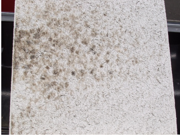
Fig 3. Moldy ceiling tile caused by high humidity.
