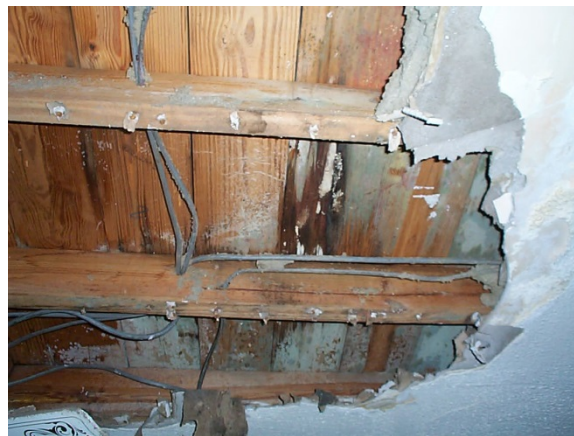
Fig 2. Hidden Molds due to a water leak.
