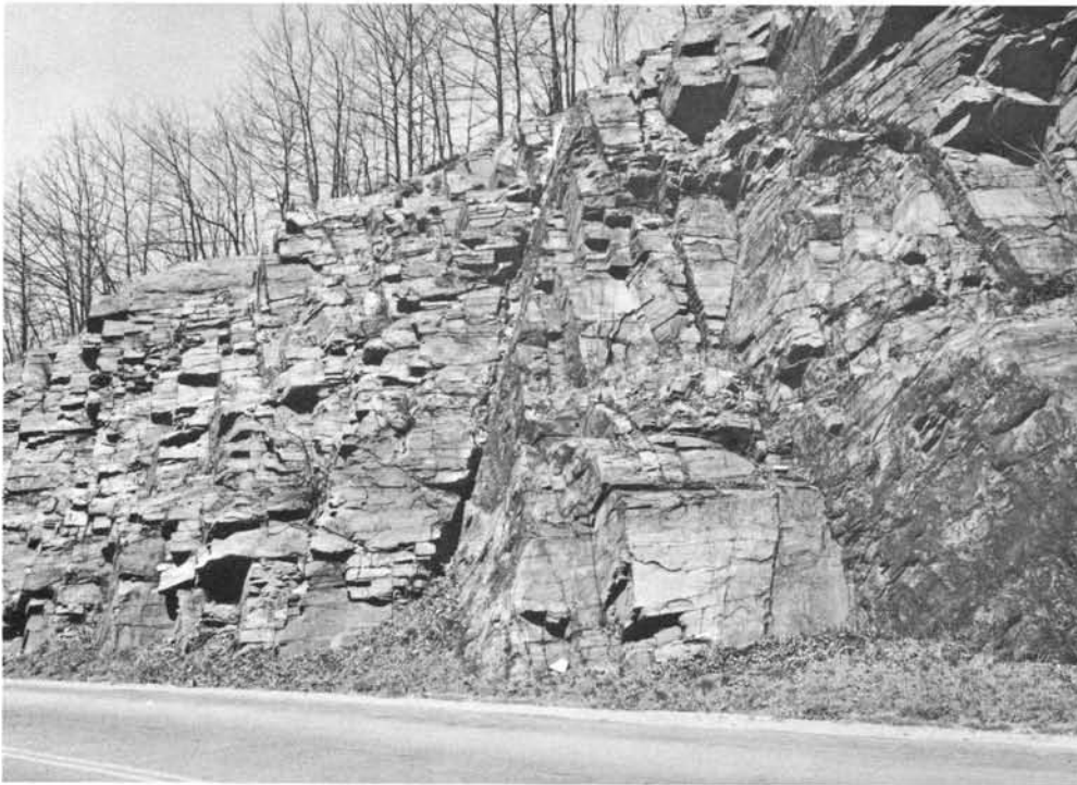
Figure 2. Bedrock outcrops along highway cuts exhibit many fractures. The gently sloping fractures are along bedding and foliation planes. The steeply sloping fractures are along joints. The prominent steeply sloping fracture in the center of the picture is a fault. All of these fractures may extend to considerable depth and serve as pathways of water movement. (Photo - U.S. Geological Survey)
