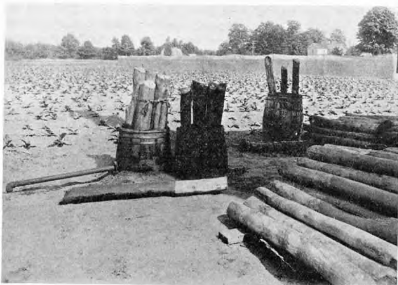
FIGURE 68. Simple equipment for treating poles by the open tank method. Creosote in barrel on left is heated to 220° F. by charcoal fire in pit under end of 2 inch pipe return coil. Cold creosote bath in second barrel. Third barrel is for draining excess creosote. Tops of poles cut off in this experiment.
