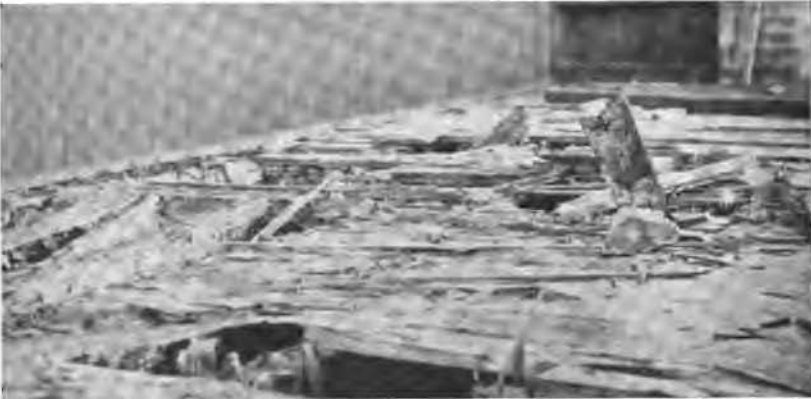
b. Rotten Condition of Living Room Floor.
