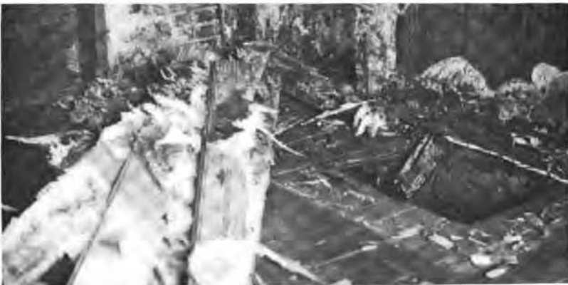
c. Luxuriant Growth of Fungus on Underside of Boards, etc.
